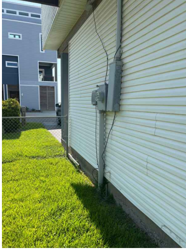
Main Service Panel Manufacturer: General Electric
