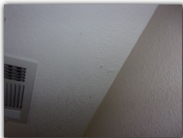
Nail pops noted in various areas.
