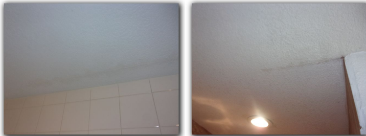
Common hairline wall cracks were noted in the
