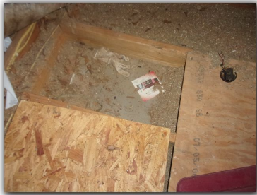
Missing insulation noted in various areas.
