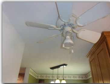
Missing globes noted.
