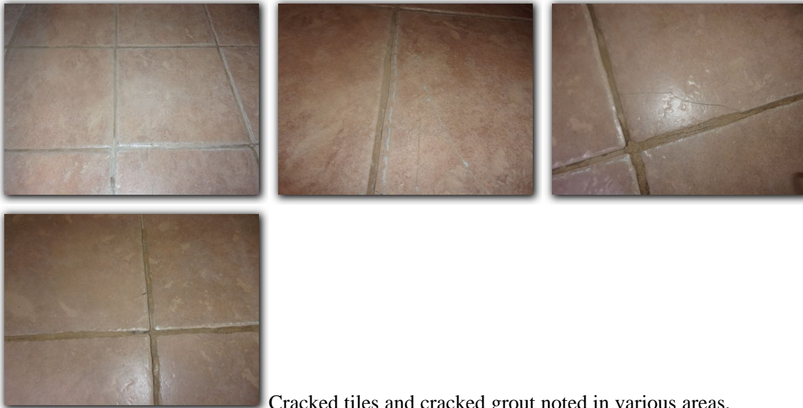
Cracked tiles and cracked grout noted in various areas.
