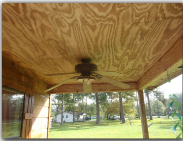
Warped fan blades noted.
