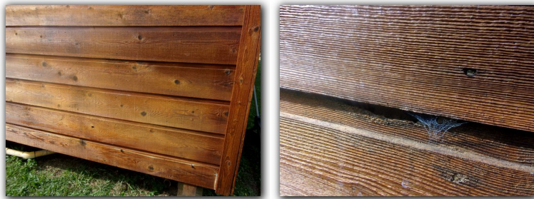
Moisture damage and openings noted on the east end
