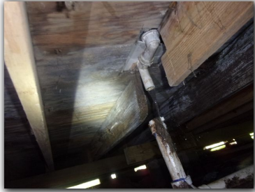
Floor joist noted under the hall tub that was improperly notched.
