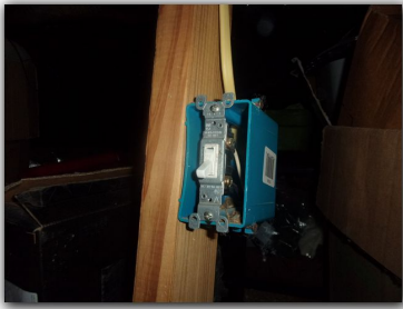
Missing cover plate noted.
