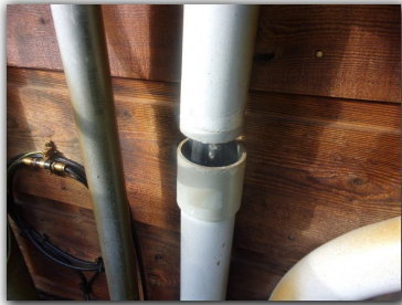
Loose conduit noted.
