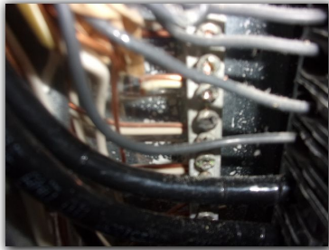
Ground and neutral wires should be separated in the sub panel area.
