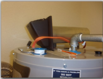
Wiring exposed on interior finishes is recommended to be relocated or protected by a rigid conduit.
