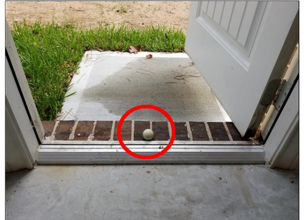
The brick sill did not slope away from the home
