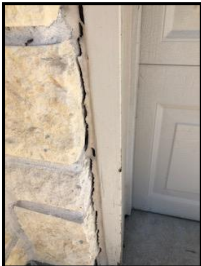
Trim separating from brick
