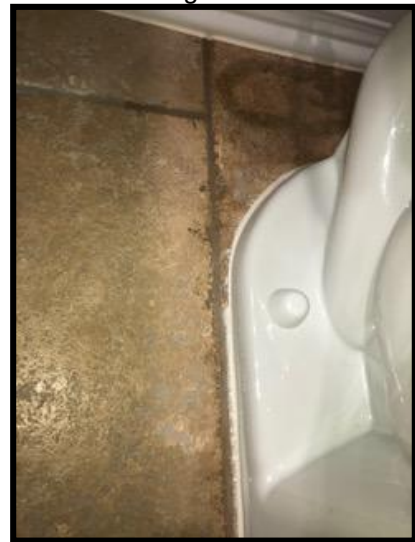
Leak at commode
