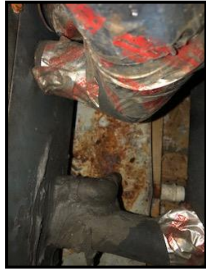
Corrosion in AC pan
