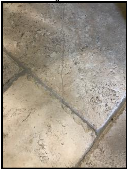
Cracked floor tiles
