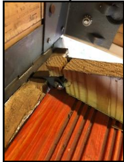
Cracked attic ladder
