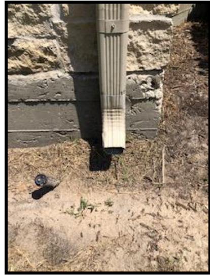
Missing splash blocks
