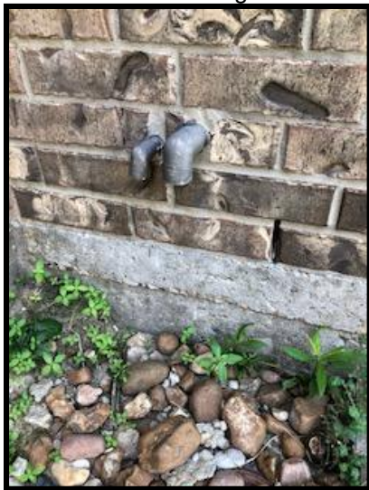
Drain too high
