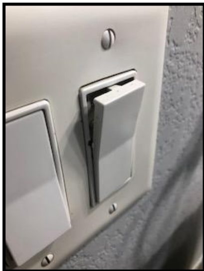
Voids at light switches
