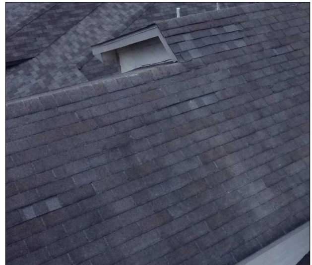
Evidence of previous repair. Multiple shingles present. Poorly attached and overlapped.
