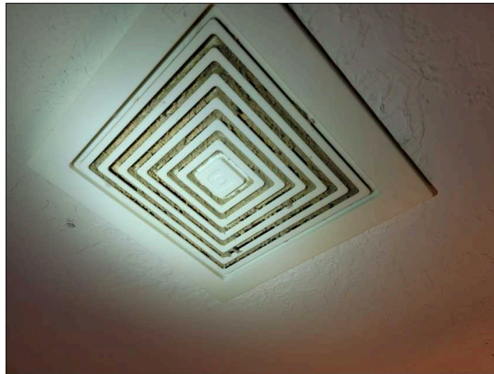
Exhaust vents are dirty. Recommend having cleaned out.
