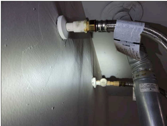
Type of Supply Piping Material:CPVC
