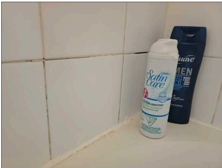
Holes / Cracks in grout around showers / baths. These could allow water to exit the shower enclosure.
