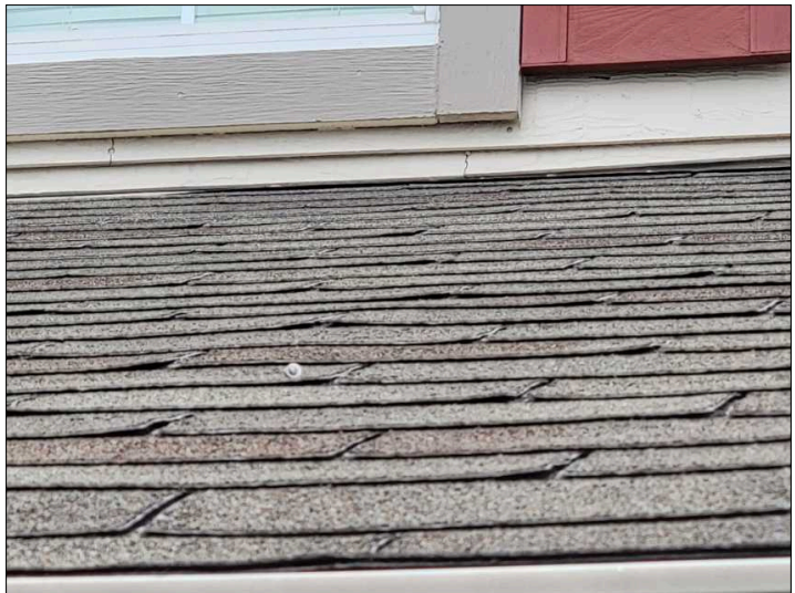
Lifted shingles noted. These are subject to wind drive rain and water entering house.
