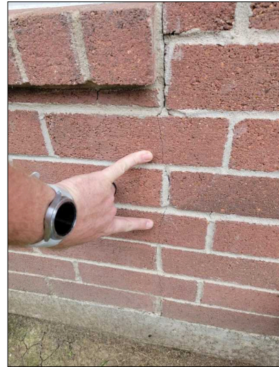
Exterior cracks in brick veneer noted. Cracks located at window corners are from settlement or uneven weight distribution.
