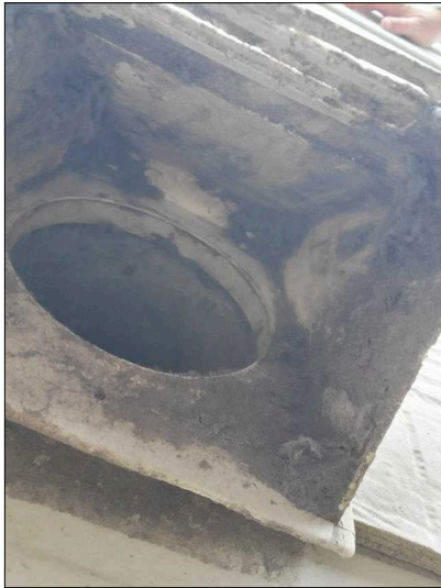
Suggest cleaning vent.
