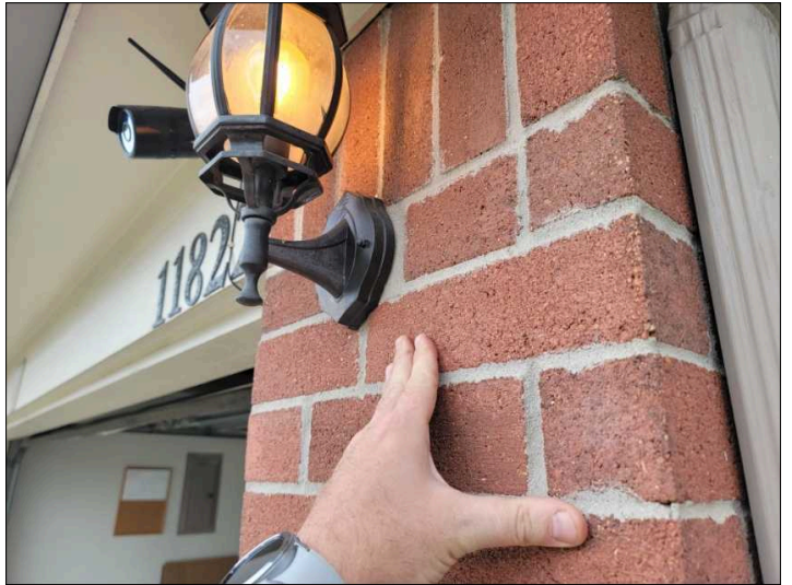
Exterior light fixtures should be weatherproofed.
