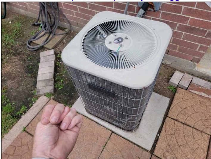
Condenser unit makes a rattle and is likely going to need replacement in the near future.
