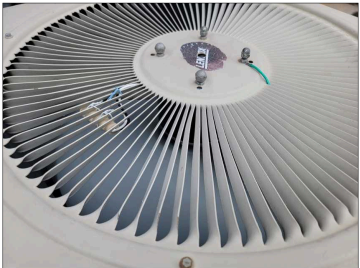
Repairs noted at condenser fan.
