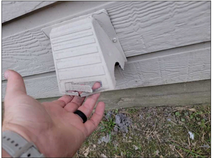
Damaged exterior cover
