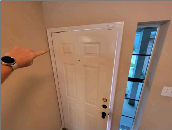
Loose hinge noted.
