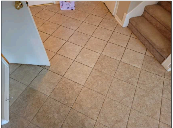
Noted that tiles in foyer are different, indicating they have been changed.
