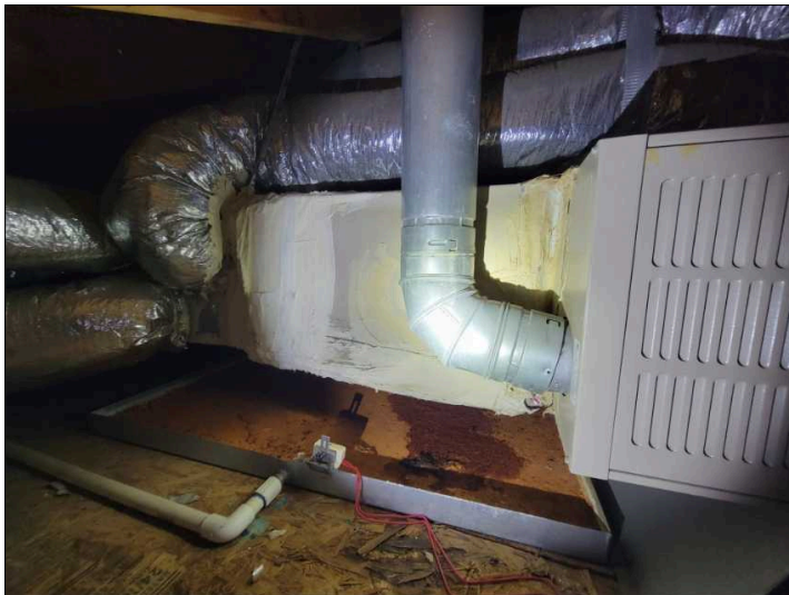
Heavy rust in overflow pan. Recommend replacement of overflow pan, as rust can cause holes to leak.
