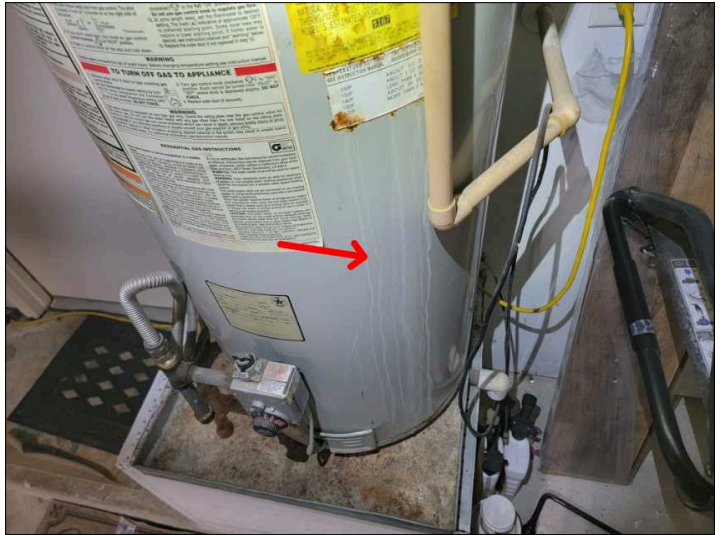
Evidence of leaking down side of tank.
