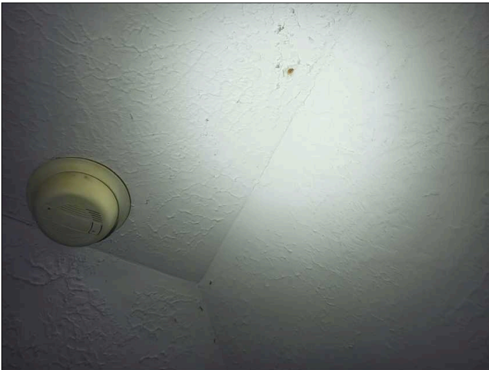
Nail pops noted.
