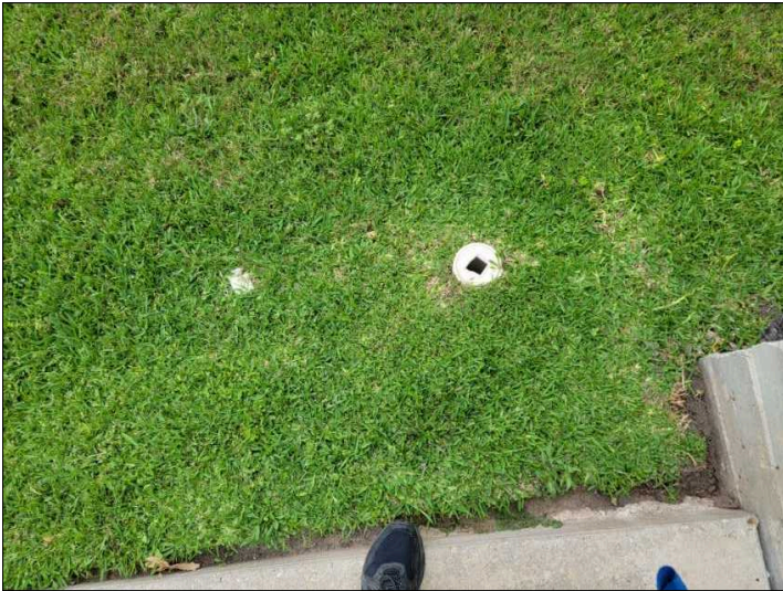
Sewer Cleanout cap is damaged
