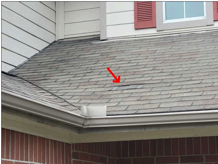
Evidence of previous repair. Multiple shingles present. Poorly attached and overlapped.
