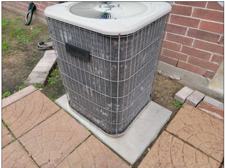
Damaged condenser fins.
