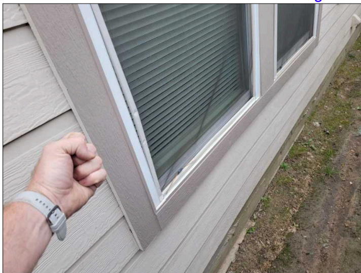
Missing / damaged screens noted.
