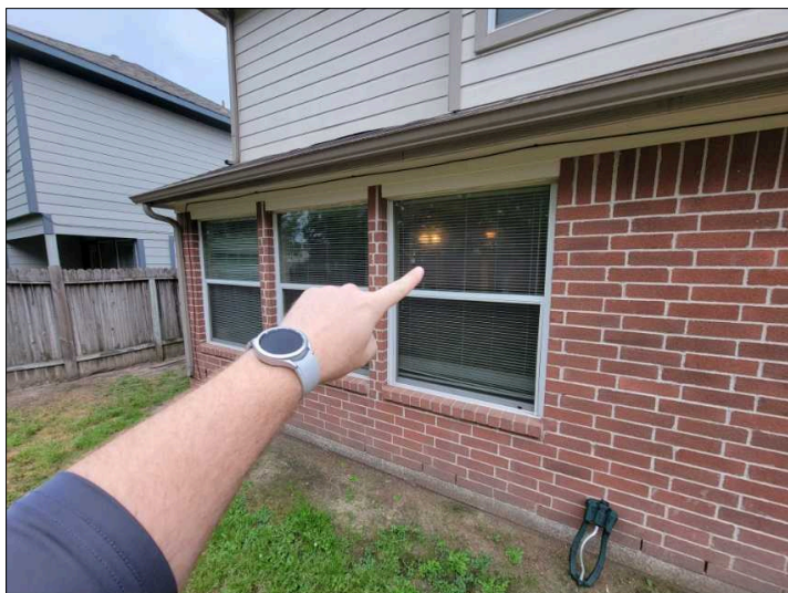
Condensation / fog present inside double pane windows. This is a sign that the gas between panes is gone, and the windows are less energy efficient and can be difficult to see through.
