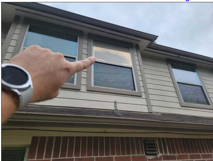
Condensation / fog present inside double pane windows. This is a sign that the gas between panes is gone, and the windows are less energy efficient and can be difficult to see through.
