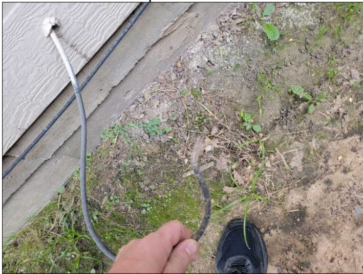
2nd Ground rod is disconnected from the grounding conductor. This should be repaired.
