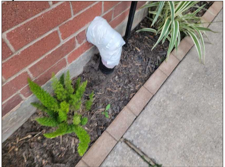
Water shutoff location.
