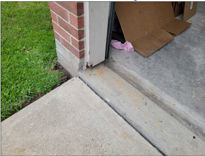
Wood rot at base of garage door trim
