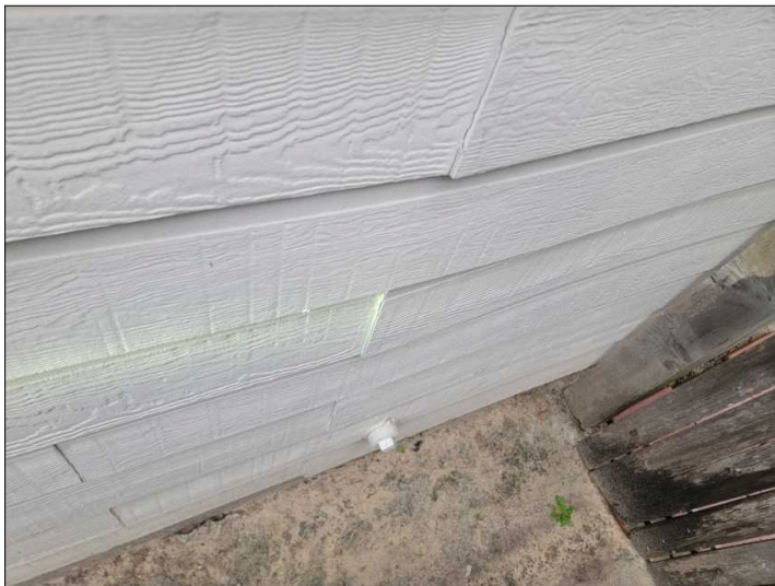
Siding is bulged at seams and sealed over.
