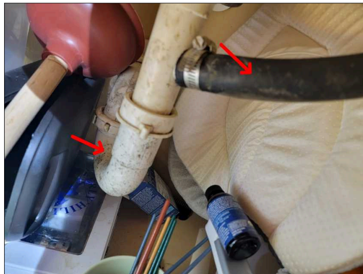
Surface mold present on drain lines under lavatory.
