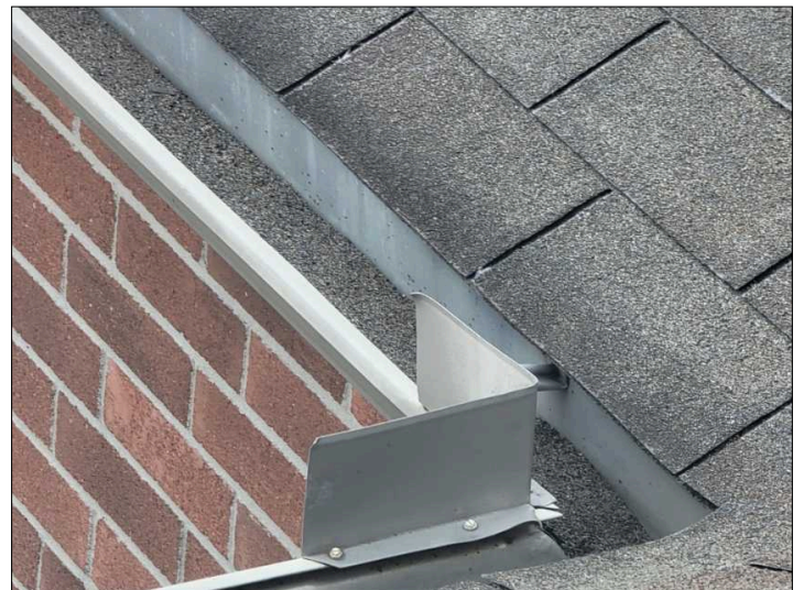
Gutters full of shingle granular. Shingles are past their life.
