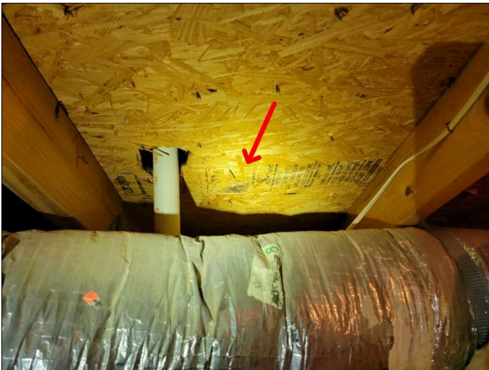
Evidence of past or present leaks, wet at time of the inspection. Monitor for leaks &/or have roofing contractor evaluate.
