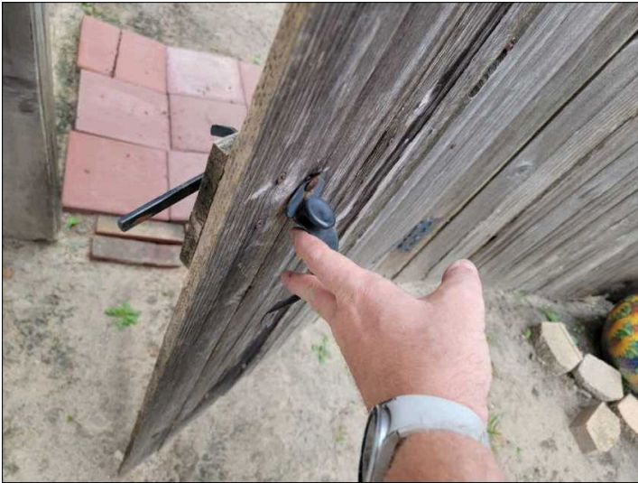
Gate latch is damaged.
