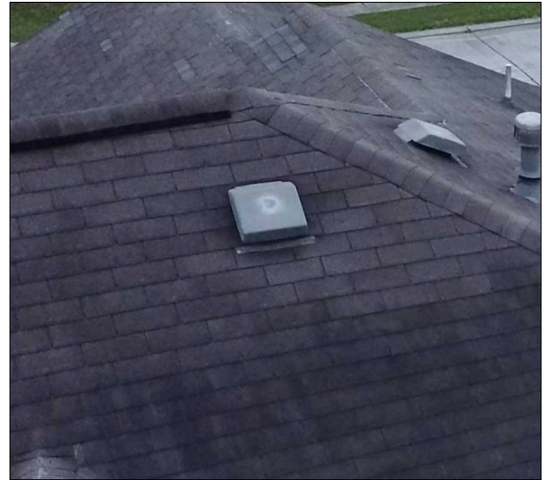
Evidence of previous repair. Multiple shingles present. Poorly attached and overlapped.
