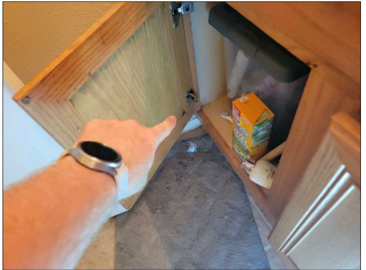
Cabinet hinge missing
