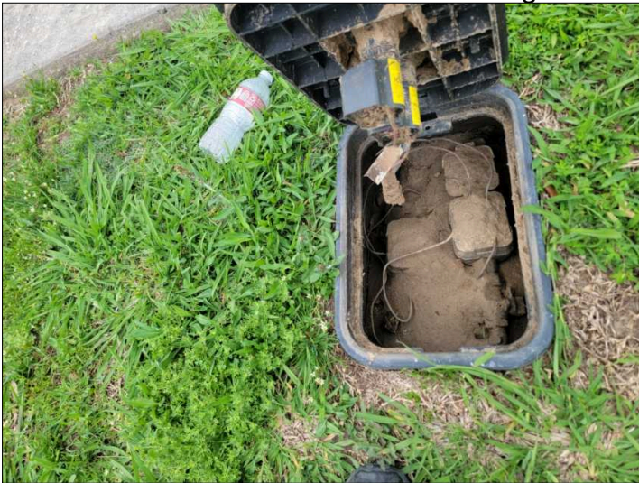
Meter box full of mud
