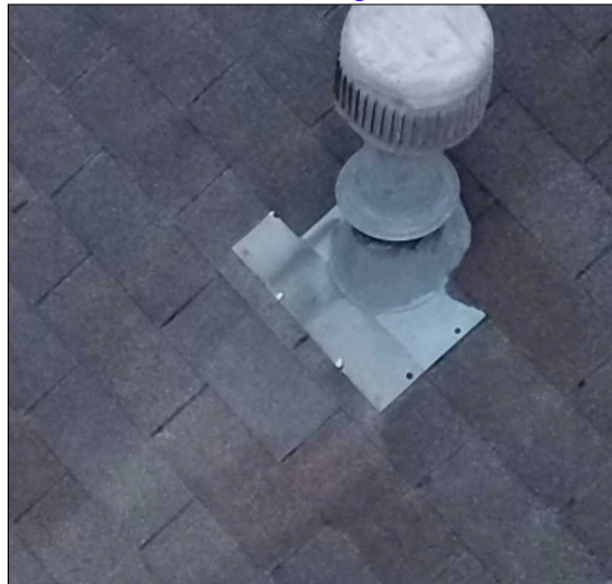
Exposed nails should be sealed over.
