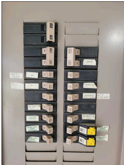
The electrical panel is not properly labeled.
