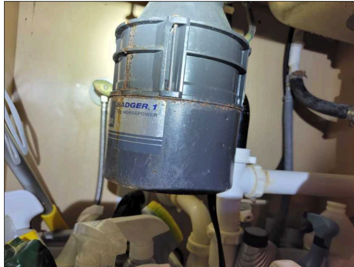
There is rust present on the disposal unit.
