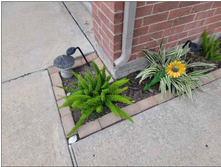
Gutters stop at edge of foundation. Gutters should terminate away from foundation or to a splash block.
