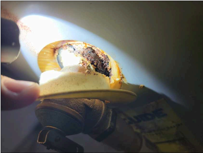
Rust on TPR valve and evidence of leaking. Repairs / tank replacement suggested.
