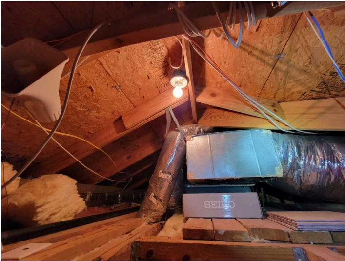
Attic light is a hazard based on its location.
