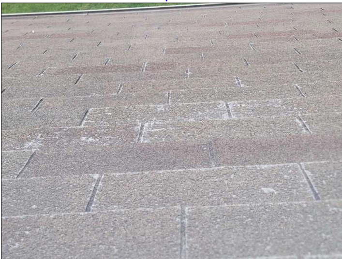
Multiple locations of granular lose. Suggest having roofing contractor to evaluate to check for full shingle replacement.
