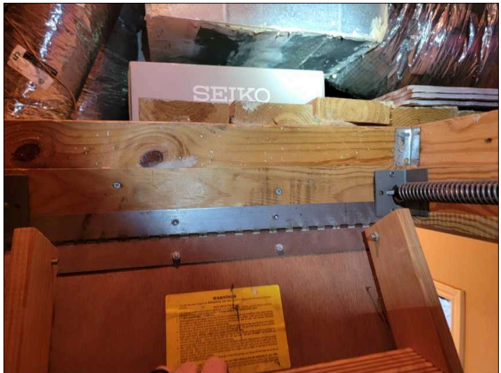
Ladder should be secured with 16d nails where indicated by manufacture, not screws.
