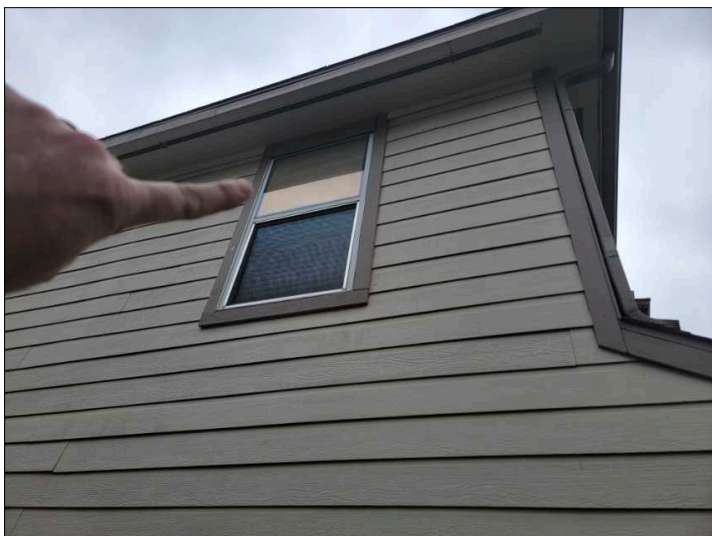
Condensation / fog present inside double pane windows. This is a sign that the gas between panes is gone, and the windows are less energy efficient and can be difficult to see through.
