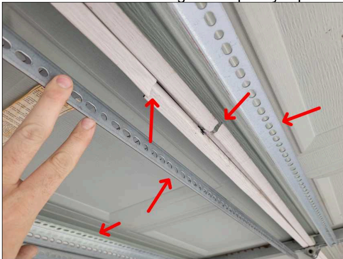
Damaged and poorly repaired garage door panels.
