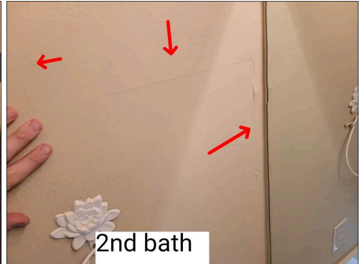
Structural settlement crack found in bathroom. Structure has movement and floors and walls are showing.
