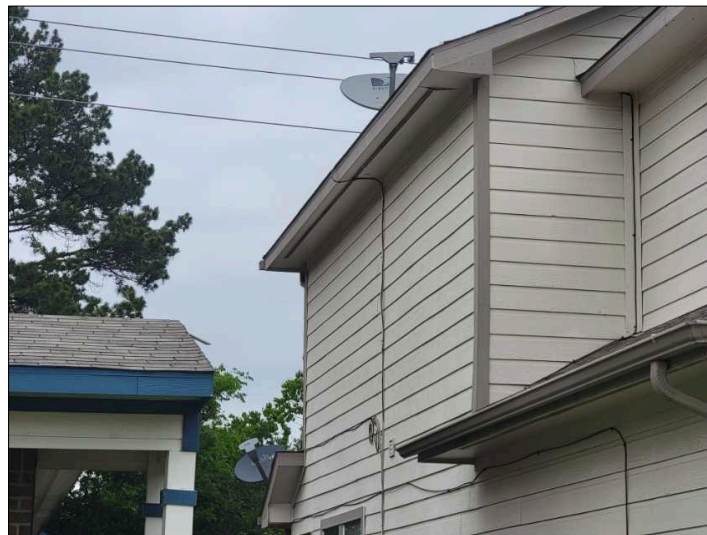
Satellite dish attached to house may add additional stresses to structure and cause damage or leaks. Monitor area for damages and leaks.
