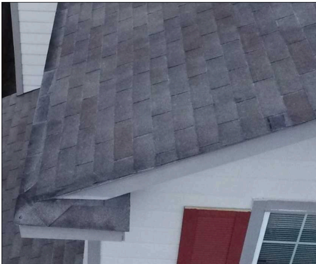
Shingles are missing / torn
