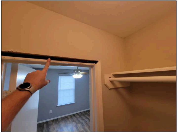
Missing trim inside closet
