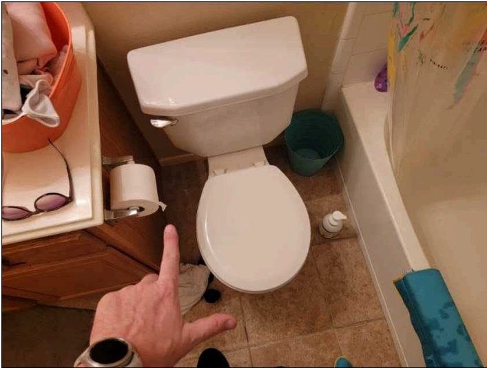
Toilets loose at base. New seal ring may be needed.
