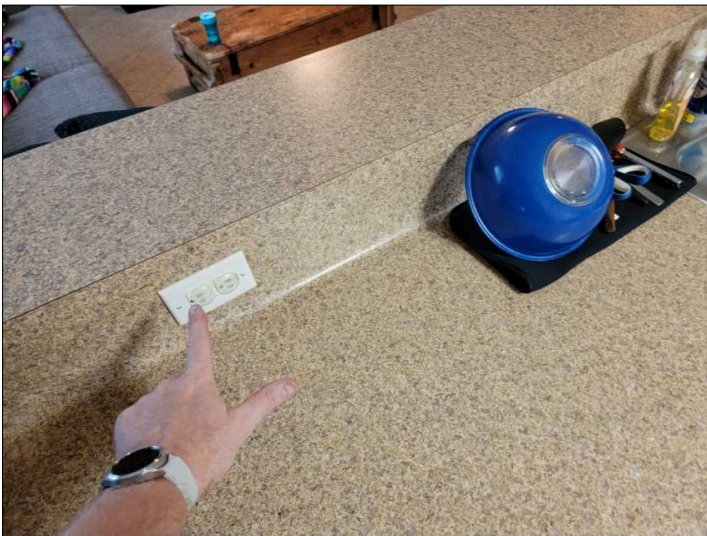
Loose receptacle found.
