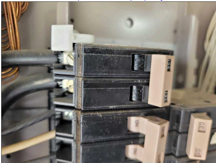
There is aluminum wiring present that does not have anti-oxidant grease
