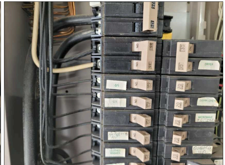
There are white wires in the panel that should be labeled as hot wires
