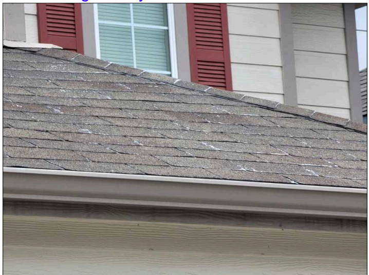
Multiple locations of granular lose. Suggest having roofing contractor to evaluate to check for full shingle replacement.
