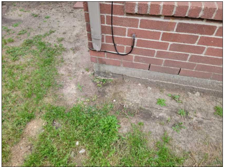
Damaged downspouts and gutters.
