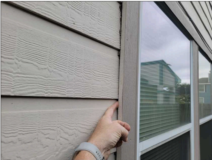
Siding not installed according to manufacturer directions. Trim should be installed first and siding cut to fit.
