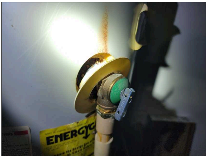
Rust on TPR valve and evidence of leaking. Repairs / tank replacement suggested.
