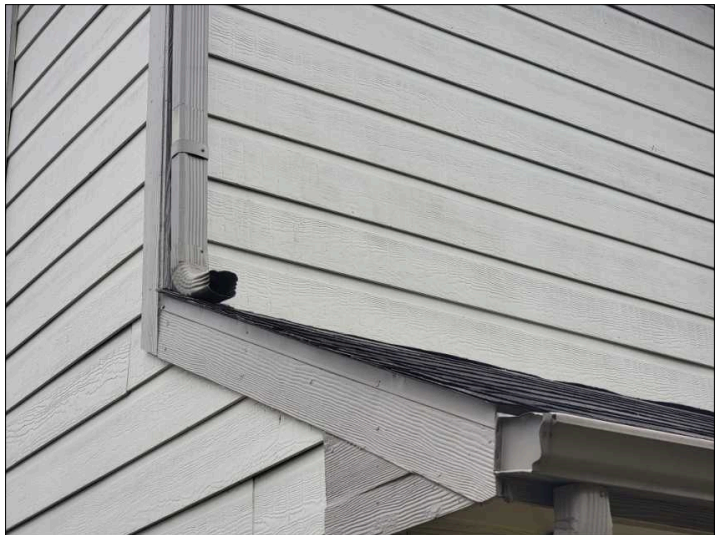
Gutters terminate on top of shingles. Gutters should extend to the ground or to another gutter. Shingles may wear faster in this area.
