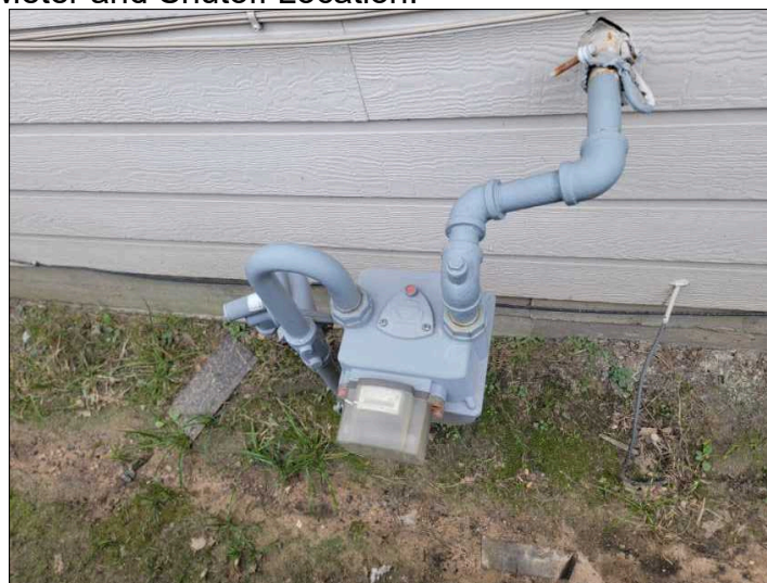
Gas Meter and Shutoff Location.
