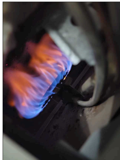
Burner flame is blue and orange indicating incomplete Combustion.
