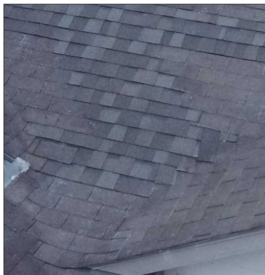
Evidence of previous repair. Multiple shingles present. Poorly attached and overlapped.
