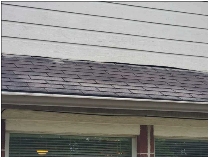
Lifted flashing. Should be flat and prevent water and wind penetration.
