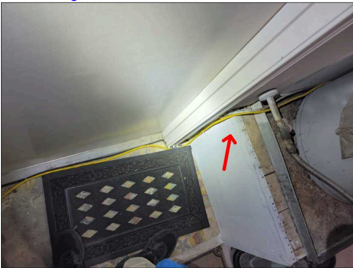
Extension cord used in garage. Garage only has 1 receptacle.
