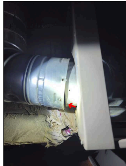
Furnace flue is disconnected in attic. High risk of CO leakage. Repairs needed. Repairs needed.
