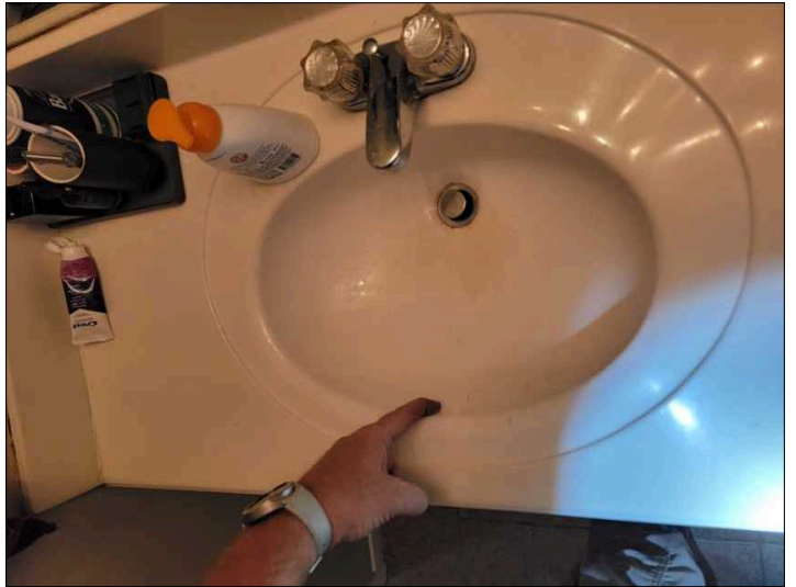
2nd floor lavatory does not have an overflow vent and can easily overflow.
