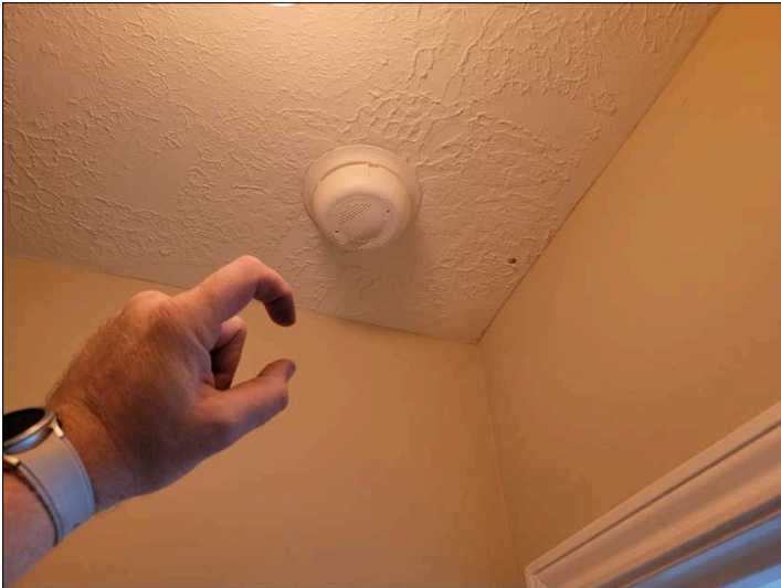
Recommend installation of CO detector 3" from ceiling in locations of a gas fired appliance.
