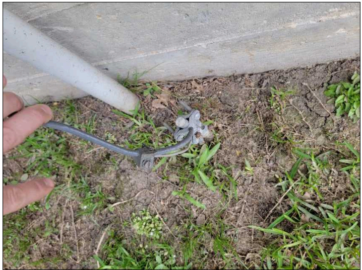
Incorrect ground clamp nut used.
