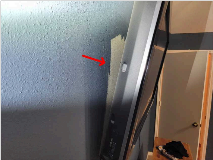
Paint behind TV not complete.
