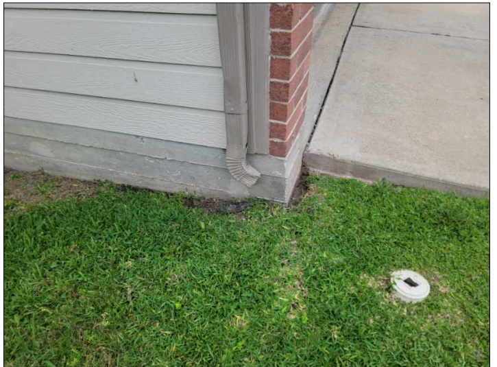
Damaged downspouts and gutters.
