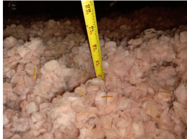
Attic Access Method: Pull Down Ladder
