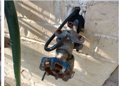
Water Line Bonding
