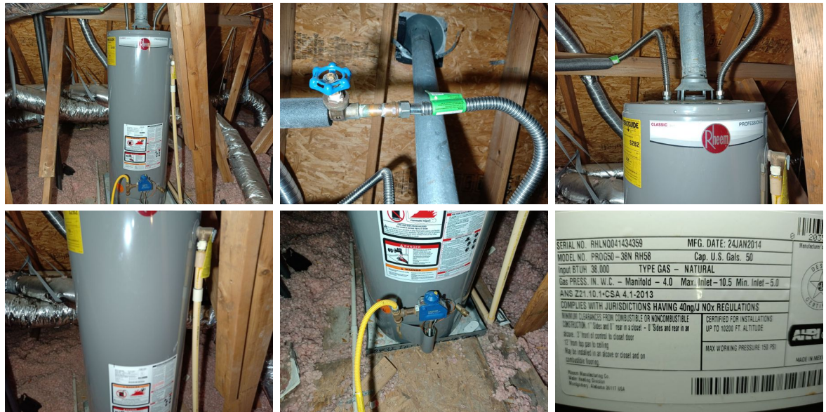
General Infrared Photos of Water Heating Equipment:
