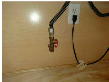
Cooktop Gas Shutoff Valve in Cabinet Below Cooktop
