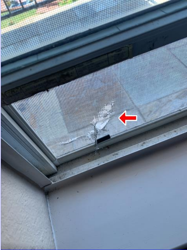
H. Item 3(Picture) There are damaged screens. Recommend repair.
