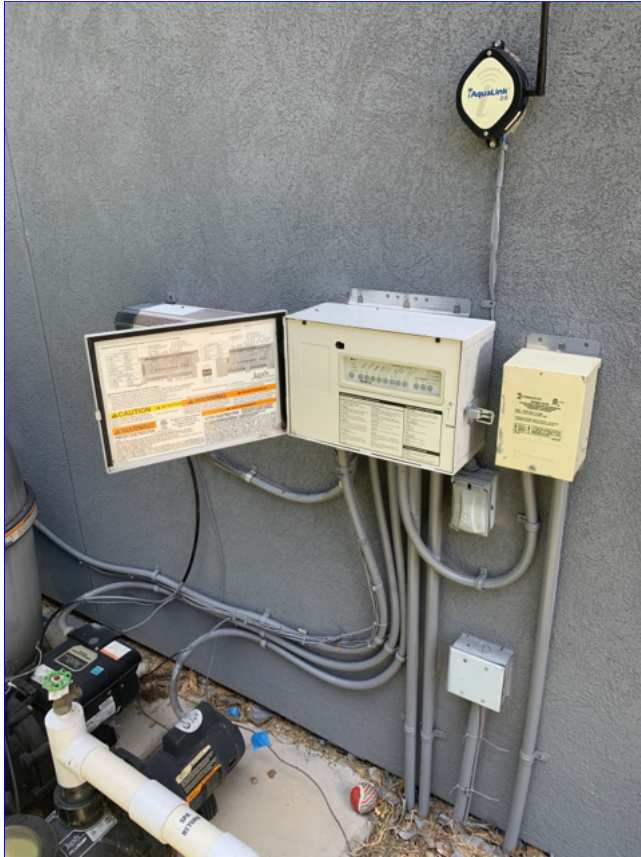
A. Item 1(Picture) Pool control observed at the pump.
