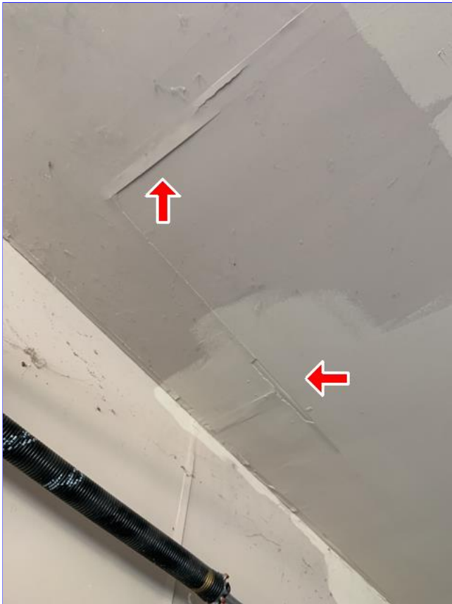
F. Item 3(Picture) Drywall tape joint cracks and/or nail pops were observed around the home.
