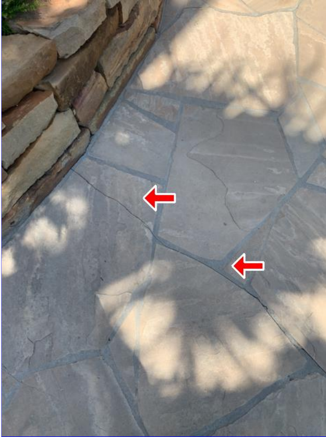
K. Item 2(Picture) Cracks where observed at the deck. Recommend repair.
