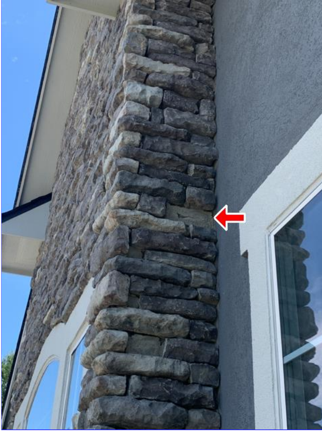
E. Item 4(Picture) Missing stones was observed at the front of the home. Recommend correction.
