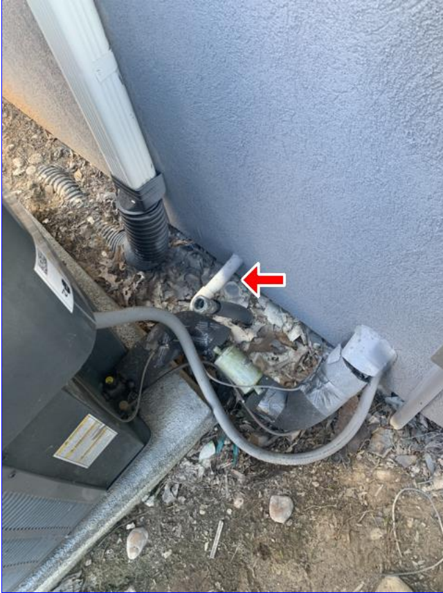
A. Item 3(Picture) The main water supply line at the exterior, is not properly protected from freezing.
