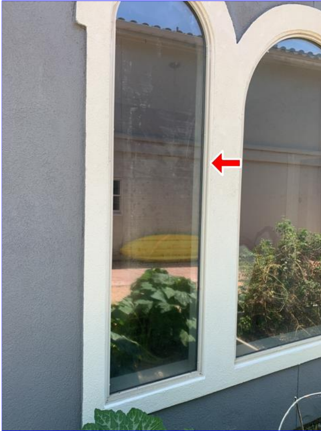
H. Item 1(Picture) Window seals appear to be compromised, as suggested by condensate and mineral deposits built up between the double panes of glass.
