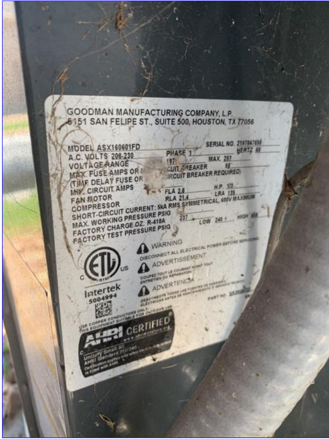
B. Item 1(Picture) AC service tag
