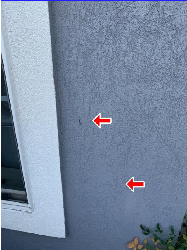
E. Item 6(Picture) Stucco damage and cracks or repaired cracks observed.
