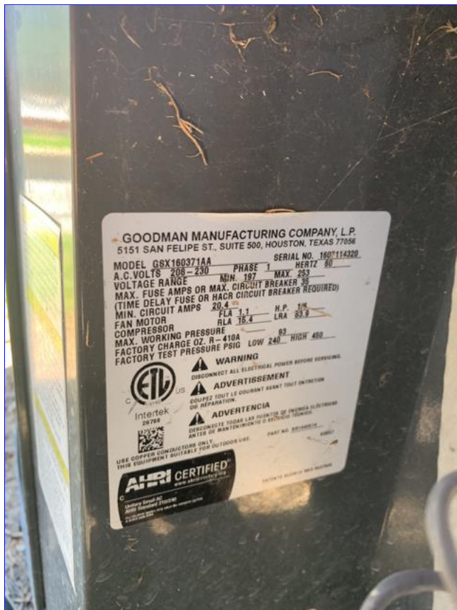
B. Item 2(Picture) AC service tag
