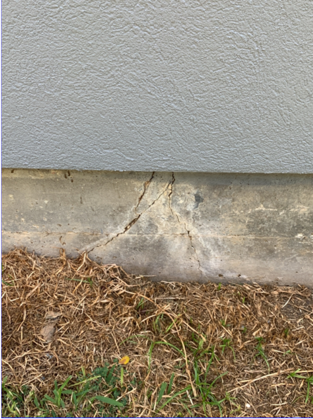
A. Item 1(Picture) There is some slab edge cracking.
