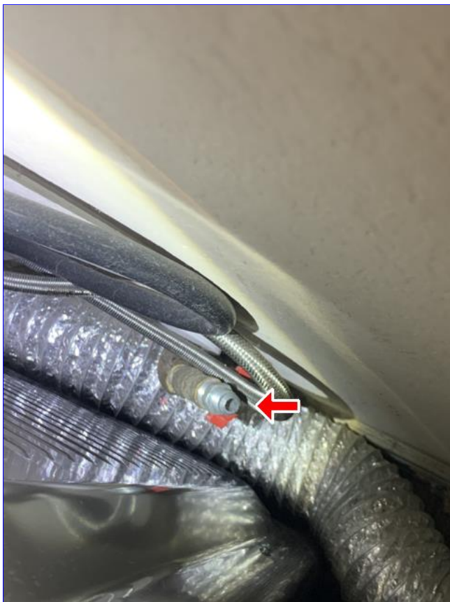
E. Item 1(Picture) The gas line at the clothes dryer location should be properly capped if not in use.
