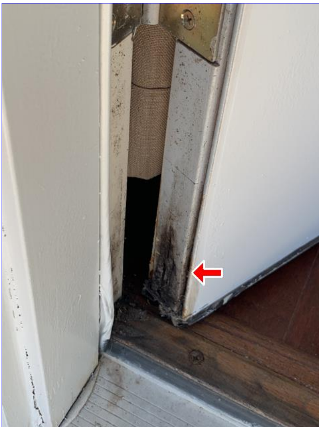
G. Item 1(Picture) Wood rot was observed on the patio door to the master bedroom. Recommend replacing.
