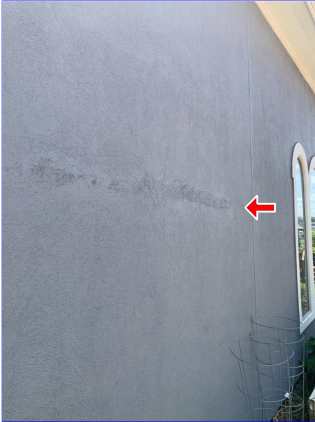
E. Item 8(Picture) Stucco damage and cracks or repaired cracks observed.
