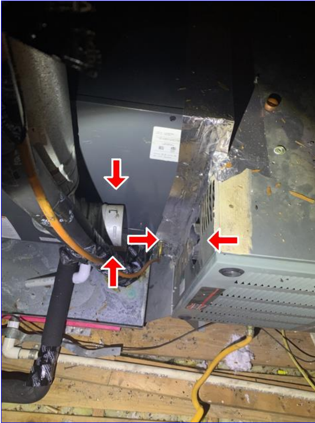
A. Item 5(Picture) The exhaust flue for the furnace is not connected. Exhaust fumes are going into the attic space. Recommend correction.
