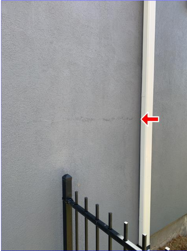
E. Item 9(Picture) Stucco damage and cracks or repaired cracks observed.
