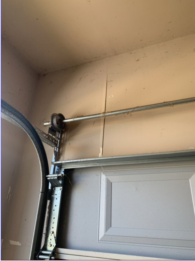
E. Item 1(Picture) Drywall tape joint cracks and/or nail pops were observed around the home.
