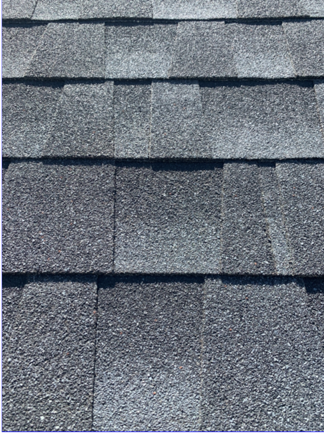
C. Item 1(Picture) The roof covering, is not new and shows signs of wear consistent with its age.
