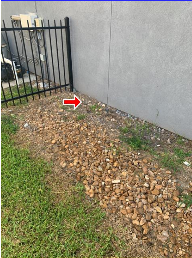
B. Item 2(Picture) High soil conditions observed at left side (facing front).
