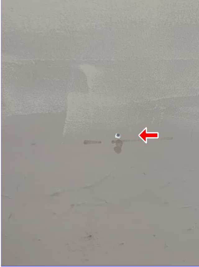
F. Item 1(Picture) Drywall tape joint cracks and/or nail pops were observed around the home. These are cosmetic in nature, and can be repaired as needed.
