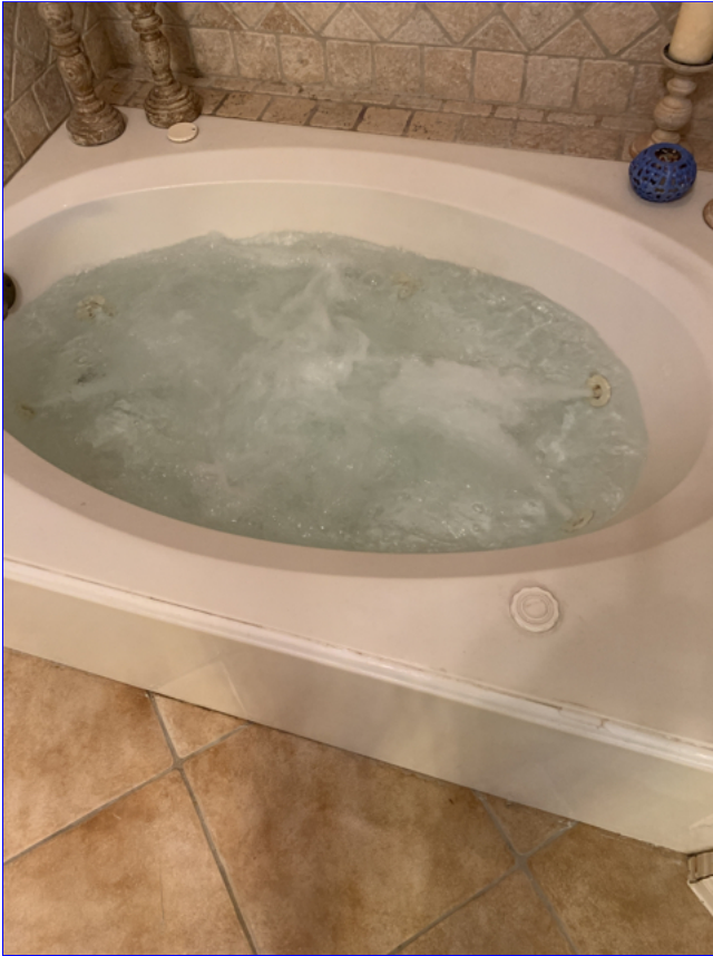
D. Item 1(Picture) A readily accessible inspection port is not available.
