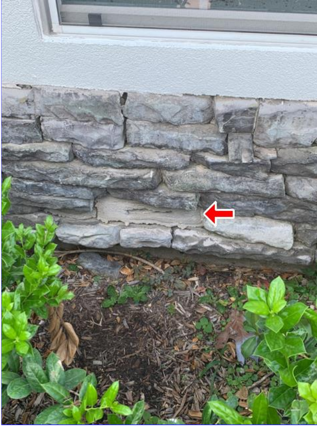
E. Item 5(Picture) Missing stones was observed at the front of the home. Recommend correction.
