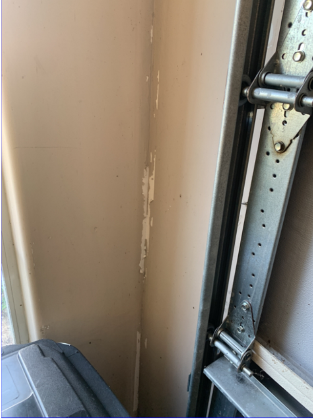
E. Item 2(Picture) Drywall tape joint cracks and/or nail pops were observed around the home.
