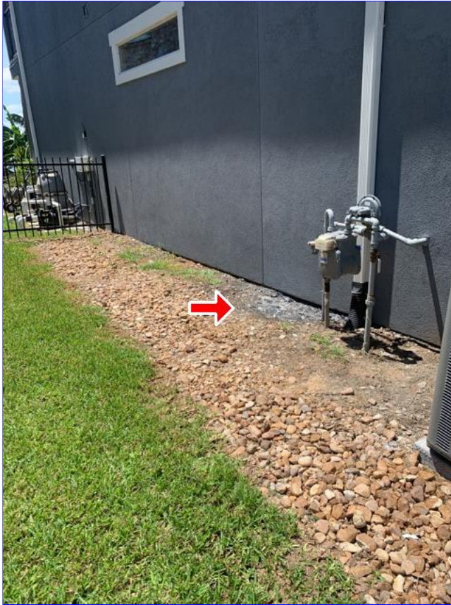
B. Item 1(Picture) Drainage swales at the sides of home appears to have low spots.
