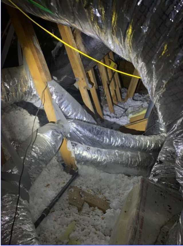
D. Item 2(Picture) Walkways and/or service platform(s) not installed to access mechanical equipment in the attic.
