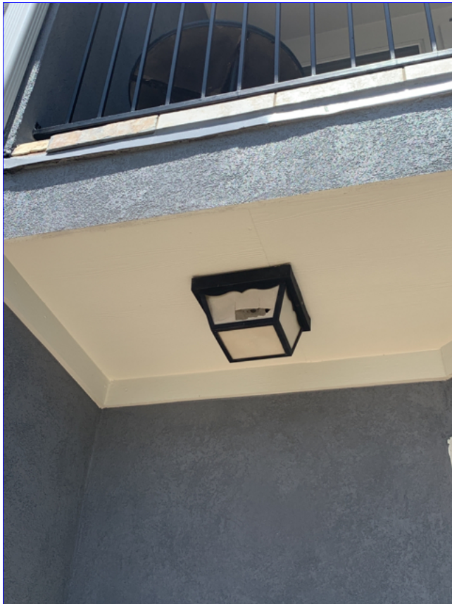
B. Item 2(Picture) The light cover is broken at the back porch. Recommend replacing.
