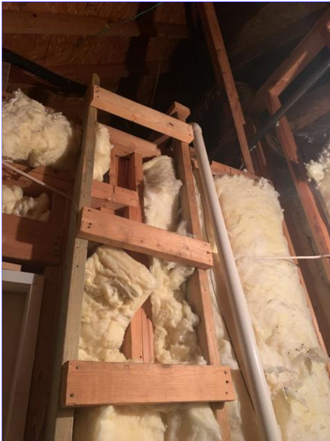
D. Item 3(Picture) Walkways and/or service platform(s) not installed to access mechanical equipment in the attic.
