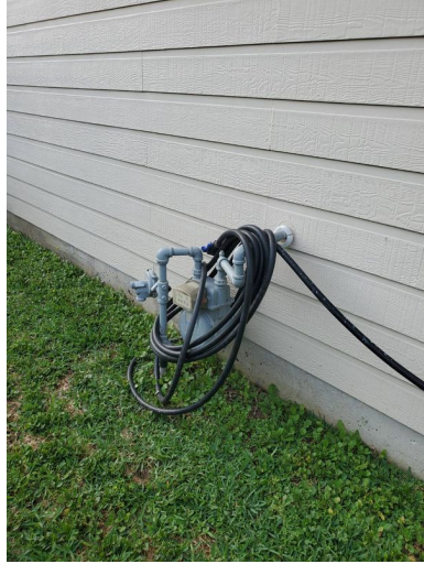
Type of gas distribution piping material: Black metal
