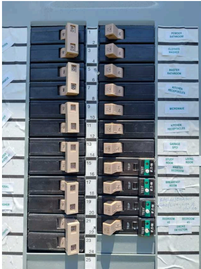
Picture of breakers
