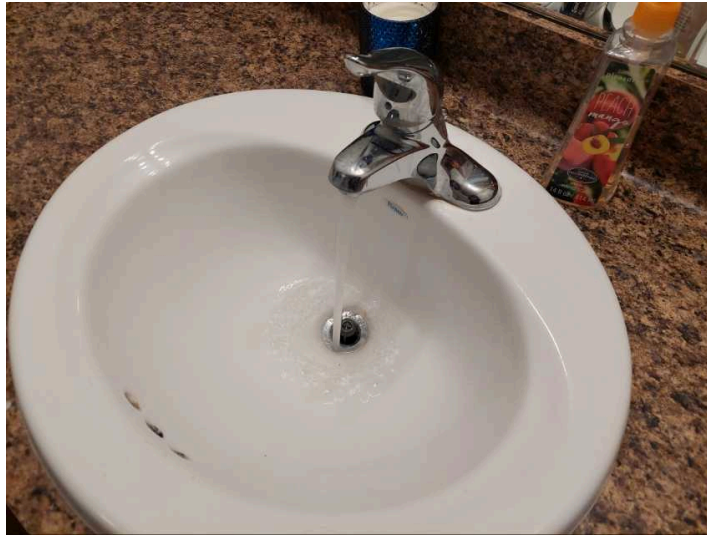
Drain stop does not function properly
