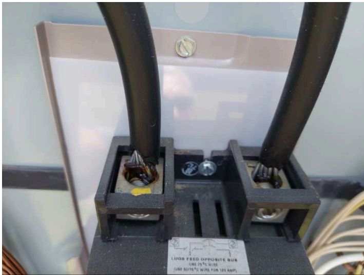
Aluminum service conductors missing anti-oxidant grease
