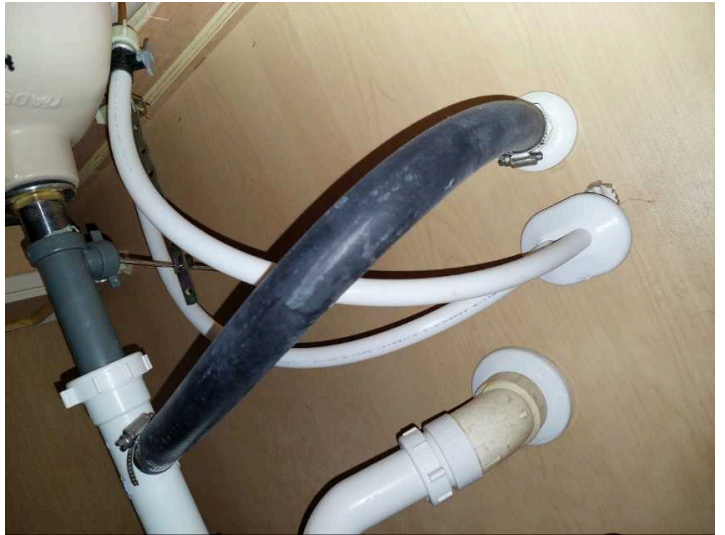
Picture of water supply lines - plastic
