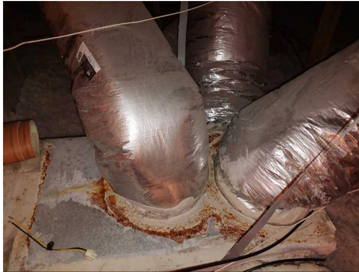
Picture of ducts in attic
