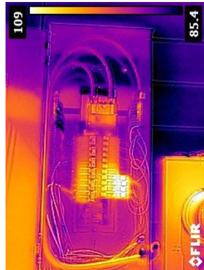
Thermal imaging camera used to detect over heating electrical components. No issues.
