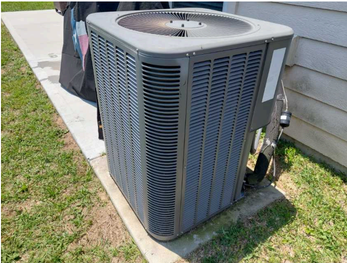
AC condensing unit
