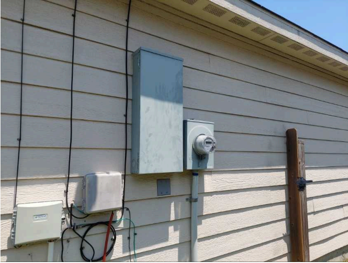
Picture of electrical service panel
