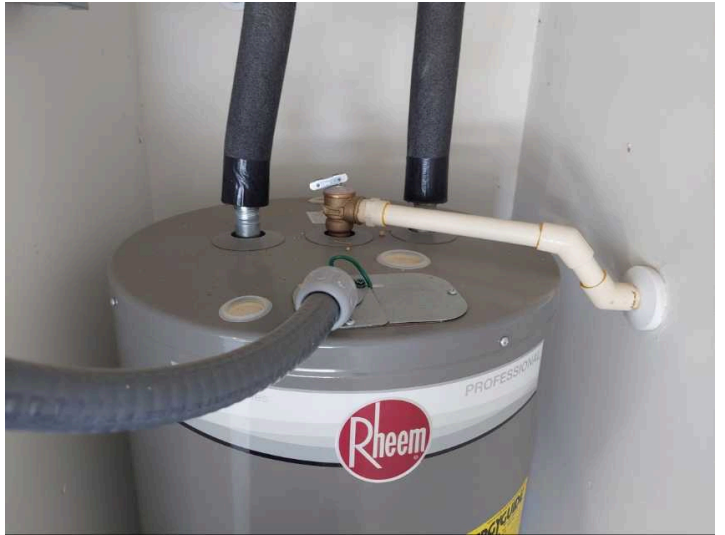
Water heater temperature and pressure relief valve is damaged - did not trip
