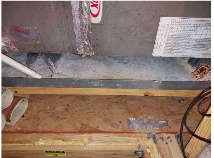
Evaporator overflow pan has corrosion and should be monitored for further degradation
