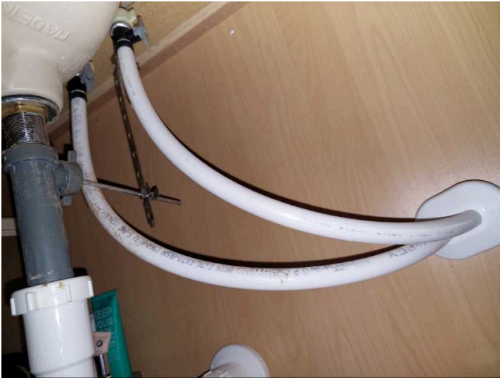
Picture of water supply lines - plastic
