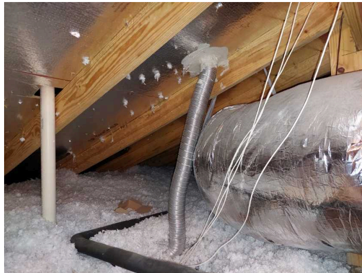
Bath fan ducts
