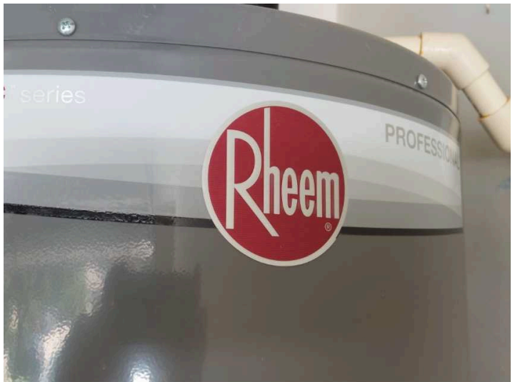
Water heater brand name
