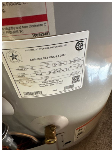
Water heater location: Attic
