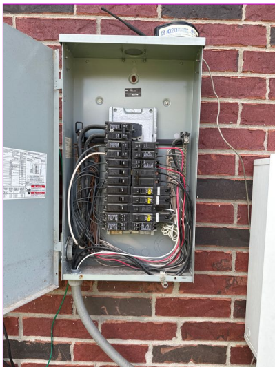
Electric panel interior
