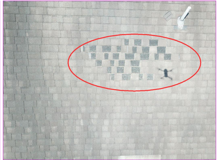
Missing shingles (zoomed view)
