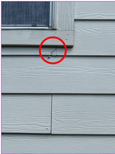
Localized siding damage (right side)
