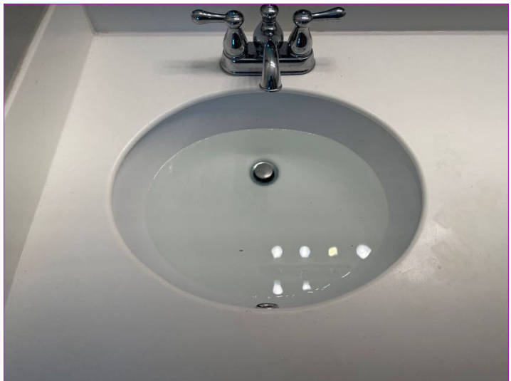
Slow sink drain (master bathroom)
