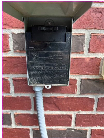
AC main disconnect OK
