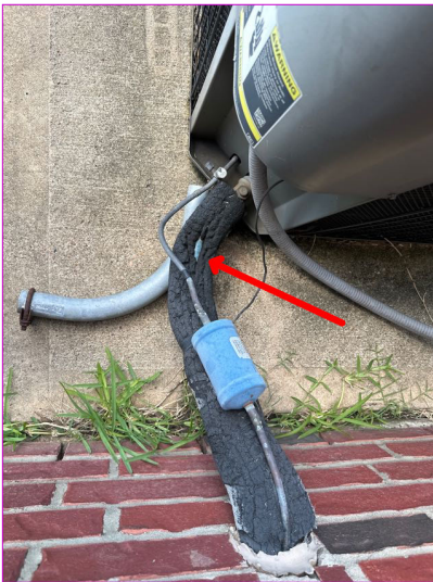
Damaged AC line insulation
