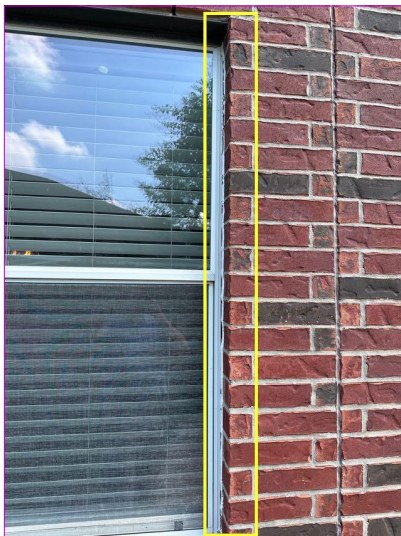
Window frame wall separation (right side)
