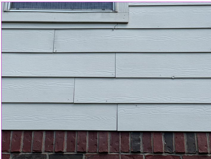
Siding gaps (right side)
