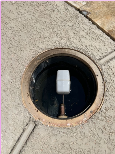
Automatic water filler OK
