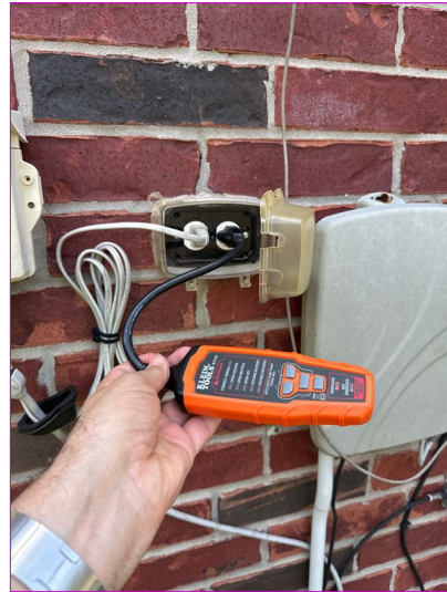
Faulty GFCI receptacle (right side)
