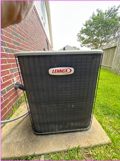
2007 Lennox AC condenser (right side)
