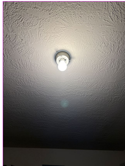
Damaged light fixture (master bedroom closet)
