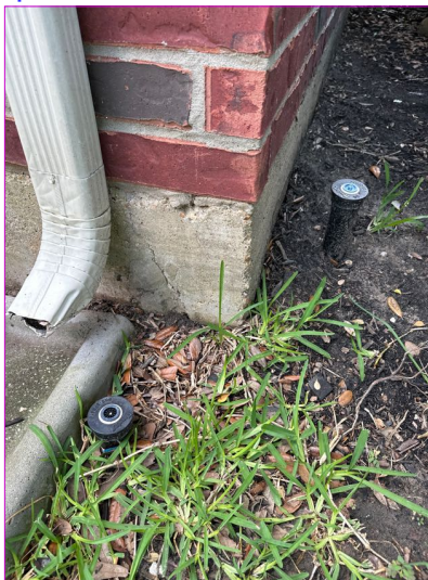
Corner crack (front-left)
