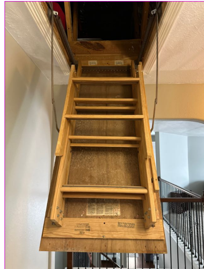
Attic ladder missing insulation
