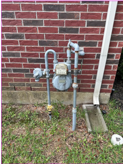
Gas meter (left side)
