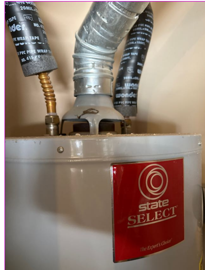
Pipe fittings OK
