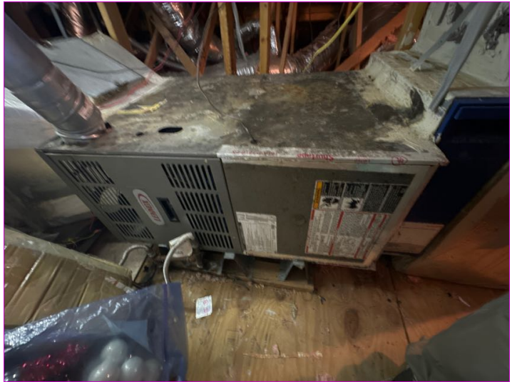
Lennox gas furnace
