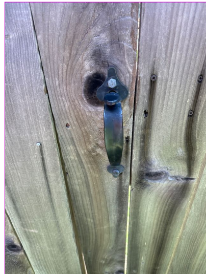
Gate lock needs adjusting
