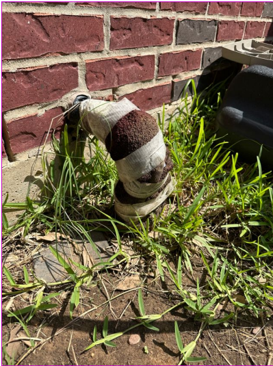
Unable to operate main water shut off valve (right side)
