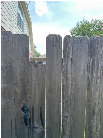
Damaged fence picket
