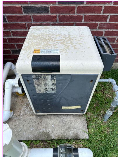
Gas furnace OK
