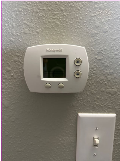
Inoperative thermostat (upstairs hallway)
