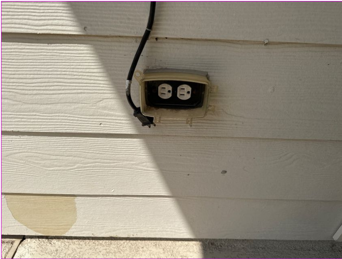
Exterior receptacle missing cover (rear side)
