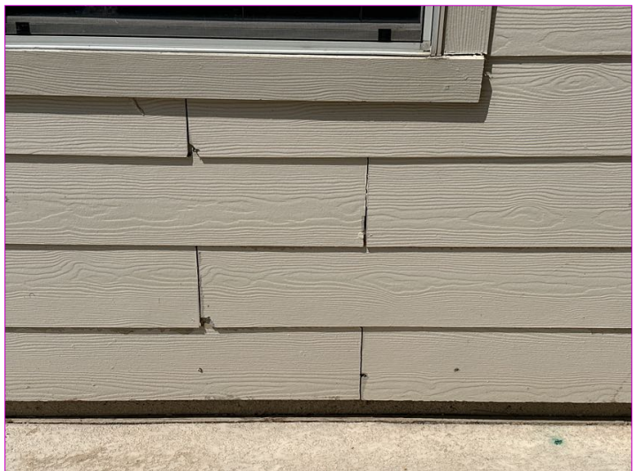
Siding gaps (rear side)
