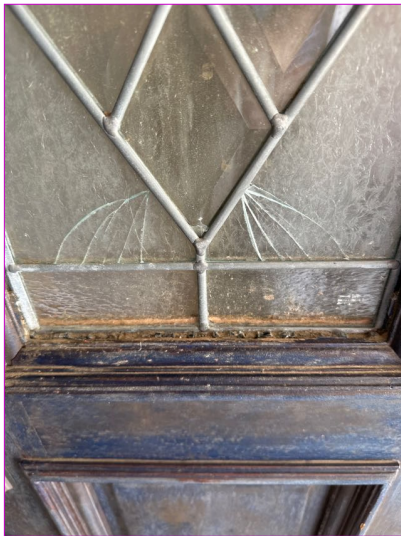
Cracked pane (entry door)
