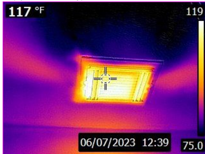
Furnace hot air temperature
