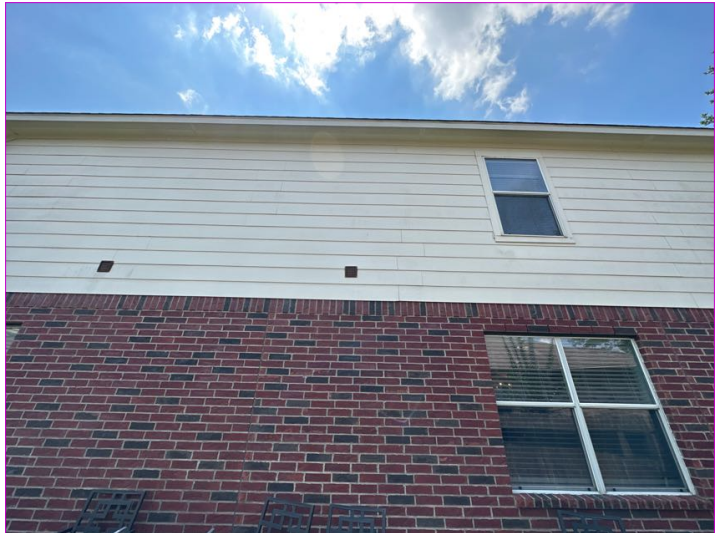
Siding gaps (left side)
