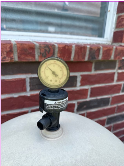
Pressure gauge OK
