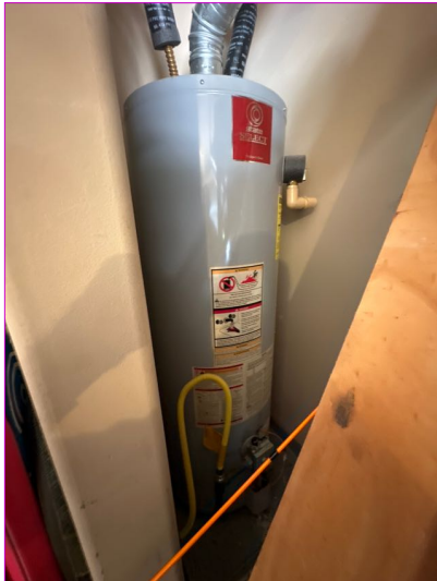
2007 State gas water heater
