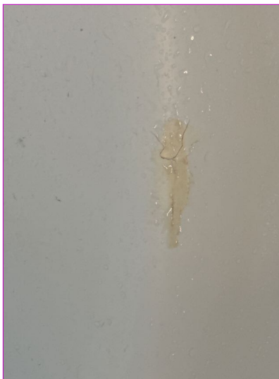
Tub cosmetic damage (master bathroom)
