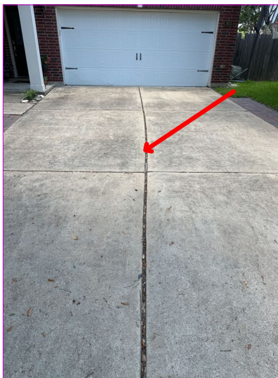
Expansion joint missing caulking
