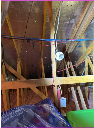
Inoperative light fixture (attic)
