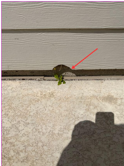
Localized siding damage (rear side)
