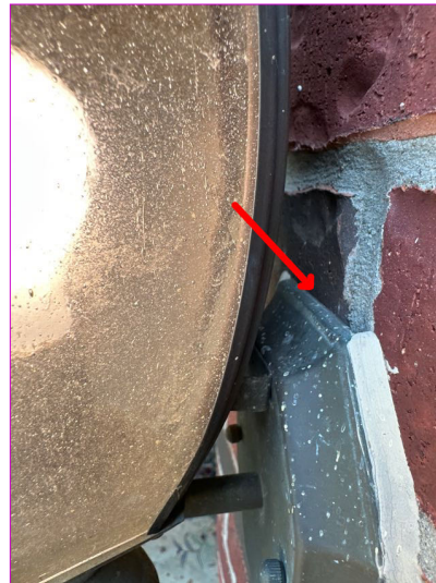
Missing sealant around exterior light fixture (entry)
