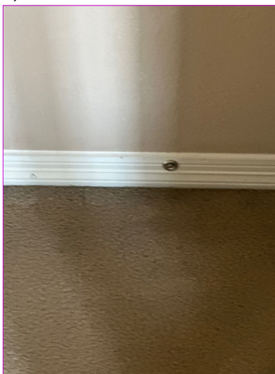
Missing door stop (upstairs bedroom)
