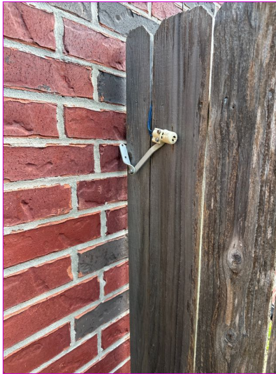
Loose rain sensor
