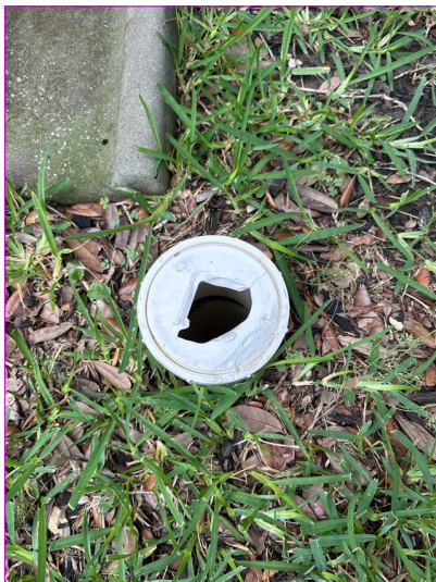
Damaged clean out cover (left side)
