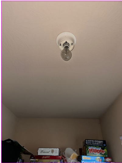
Damaged light fixture (upstairs bedroom closet)
