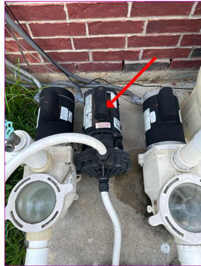
Cleaner pump OK
