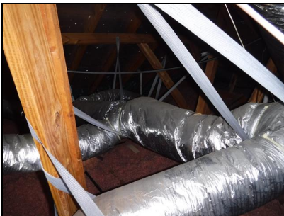
Vent cover within living room loose. Repair as needed
