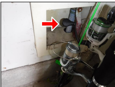
Main water shut off located within the garage.
