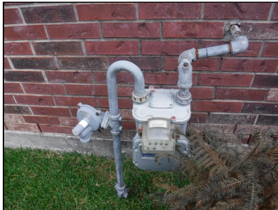
Gas meter located left side of residence.
