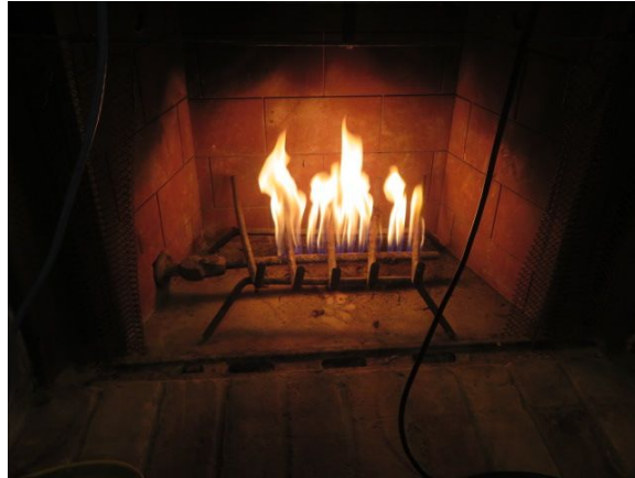
There are cracks in the bottom of the fireplace.
