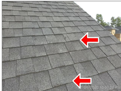
Front: Worn Shingles
