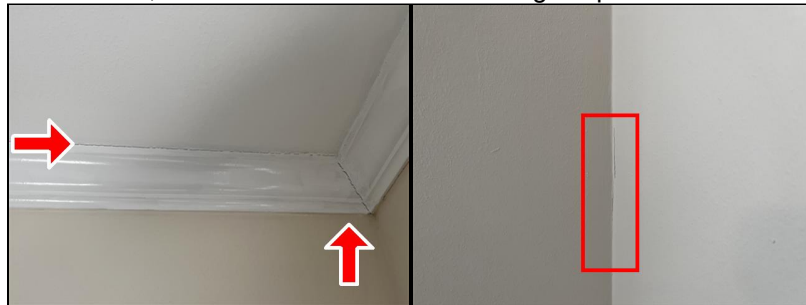
Cracks on walls in various areas, consistent with structural settling. Repair as needed.
