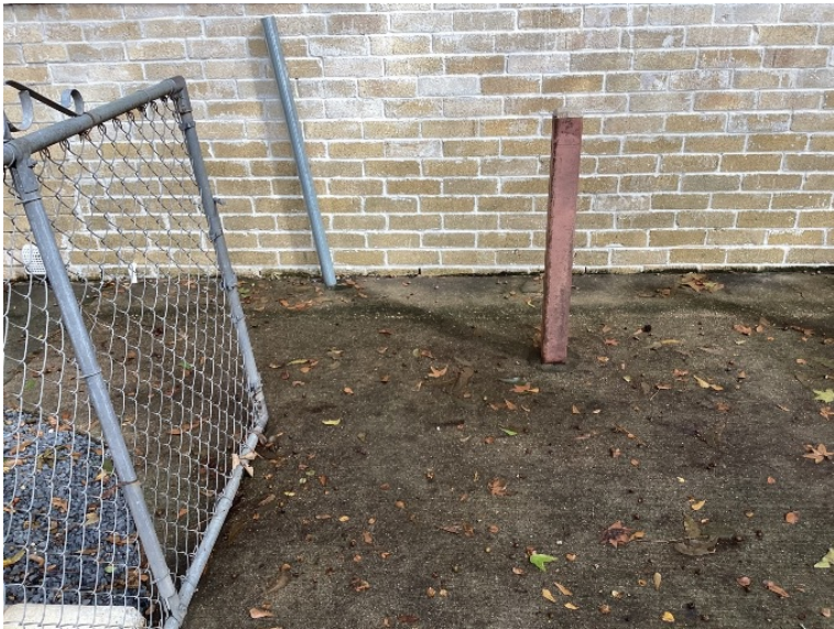
At the right side of the home, a driveway has been poured against the home with a negative slope. This driveway is in place above the bottom run of the brick and is obstructing some weep holes along the rear section.
