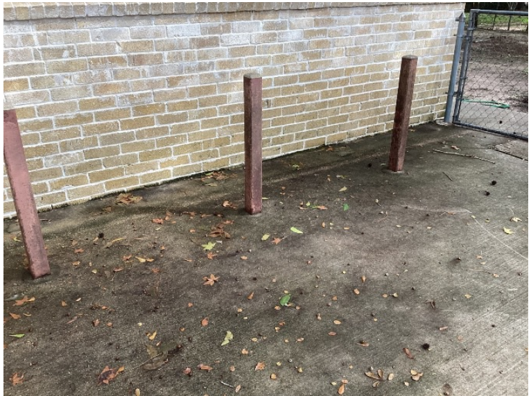
At the right side of the home, a driveway has been poured against the home with a negative slope. This driveway is in place above the bottom run of the brick and is obstructing some weep holes along the rear section.
