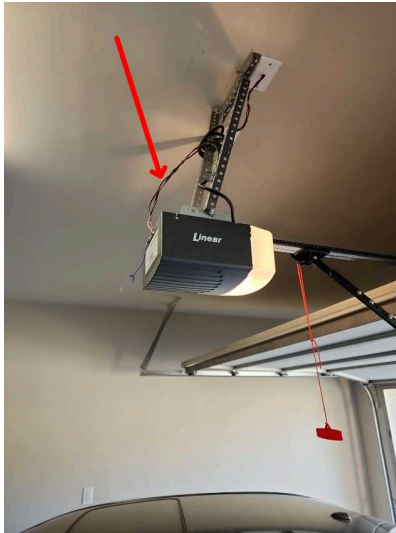
Garage door operator
