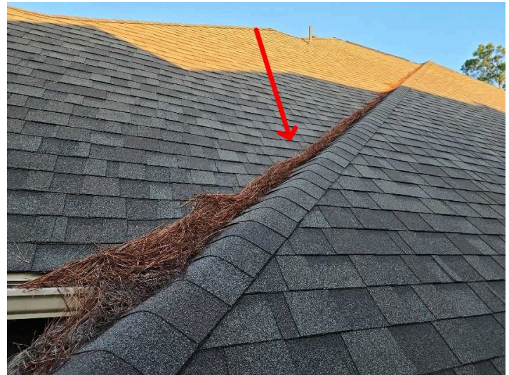
Debris should be removed from the roof coverings to prevent future damage.
