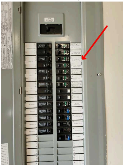
Electrical supply distribution panel
