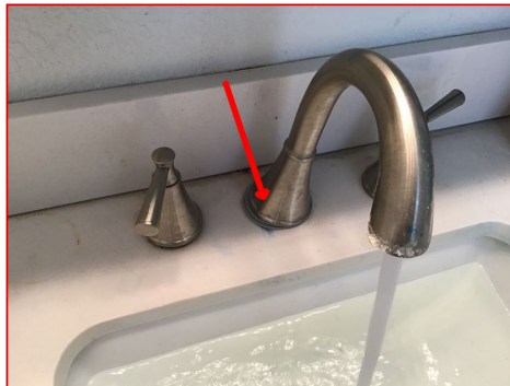
Loose faucet, attached bath sink
