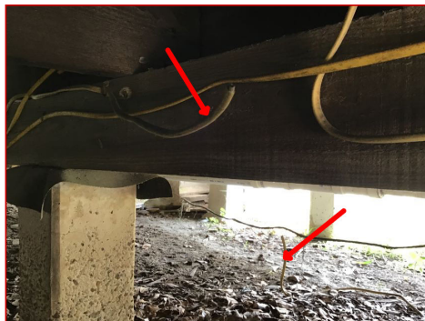
Example of improperly terminated wires
