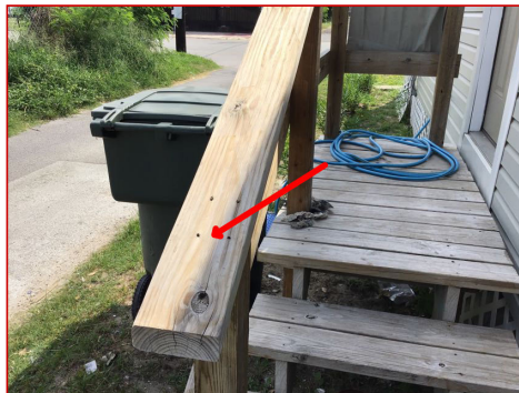
Non graspable handrail
