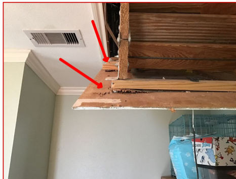
Damaged attic ladder
