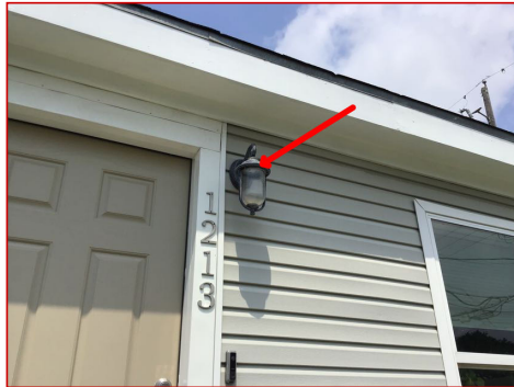
Inoperative exterior light
