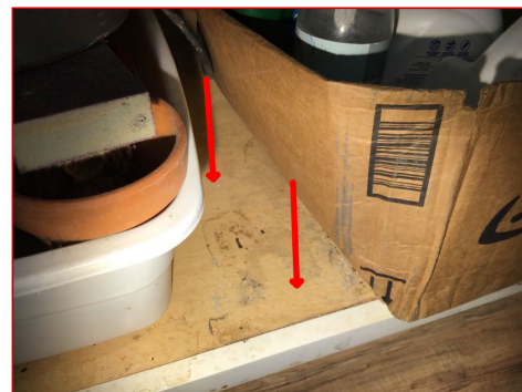
Evidence of prior moisture intrusion
