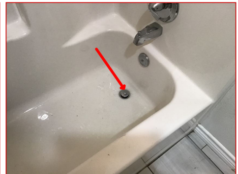
Slow to drain, hall bath tub
