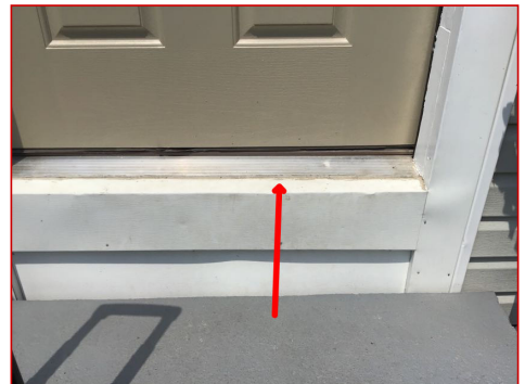
Exceeds maximum riser height
