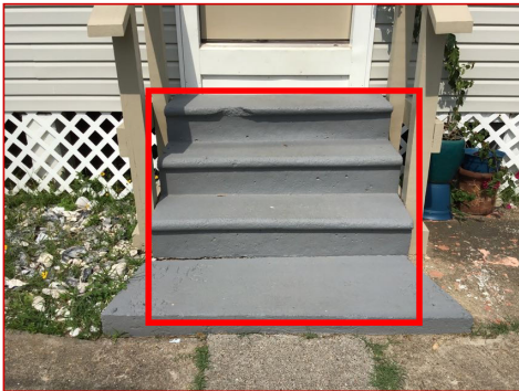
Uneven stairway/ riser height varies
