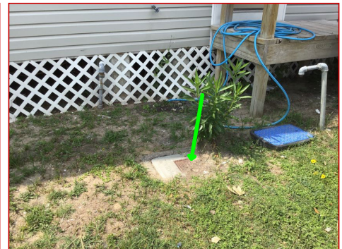
Water meter location
