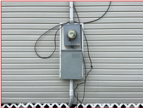
Service panel/ meter location
