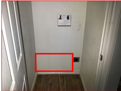
Laundry area/ no vent to exterior
