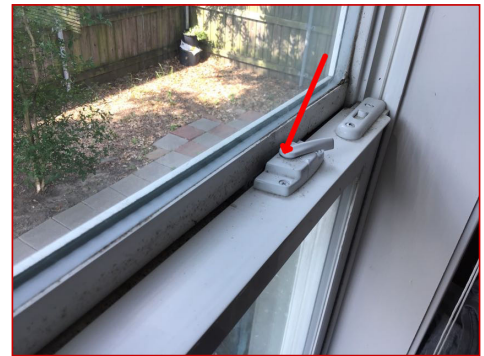
Misaligned latch, rear bedroom
