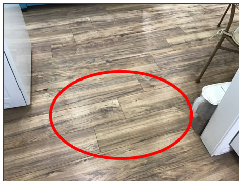
Soft area noted
