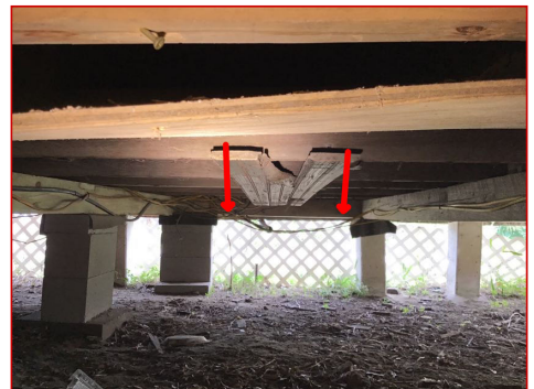
Example of unsupported wires, below structure
