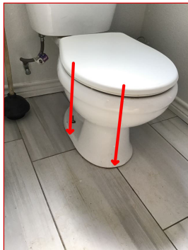
Loose at floor/ missing sealant
