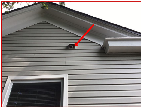
Improper auxiliary drain location
