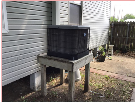
Condenser unit location
