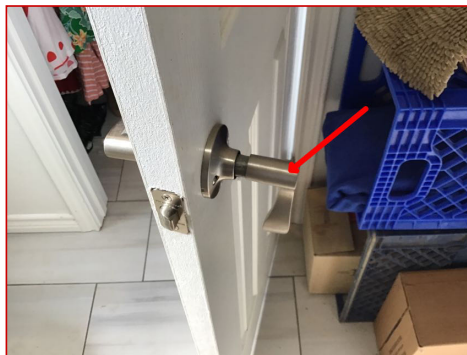
Loose hardware, bath closet
