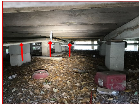
Improperly sloped primary drain pipe
