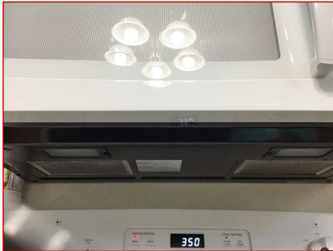
Range hood/ inoperative
