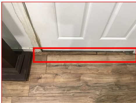
Damaged laminate flooring
