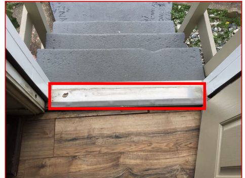
Inadequate support below threshold
