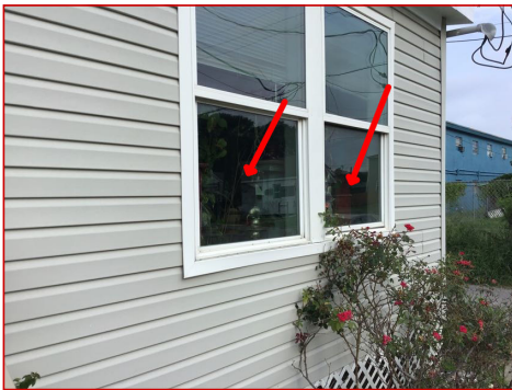
Example of missing screens
