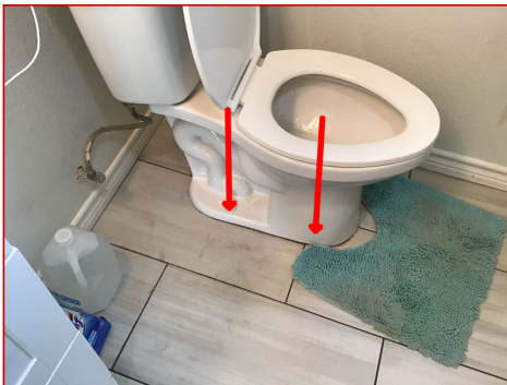
Loose at floor/ missing sealant, hall bath
