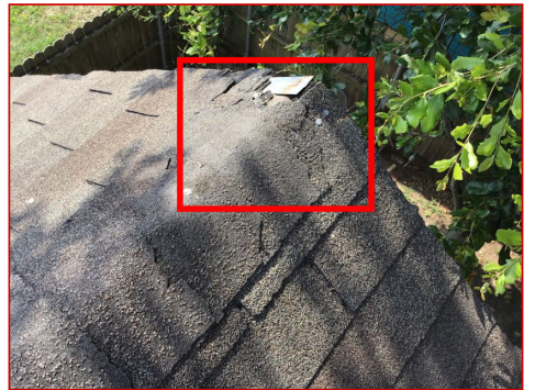
Damaged/ missing shingles
