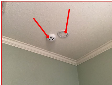
Inoperative/ missing smoke detectors
