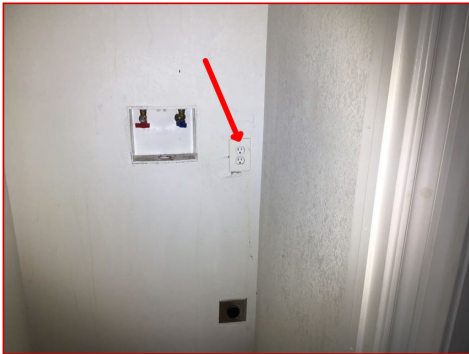
Loose outlet, laundry area
