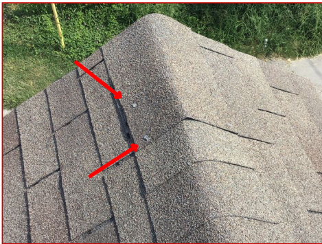
Example of exposed nail heads
