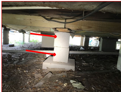
Leaning support column
