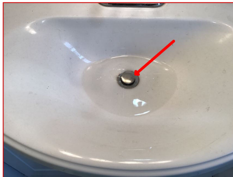
Slow to drain, hall bath sink
