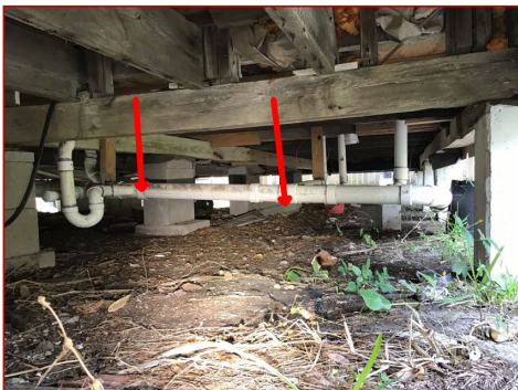
Inadequate support for waste line
