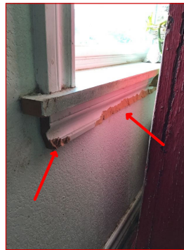
Damaged trim, living room
