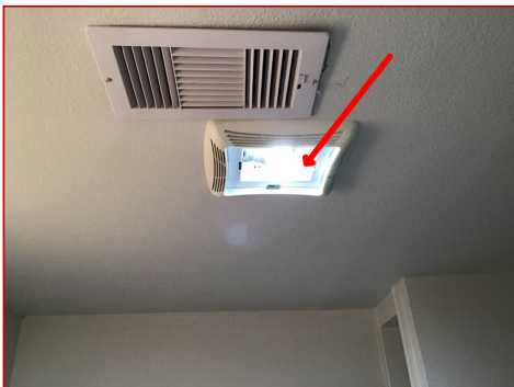
Missing diffuser, hall bath
