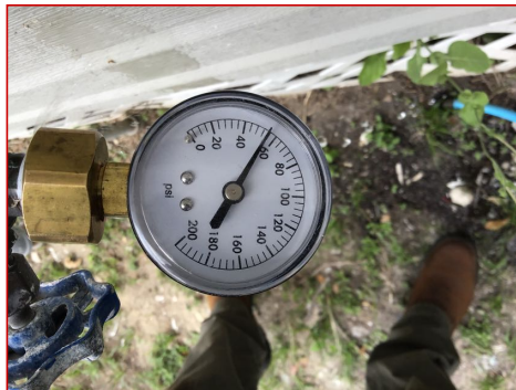
Static water pressure approximately 55 psi
