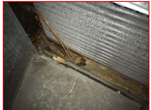
Coils appear ok
