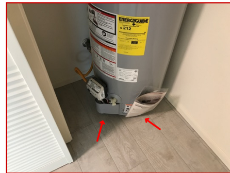
Missing catch pan at water heater
