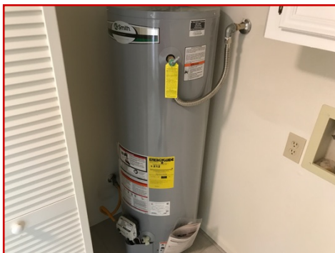
Water heater in laundry room
