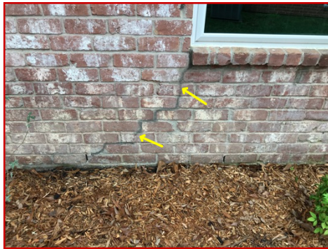
Crack at right of house
