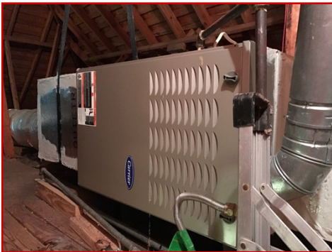
Furnace in attic space
