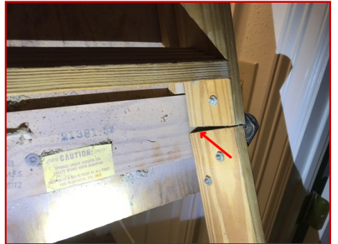
Gaps at ladder hinges
