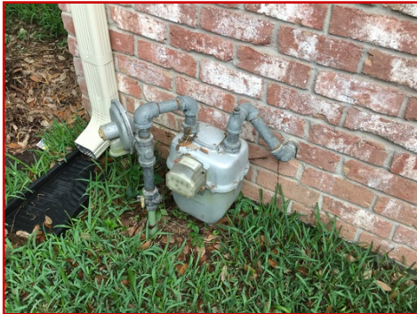
Gas meter at left of house
