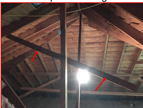
Apparent loose collar tie
