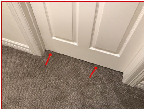
Bedroom doors are rubbing on carpet
