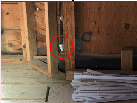
Gaps in flashing
