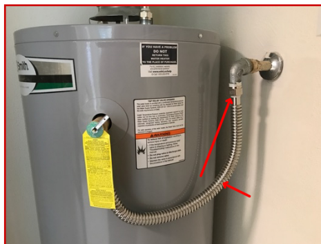
TPR valve, improper slope, possible improper material
