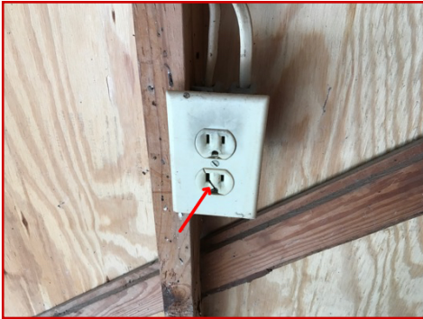
Damaged outlet in garage
