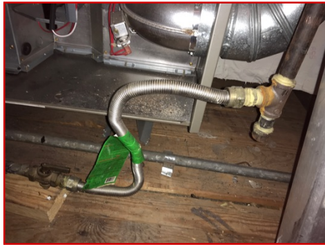
Gas supply appears ok
