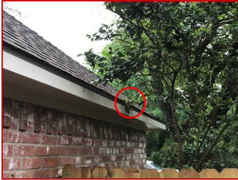
Tree touching structure
