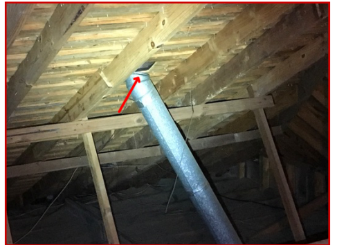
Detached vent hood exhaust in attic
