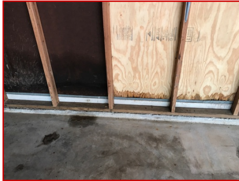
Moisture intrusion in siding
