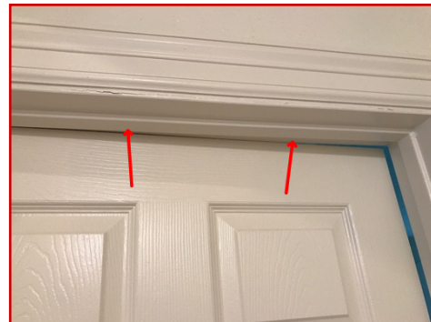
Front bedroom door rubs on jamb, will not close
