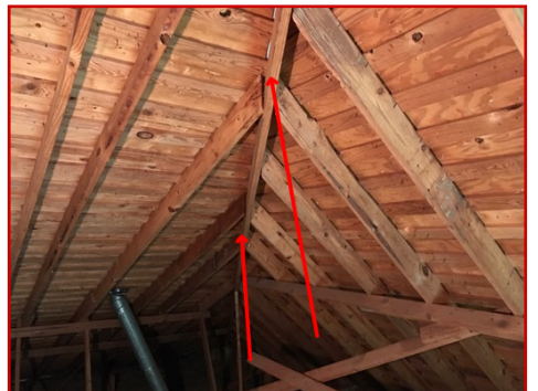
Rafter has no support after joint
