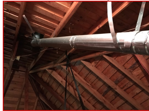
Venting appears ok
