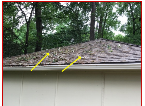
Debris on roof surface
