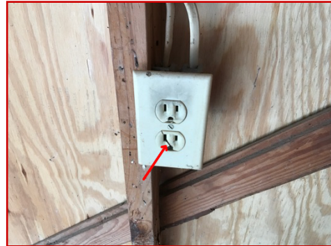
Damaged outlet in garage
