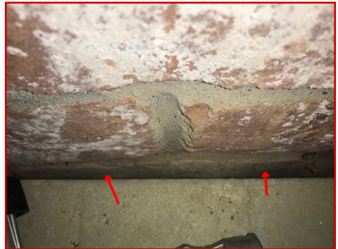
Meter is not securely mounted
