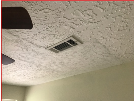
Ceiling patch in bedroom
