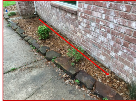
Inadequate foundation clearance to grade
