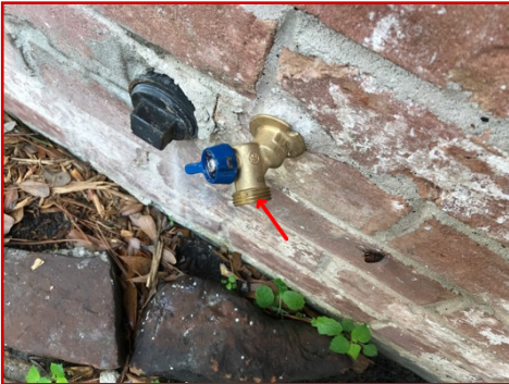
Missing anti siphon valve
