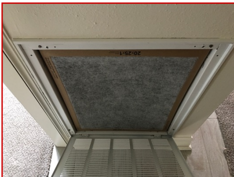
Return in living room wall, filter appears ok
