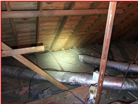
No visible termination for bath fan in hallway bathroom
