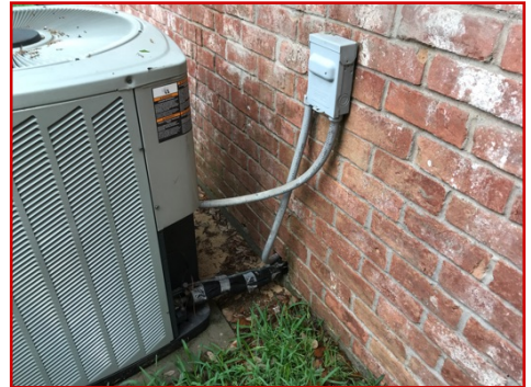
Line insulation and shut off appear ok
