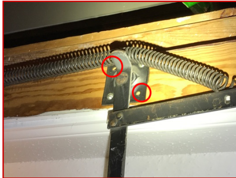
Improper/missing fasteners in attic ladder
