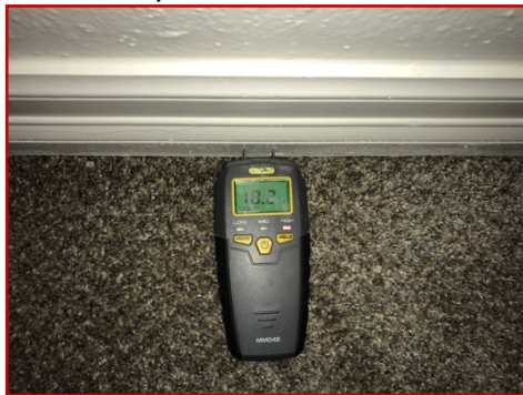
Elevated moisture levels in the master bedroom base board
