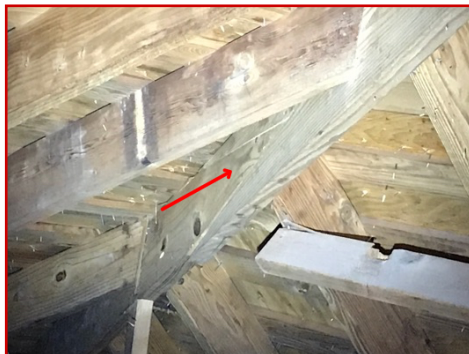
Joint is poorly secured
