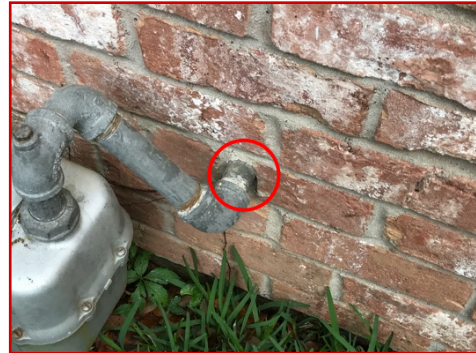
Missing protective cover at entry point
