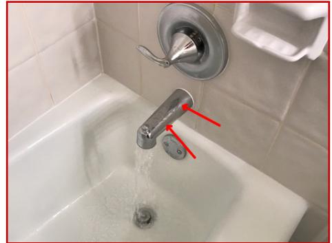
Hallway tub spout is extremely loose
