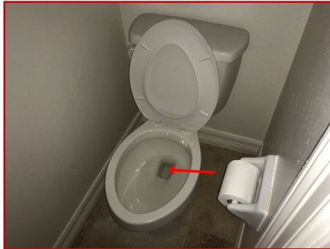
Master toilet runs continuously
