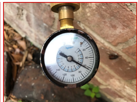
Static pressure approximately 60 psi
