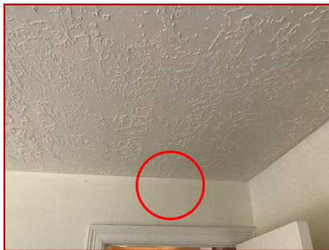
Missing smoke detectors in bedrooms
