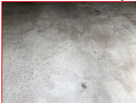
Typical cracks in garage floor
