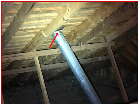
Detached vent hood exhaust in attic
