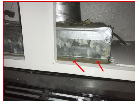
Range hood is not properly sealed in cabinet
