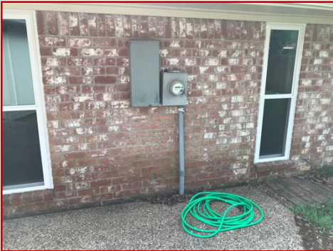
Service panel, meter and driven rod ground at rear of house
