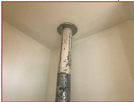
Venting appears ok
