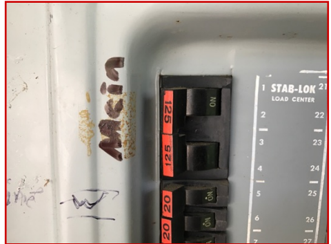
125 amp main breaker
