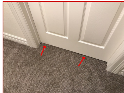
Bedroom doors are rubbing on carpet
