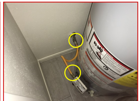
Missing sediment trap in gas supply
