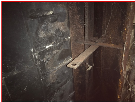
Damper appears functional
