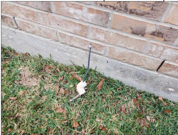
Conduit for protecting sprinkler wiring damaged
