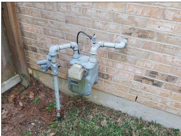
Gas Meter and Shutoff Location.
