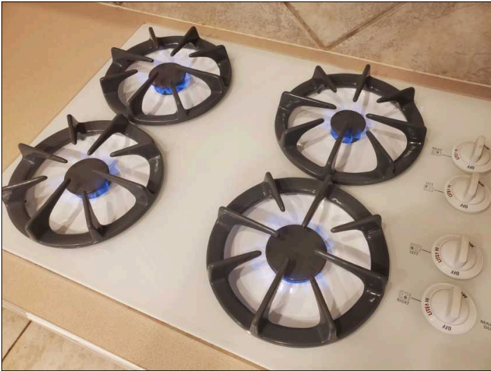
All heating elements operated when tested.
