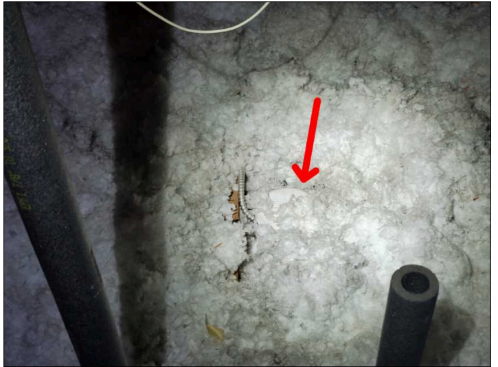
Canned lights need minimum 3" clearance from insulation unless labeled otherwise. (Unable to verify label).
