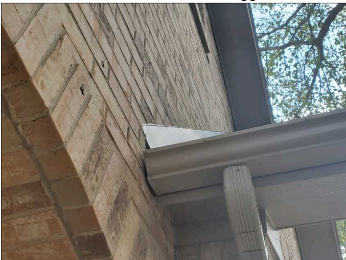
Missing kick out flashing to divert water away from house or areas of possible damage.
