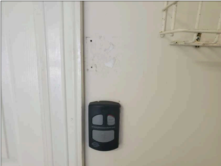
Missing safety test instructions on wall next to the operators.
