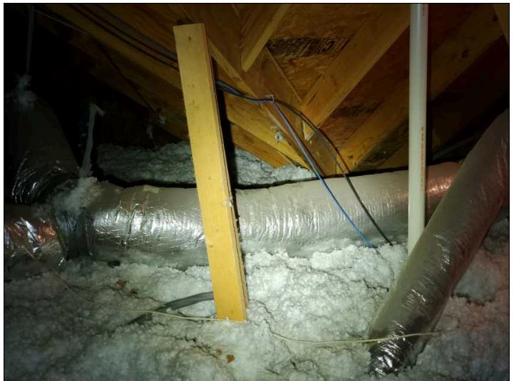
Flex ducting in contact with blown in insulation. This can cause mold growth. Flex ducting should be fully suspended.
