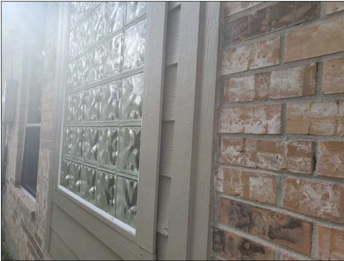
Recommend exterior siding weather proofing
