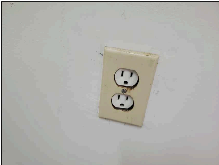
Loose receptacle found.
