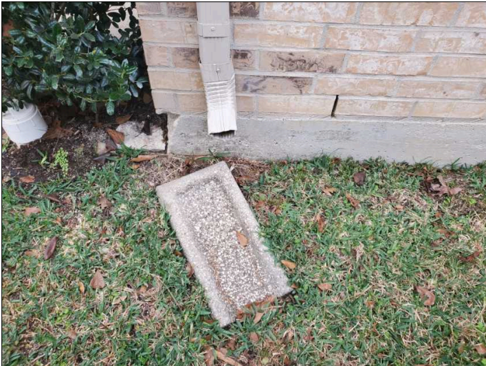
Damaged and bent gutters.
