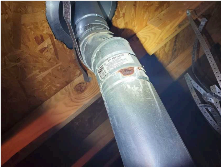
Rusted flue present. If rusting continues, it will allow combustion gasses such as carbon monoxide into the home.
