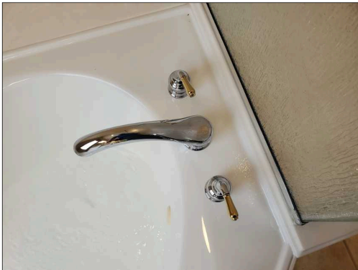
2 handle tub present without a temperature regulating mixing valve present / found. This allows for a max temperature to be preset to avoid scolding.
