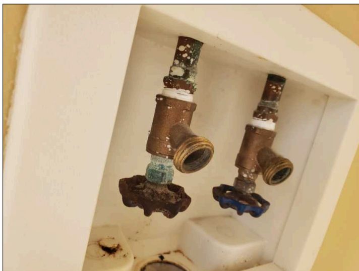
Corrosion present on washing machine valves. Leaking possible.
