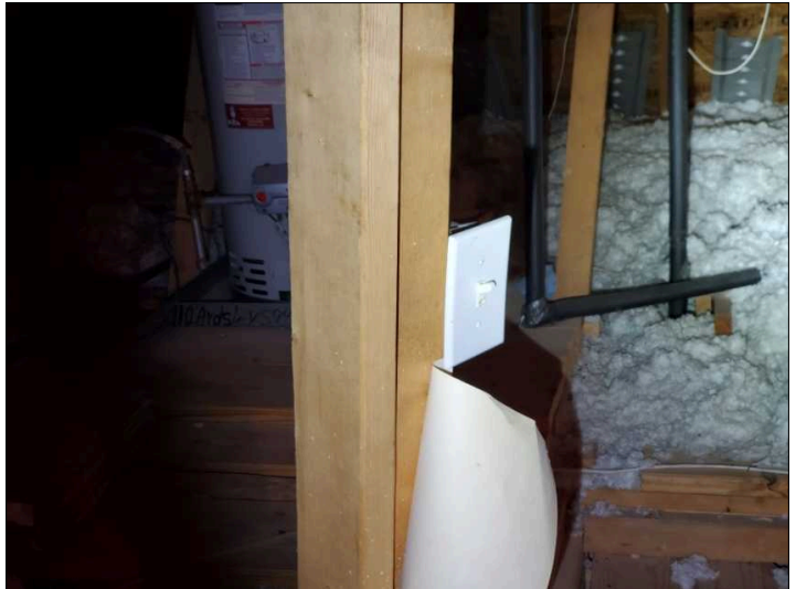
No marked service disconnect could be found at air handler unit.
