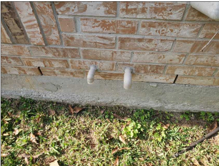
Water heater vent and drain lines. If water is seen coming from here, contact plumber for evaluation.
