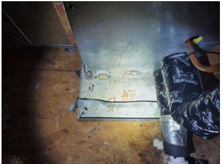
Light rust in condenser pan. Heavy rust may cause pan to leak. Recommend replacement or evaluation over time.
