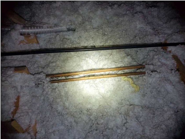
Piping materials present:Copper
