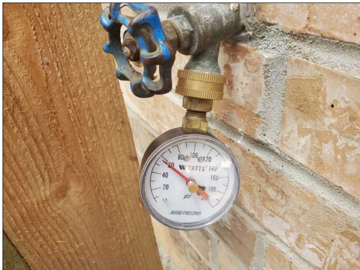
Static Water Pressure Reading: 60 psi
