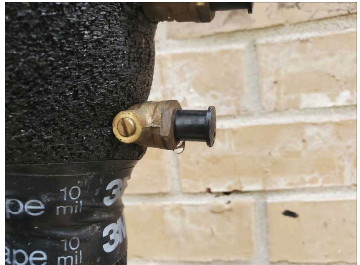
Backflow preventor is leaking.
