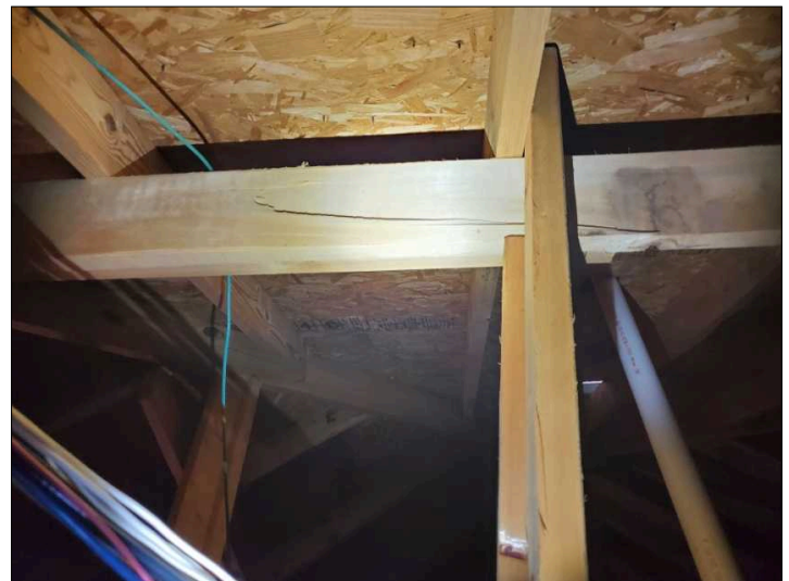
Split/Broken framing boards observed.
