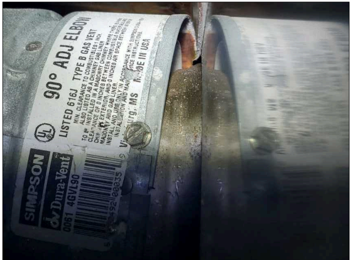
Rusted flue present. If rusting continues, it will allow combustion gasses such as carbon monoxide into the home.
