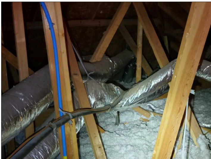
Flexible ducting present. Flex ducting performs best with long bends and full suspension from ceiling.
