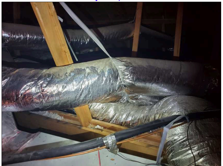
Flex ducting in direct contact with flex ducting. Possible condensation location. Moisture and microbial growth possible in these areas. Recommend spacing ducting so that not in contact with each other.
