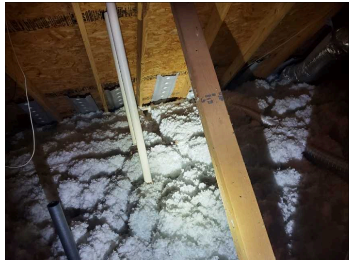
Signs of either past or present rodent activity. Feces, urine, tunneling and / or bedding noted in attic.
