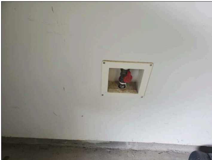
Water shutoff location.
