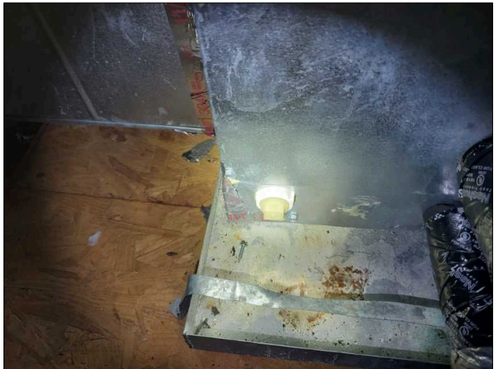
No secondary drain installed. This should drain into a catch pan if the primary is clogged.
