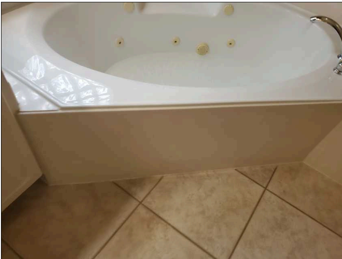
No access panel to pumps or receptacle.
