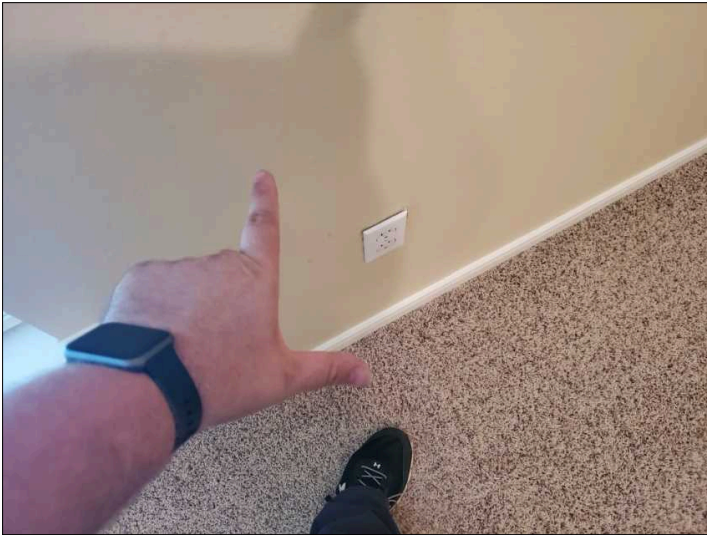
Loose receptacle found.
