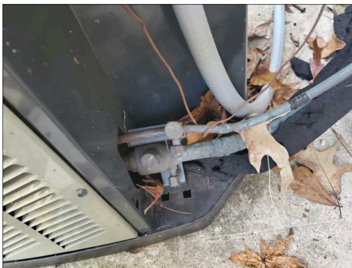
Missing locking refrigerant caps. These caps prevent tampering and possible chemical abuse.
