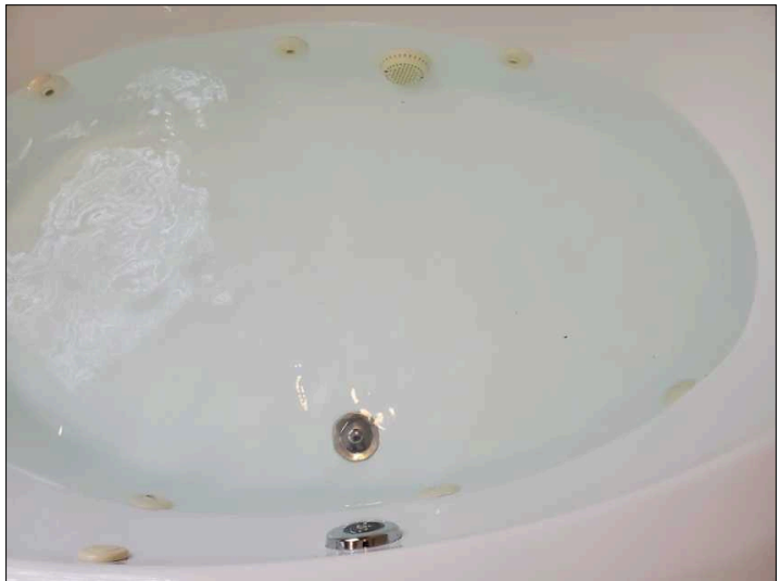
Heavy debris from inside hydro therapy tub. Suggest deep cleaning prior to use.
