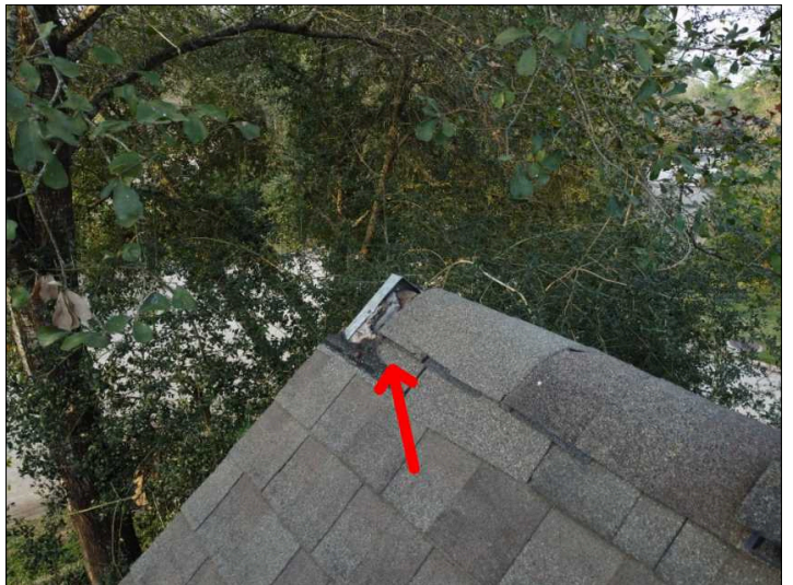
Shingles are missing / torn
