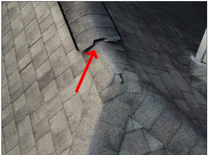
Shingles are missing / torn
