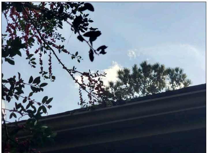
Tree in contact with roof. Should remain clear to prevent damage.
