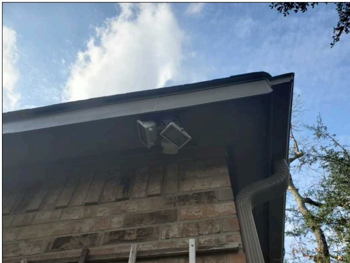
Some lights / switches did not function at time of inspection.
