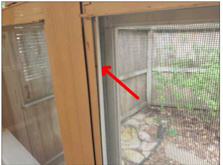
Some windows trims in need of weather proofing (caulk).
