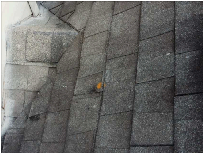
Rust staining present.
