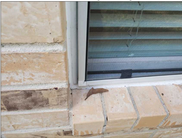
Missing / damaged screens noted.
