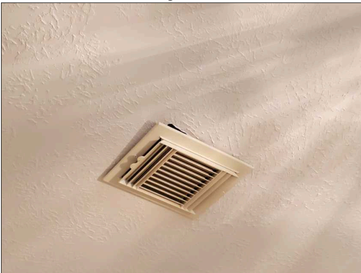
Registers are loose
