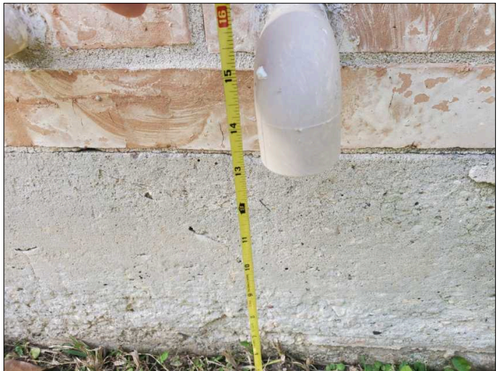
Temperature and pressure valve does not have proper discharge line. This min. 3/4" cpvc line should exit attic space and discharge *within 6" of the ground outside.*
