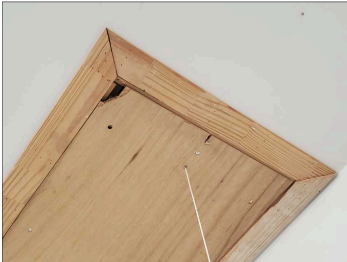
Attic ladder has loose or damaged hardware. Suggest repairs prior to using access ladder.
