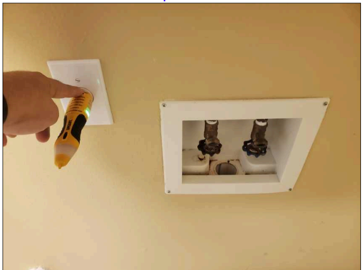
All receptacles near "wet" locations should be GFCI protected. This includes bathrooms, kitchen counter area, outside receptacles, garage and utility areas.
