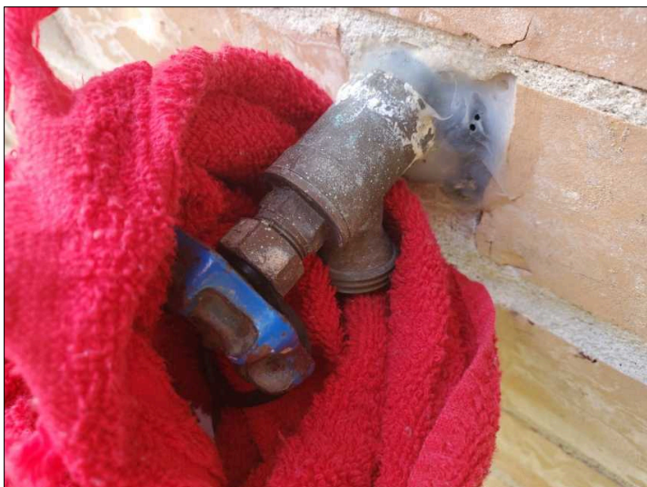
Backflow preventer not present on exterior hose bib. This will prevent contaminants from flowing back into the potable water system.
