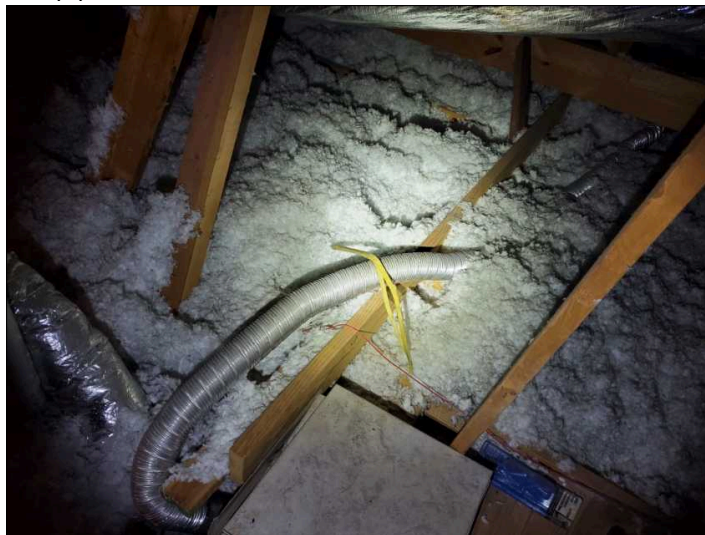
The vent pipe from the exhaust fan terminates and is pointed at the attic roof ridge vent/soffit vent/gable vent. This is less efficient and can cause a buildup of moisture and eventually mold in the attic. Recommend upgrading to properly route vent(s) to the exterior of the home.
