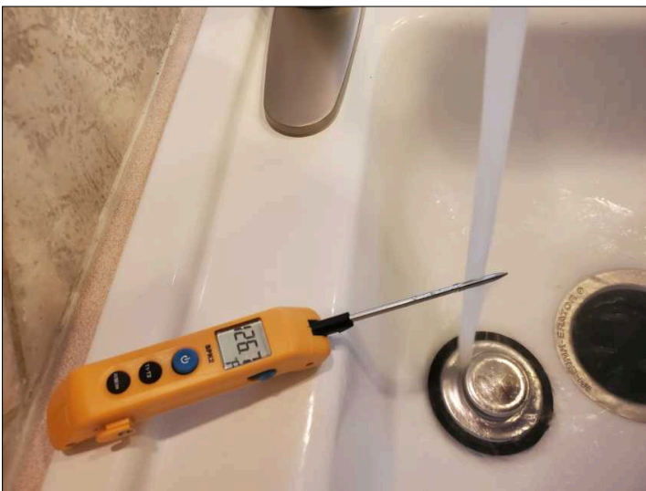
Water heater is set to [125F]. This is high, may scold and be less energy efficient as the normal 120F setting. High temp setting may also indicate a failing water heater or needs the sediment removed.
