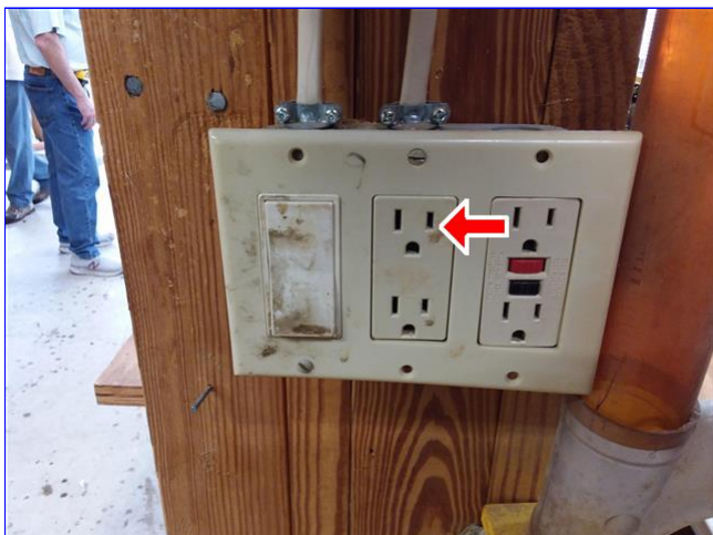
B. Item 8(Picture) missing GFCI in garage
