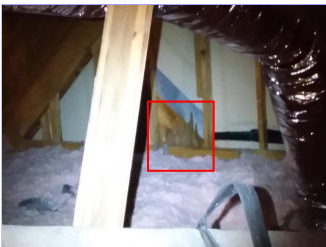
D. Item 2(Picture) evidence of former beehive in attic
