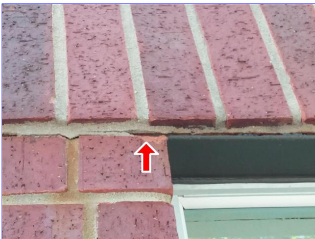
E. Item 2(Picture) window lintel rust
