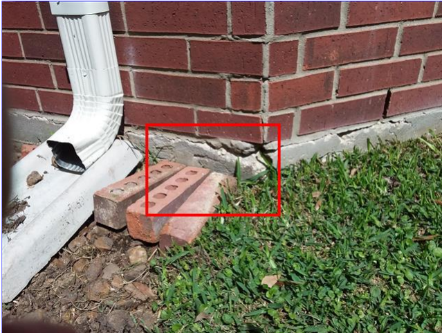
A. Item 6(Picture) foundation flaking back right
