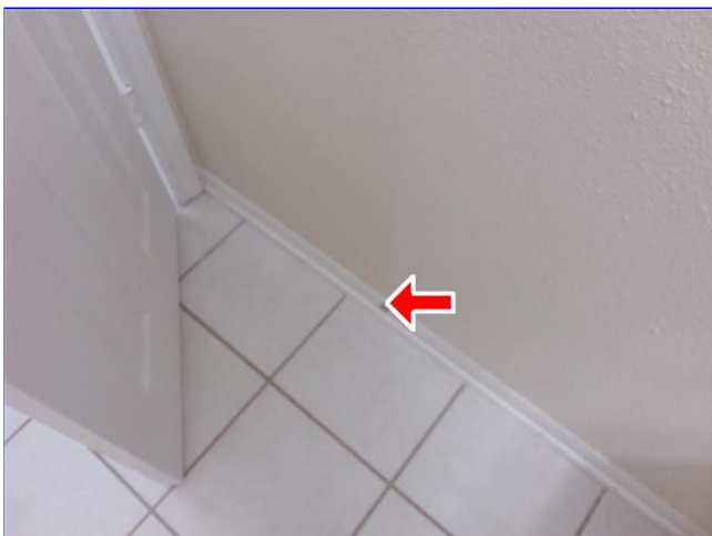
G. Item 3(Picture) doorstops missing in areas
