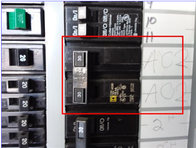
B. Item 3(Picture) Square D breaker in cutler hammer box
