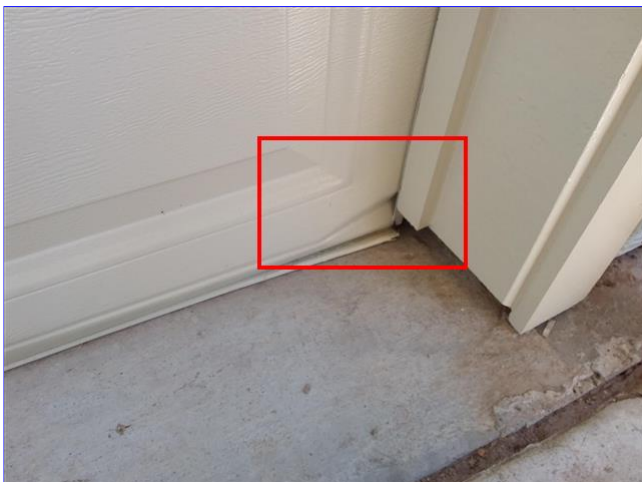
G. Item 1(Picture) right garage door warped
