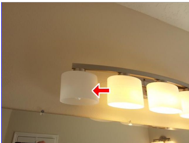
B. Item 13(Picture) master bathroom light out
