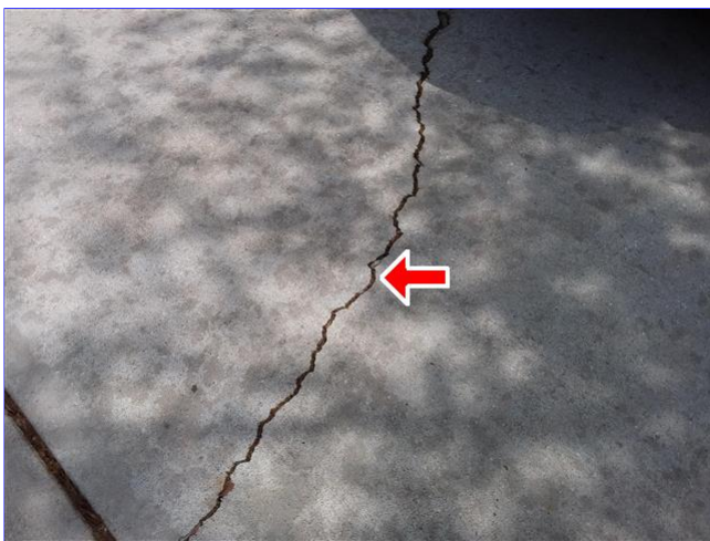
L. Item 1(Picture) settlement cracks in driveway
