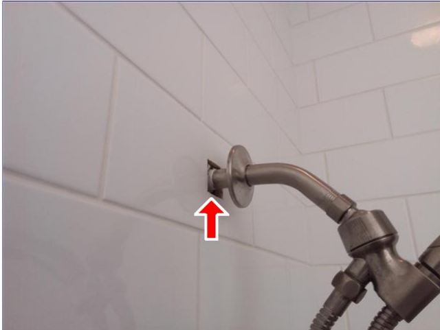
E. Item 5(Picture) master bathroom shower head not sealed to wall
