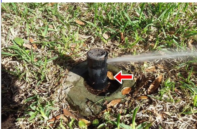
A. Item 2(Picture) slight leak at sprinkler head Repaired
