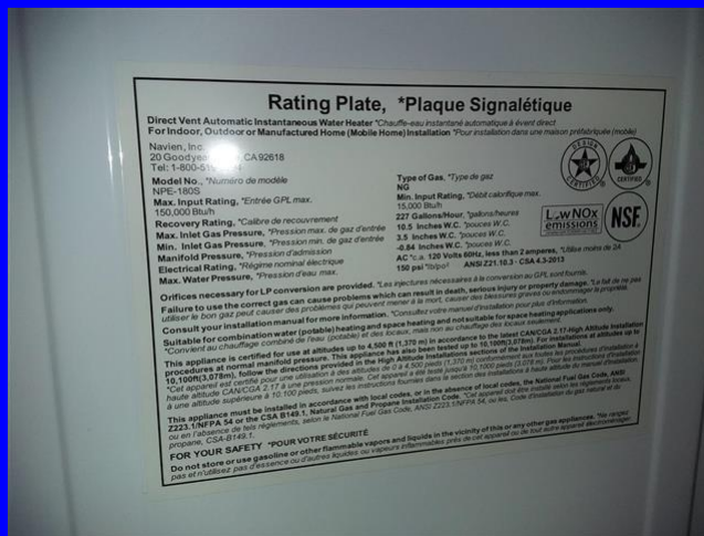
water heater label
