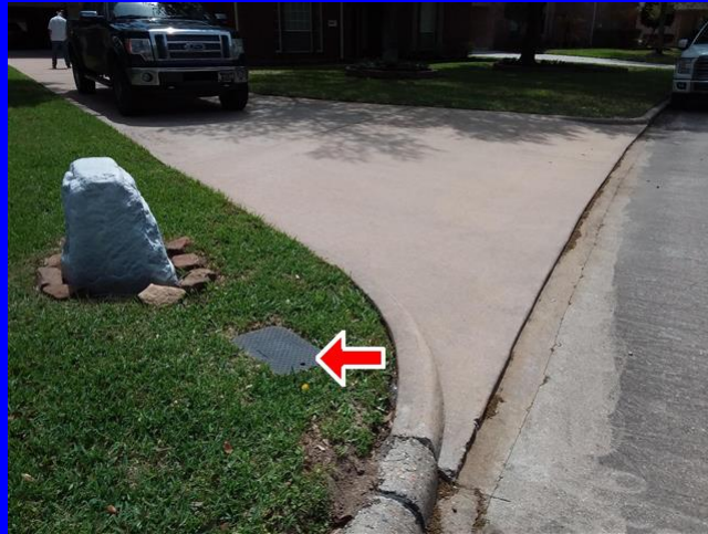
water meter location
