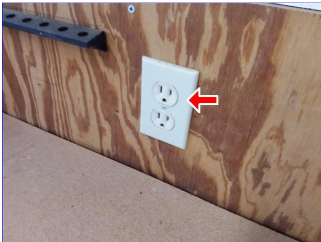
B. Item 9(Picture) loose outlets in areae
