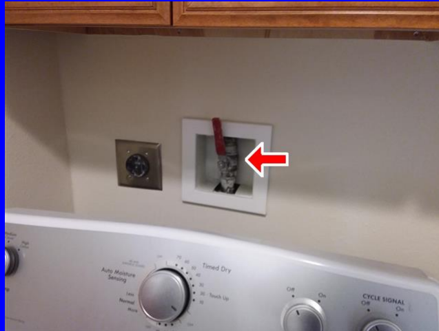
main water supply laundry room
