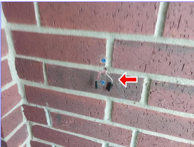
B. Item 1(Picture) doorbell missing
