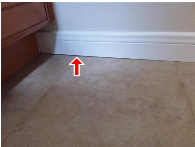
E. Item 3(Picture) baseboard separation and master bathroom
