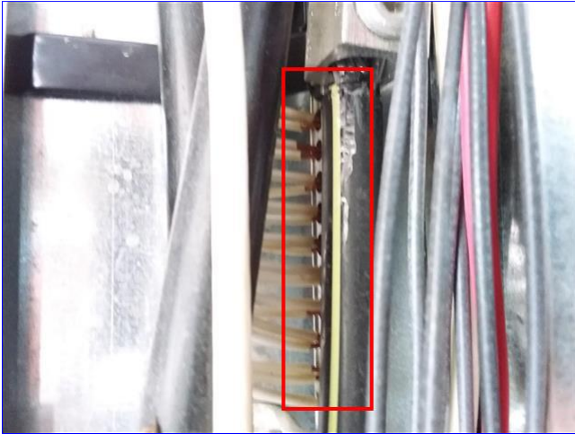
B. Item 4(Picture) double lugged neutrals in main panel
