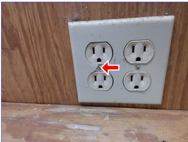
B. Item 10(Picture) damaged cover in garage
