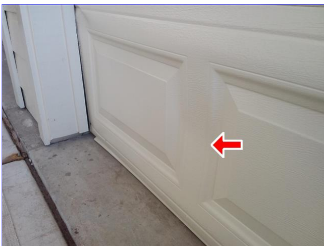
G. Item 2(Picture) right garage door warped
