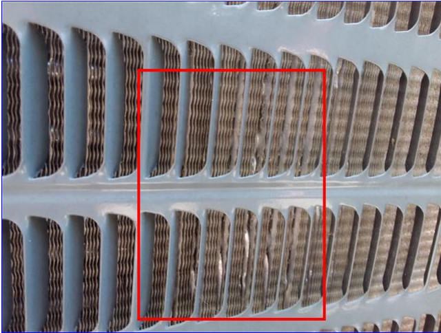
B. Item 12(Picture) unit 2 coil damage
