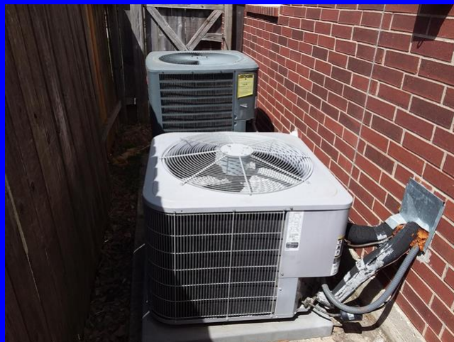
condenser units for home right side
