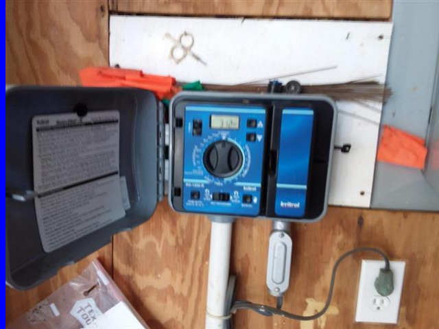
irrigation control in garage
