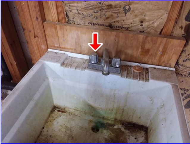
A. Item 1(Picture) no hot water supply and continuous drip in garage
