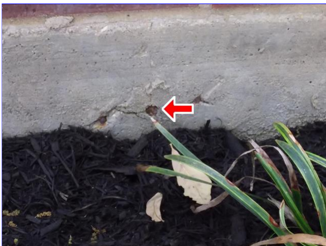
A. Item 4(Picture) exposed to cable front of home
