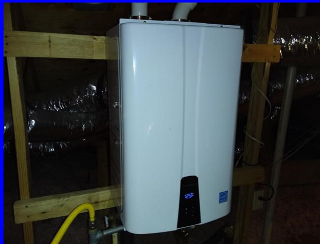
tankless water heater in attic
