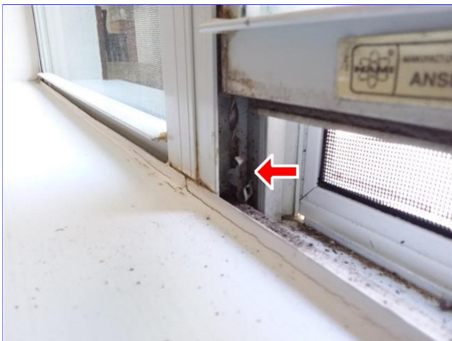
H. Item 3(Picture) spring loose in living room window
