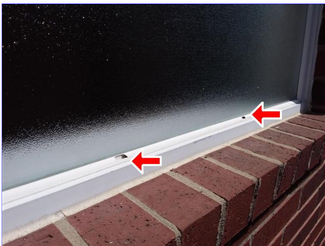
H. Item 1(Picture) cracked glazing strip master bathroom exterior
