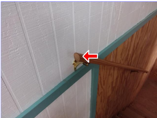
I. Item 2(Picture) corner piece missing
