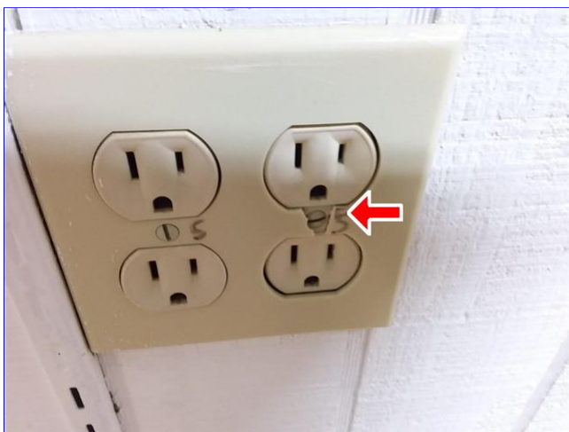
B. Item 11(Picture) damaged cover second floor garage outlet
