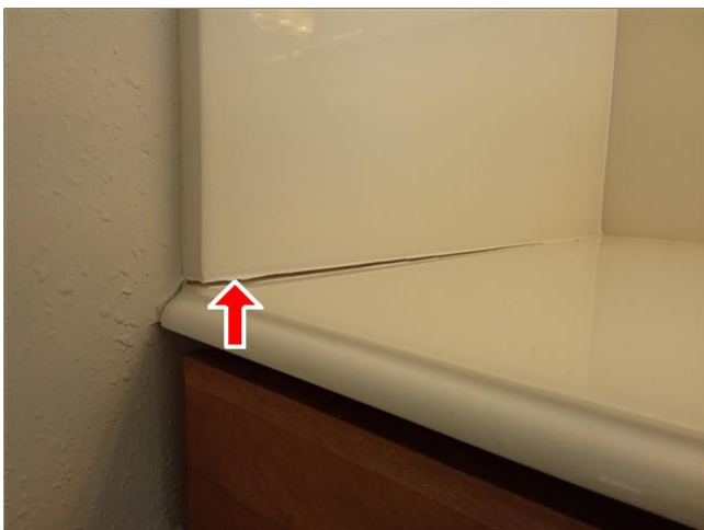
E. Item 4(Picture) missing sealant master bathroom counter
