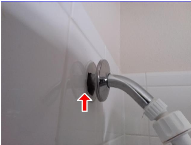
E. Item 6(Picture) guest bathroom one shower had not sealed
