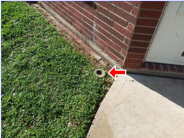
A. Item 1(Picture) sprinkler head not in use in backyard Functioning normally
