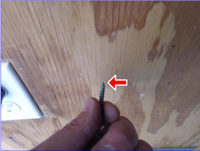
A. Item 3(Picture) improper panel screw
