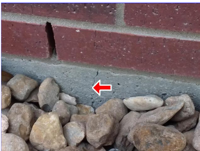
A. Item 5(Picture) slight crack left side
