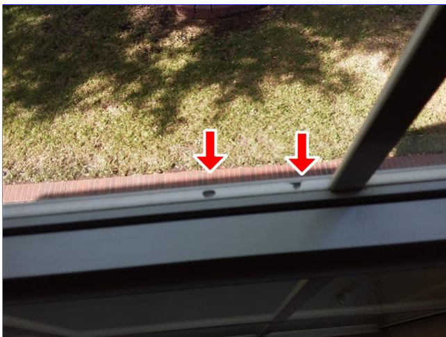
H. Item 2(Picture) glazing strip damage second floor living room window
