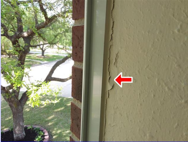
E. Item 7(Picture) drywall cracking second floor living room window
