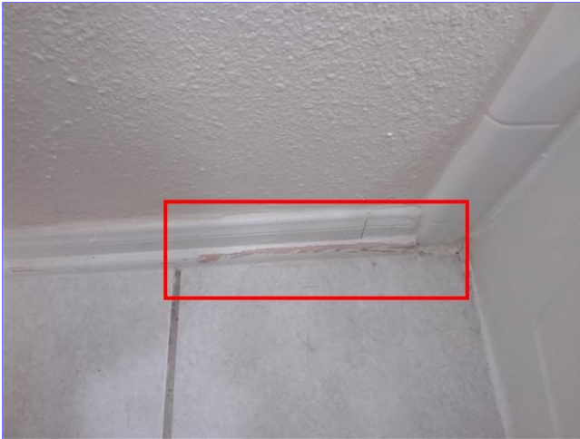
E. Item 8(Picture) guest bathroom baseboard trim peeling
