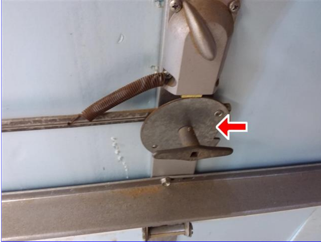
G. Item 1(Picture) garage lock not disabled
