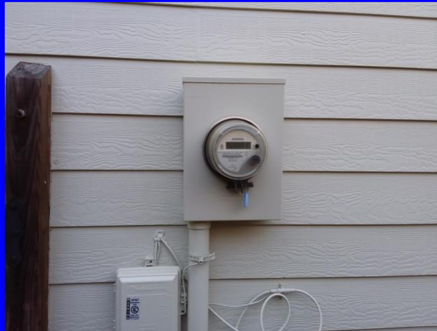
electrical meter left of garage underground service
