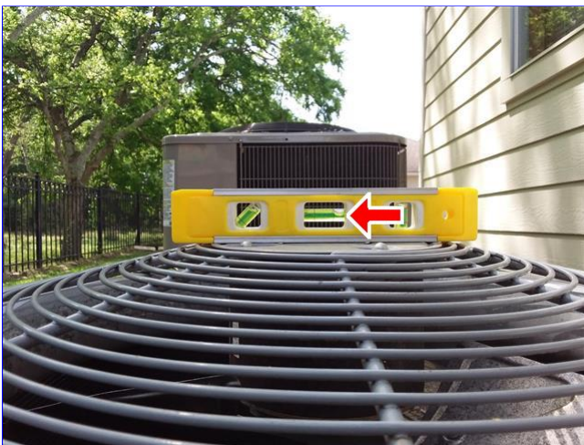
B. Item 11(Picture) garage unit 2 not level Has been leveled
