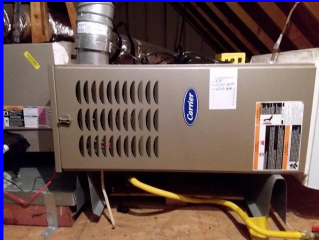
gas furnace unit 1
