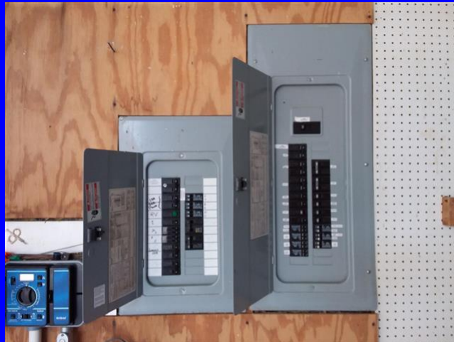
200 amp panel and 100amps of panel in garage
