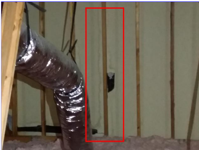
D. Item 1(Picture) evidence of previous leak in attic
