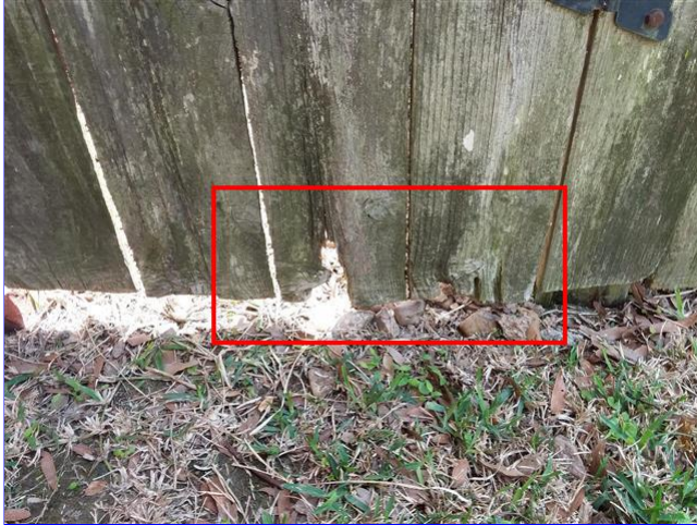
L. Item 2(Picture) fence deterioration in areas
