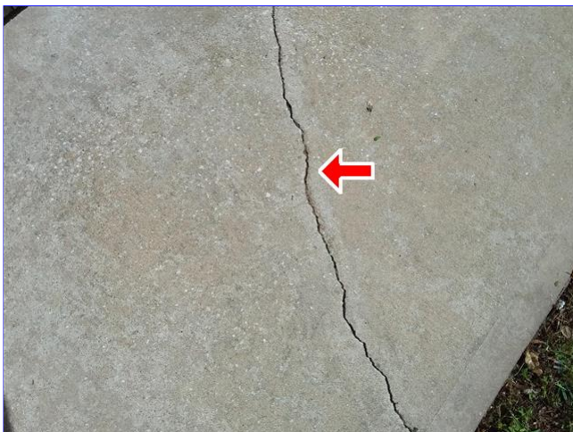
K. Item 1(Picture) cracked back patio
