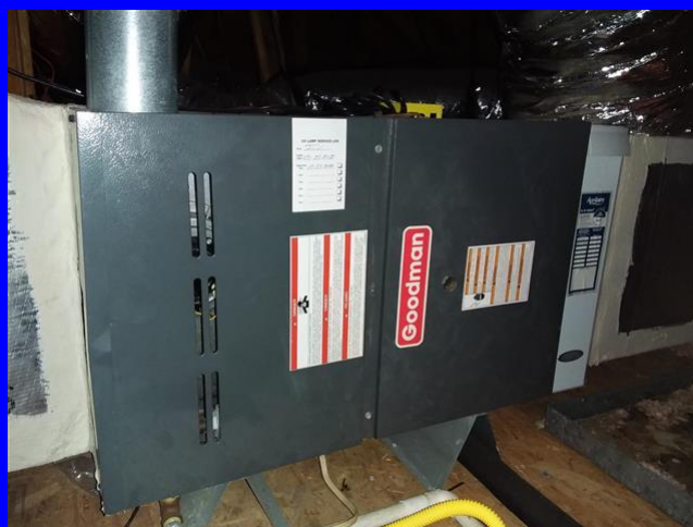
gas furnace unit 2
