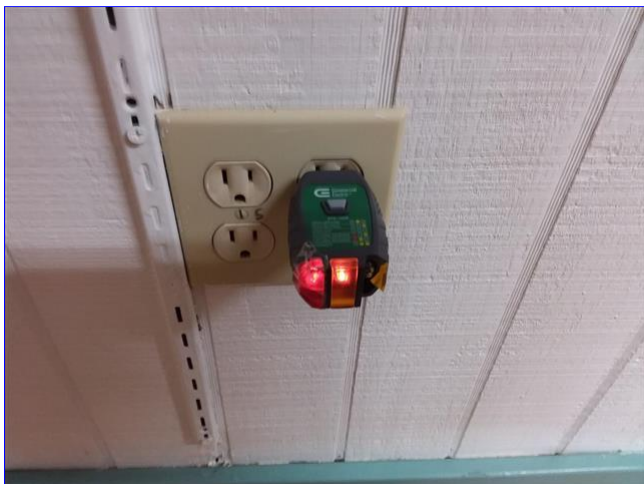
B. Item 12(Picture) reversed polarity second floor garage outlet
