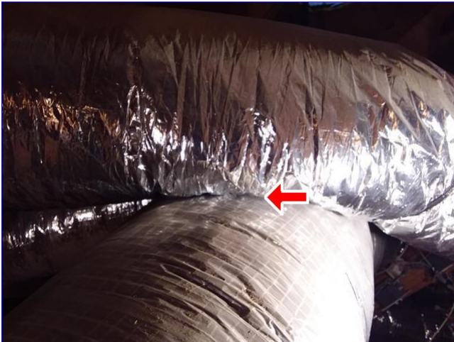
C. Item 1(Picture) duct contact in attic
