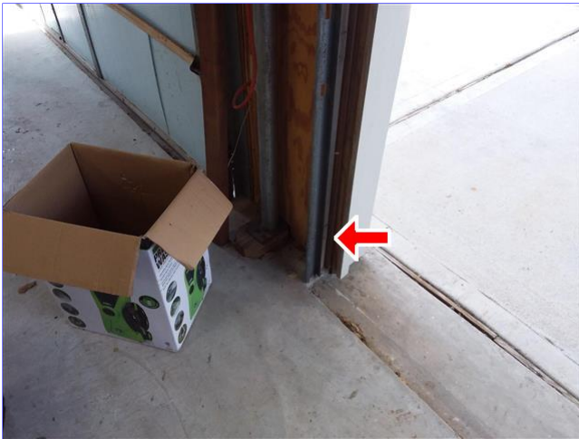
G. Item 2(Picture) door sensors missing
