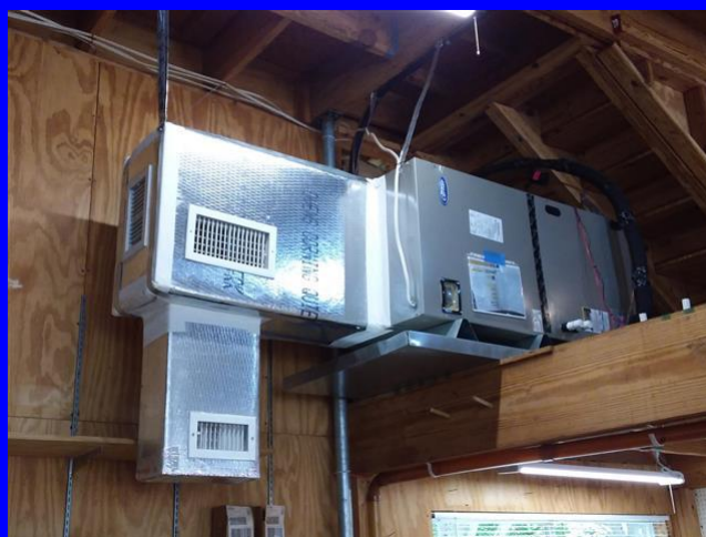
unit 1 furnace in garage
