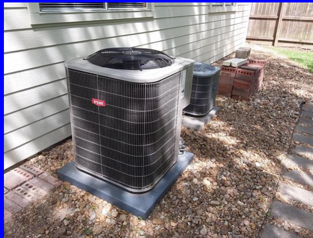
condenser units behind garage
