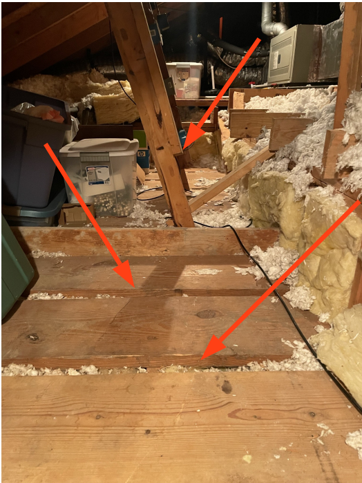
Improper access to appliances in the attic
