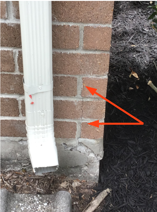
Cracks in the brick veneer
