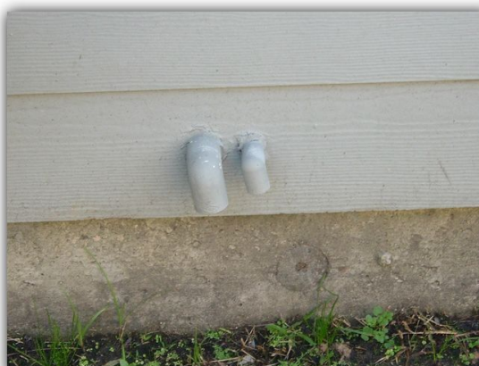
The water heater performing as intended at time of the inspection.
