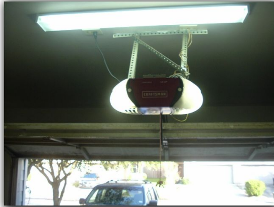
The garage door operator performing as intended at time of the inspection.
