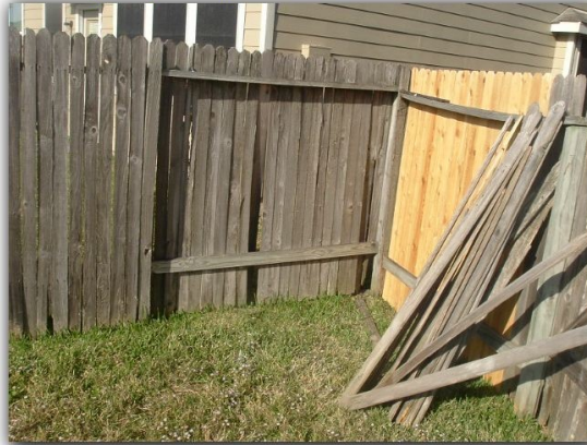
There are damage/decayed/loose pickets.
