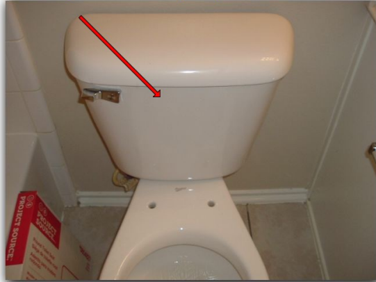
The second floor guest toilet flush assembly is noisy.
