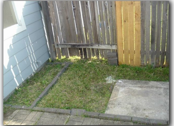
There are damage/decayed/loose pickets.
