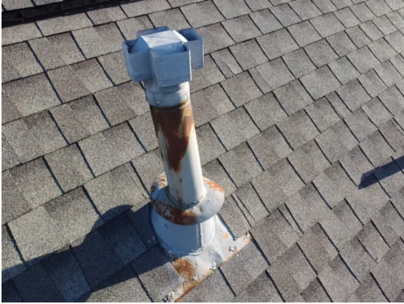
Some surface rust
