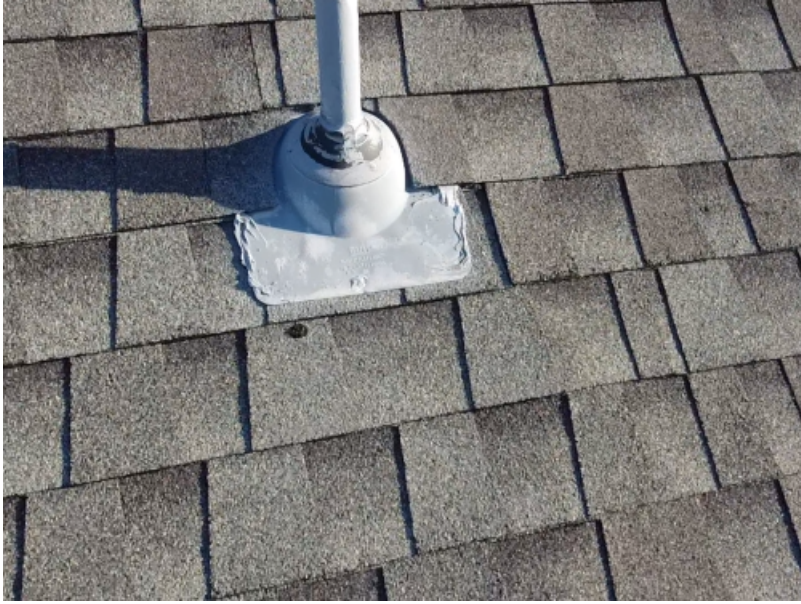
Closest penetration is well sealed and installed.
