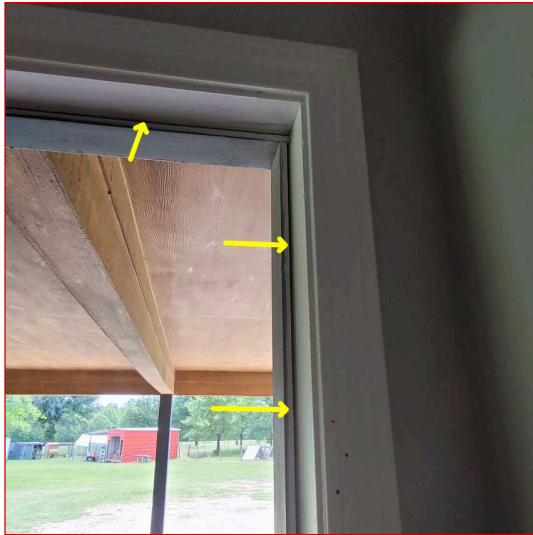
Weather stripping needed.
