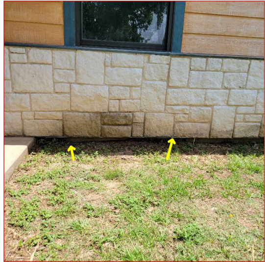
Earth to siding contact was observed on the exterior siding and should be a minimum of {4"} clearance from the ground for brick/stone {6"} for wood and {8"} for stucco. Common in older homes.
