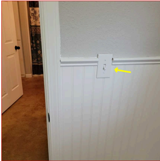
Light switch installed upside down.
