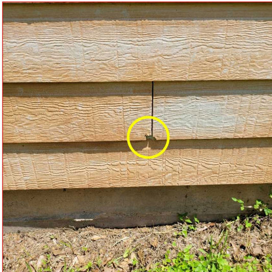
Damaged or missing board(s)noticed.
