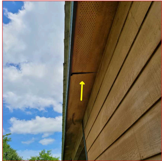
Soffits are sagging and or pulling apart in area or areas around the home.
