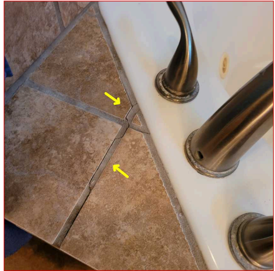
Missing and or damaged grout was observed in the shower area and should be corrected to avoid future water leakage.
