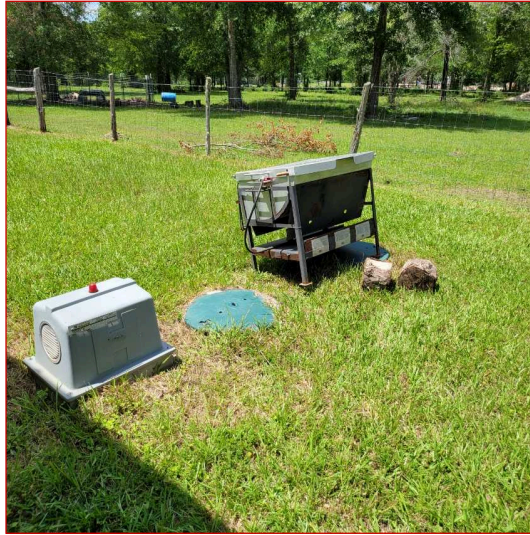
Aerobic septic system noted.
