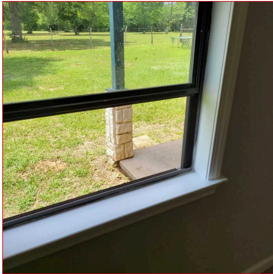
Window screens were observed to be damaged or missing.
