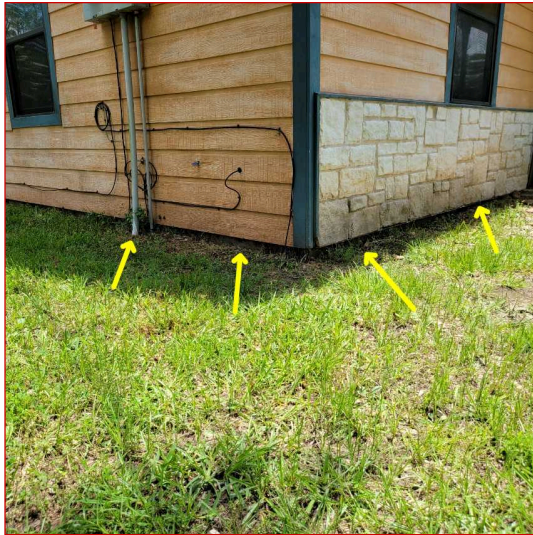
Earth to siding contact was observed on the exterior siding and should be a minimum of {4"} clearance from the ground for brick/stone {6"} for wood and {8"} for stucco. Common in older homes.
