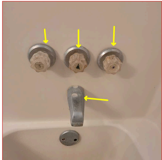
Faucets are out dated and need replaced.
