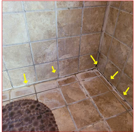
Shower or tub area needs caulking.
