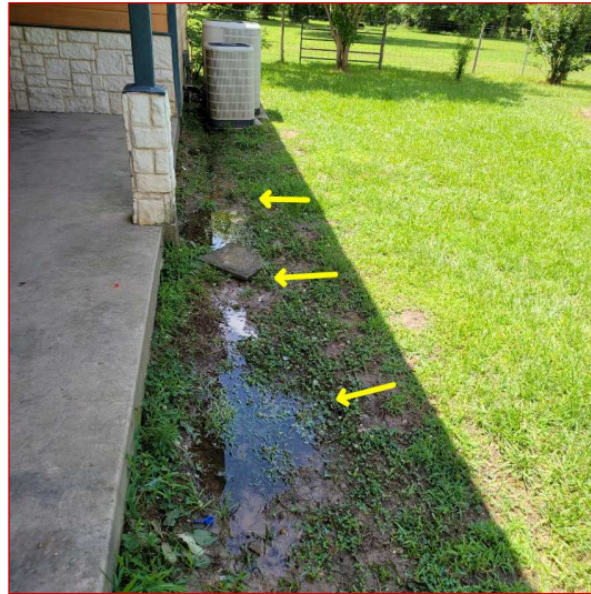
Ponding water was observed at one or more areas around the structure.
