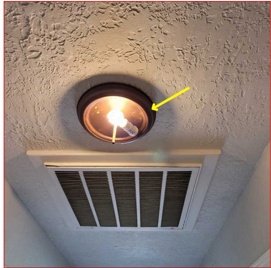
Light cover(s) missing.
