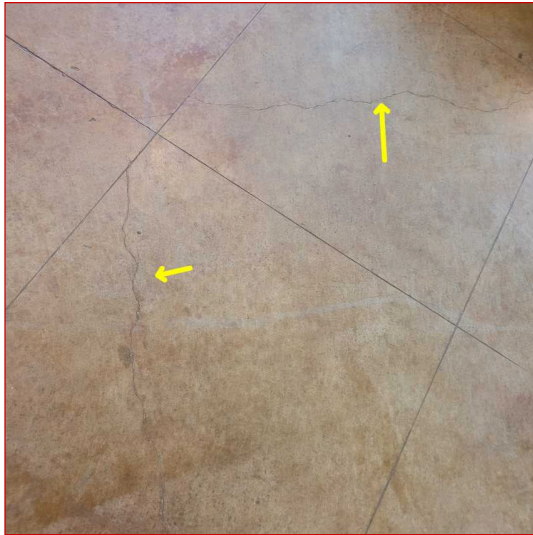
Floor cracks noted in multiple areas.
