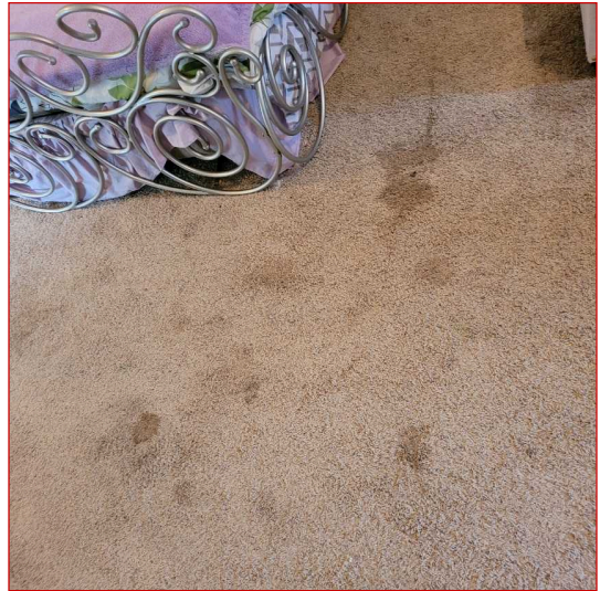
Carpet is stained in multiple areas.
