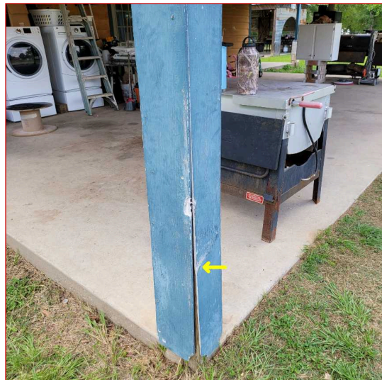
Boards need replaced in multiple locations.
