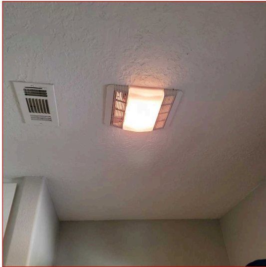
Guest bathroom fan.
