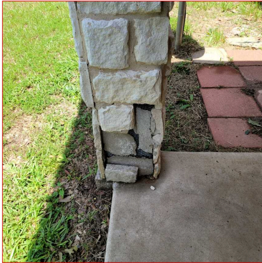
The exterior stone has some deterioration and/or damage.
