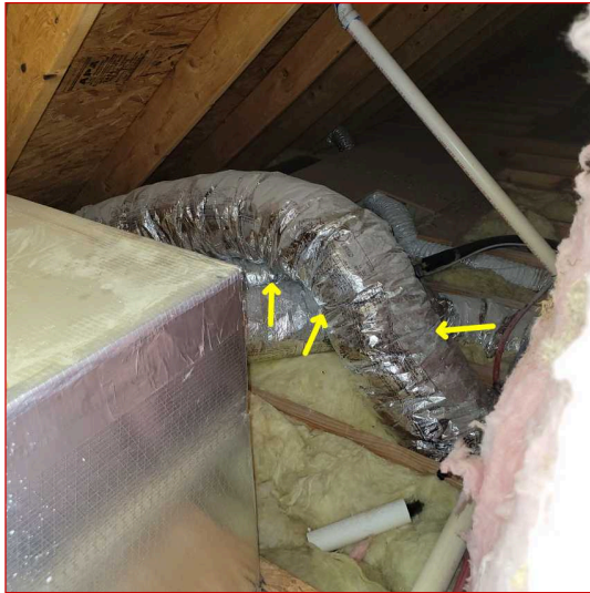
Ductwork should not be touching.
