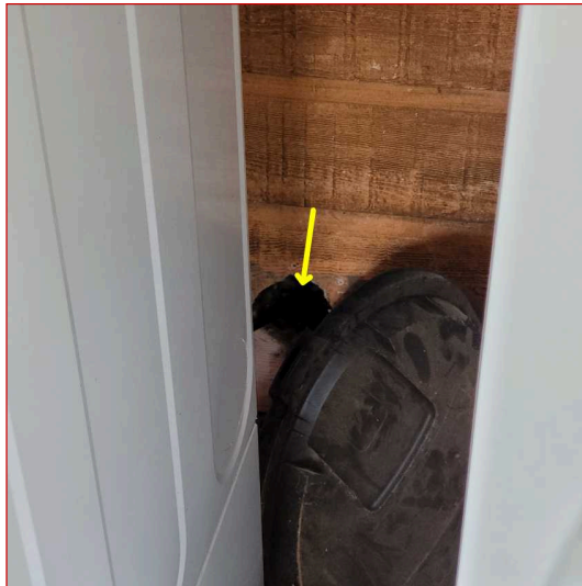
The dryer vent has either a damaged and/or missing exterior cover.
