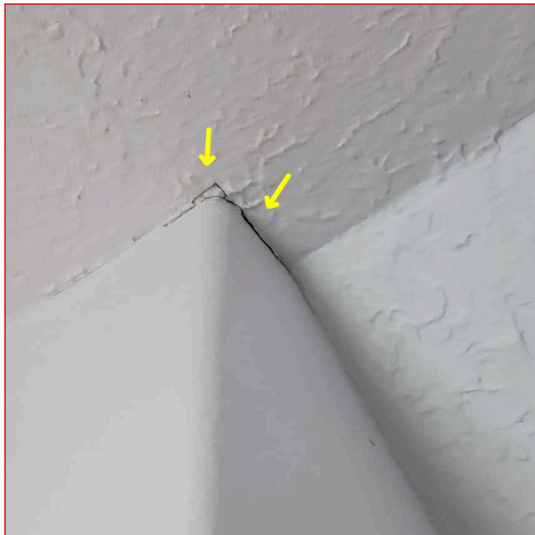
Crack(s) noted at one or more areas around the home.
