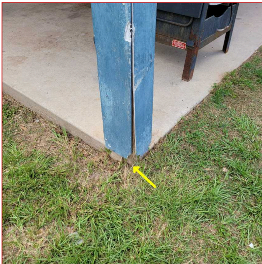
Wood to ground contact.
