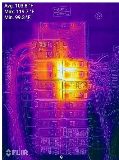
General Photos of 220V Outlets:
