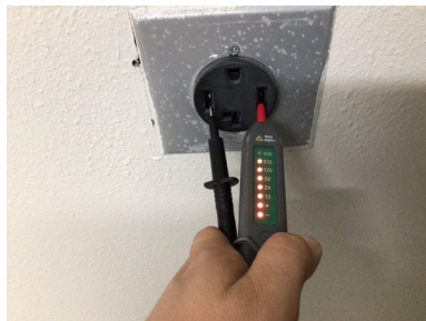
General Photos of Grounding Systems:
