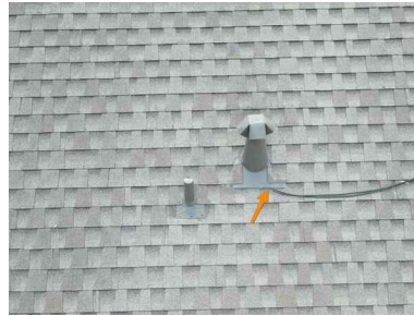
Cable Through Flashing
