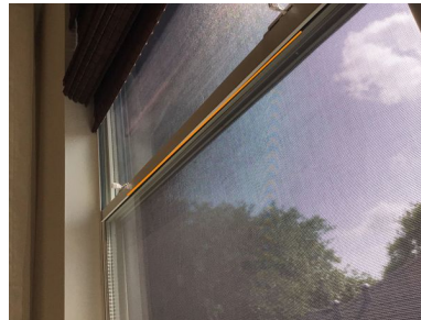
Loose from frame, 2nd Floor
