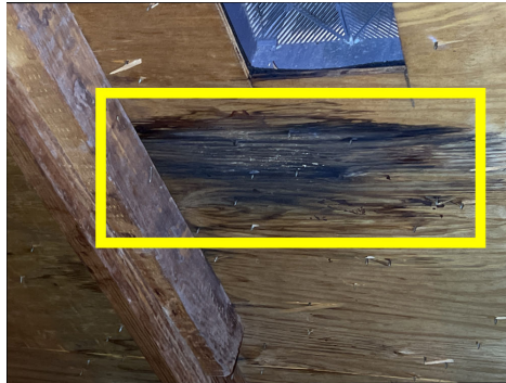
Water stains/wood rot on roof decking
