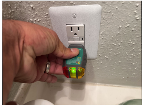
Bath GFCI outlet not working properly
