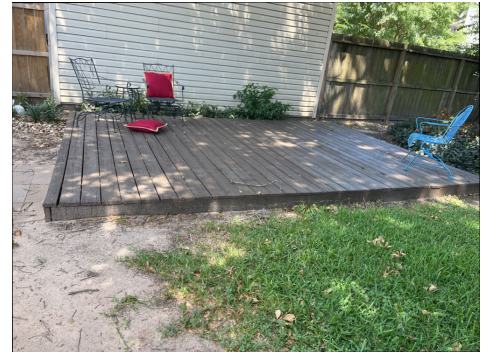
Earth to wood contact at back deck
