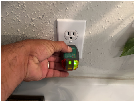
Kitchen outlet not properly GFCI protected
