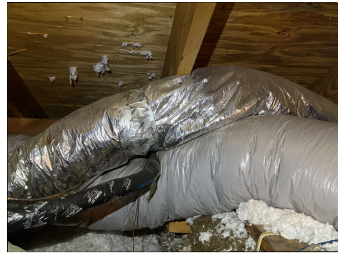
AC flex duct touching
