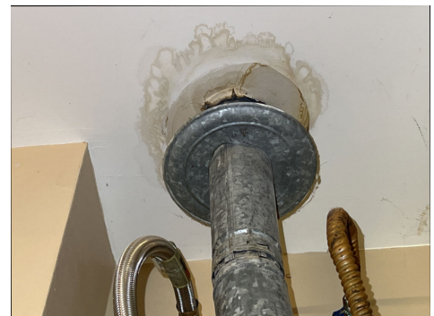
Vent collar not properly secured to ceiling
