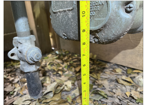
Gas meter lower than 10" from ground
