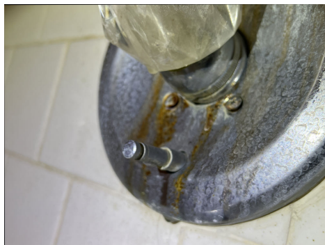
Bath faucet leaks at base
