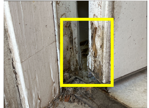
Wood rot on door/door frame
