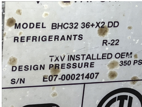
Evaporator Coil: 2007 Aspen 3 Ton
