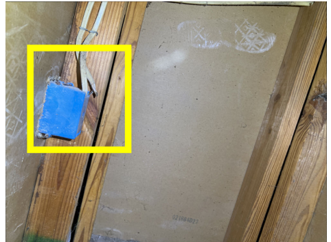
120 V wire located in return air chase
