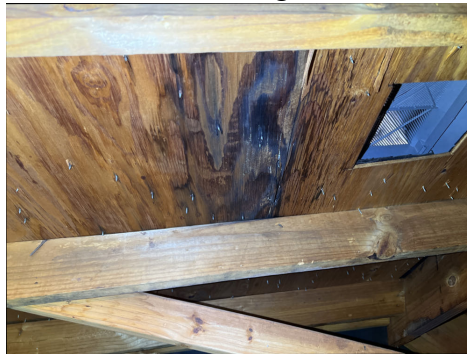
Water, stains/wood rot on roof decking
