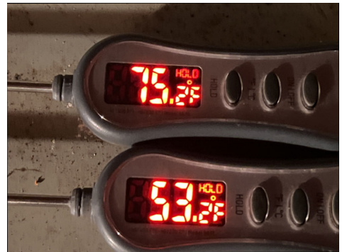
Evaporator coil temperature split: 22.0°
