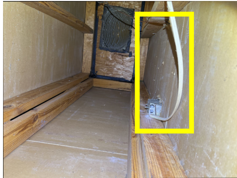
120 V wire located in return air chase
