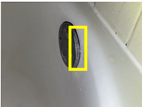
Tub overflow cover is loose
