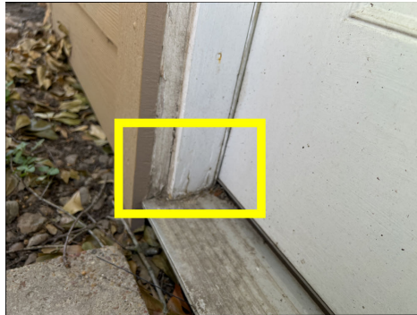
Wood rot on door/door frame
