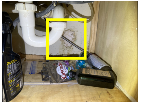
Water stains under kitchen sink Active leak
