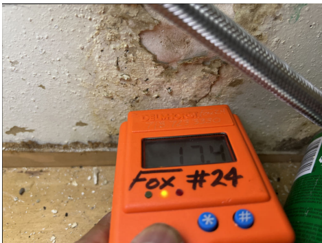
Elevated moisture observed at/below kitchen sink
