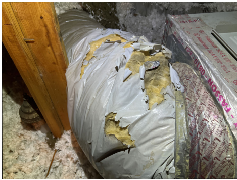
Damaged gray duct
