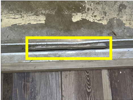
Garage pedestrian door threshold is damaged
