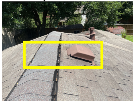
Two types of roof vent used
