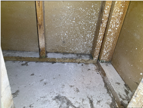
Return air chase not properly sealed
