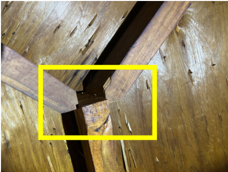
Poor framing cuts to one or more rafters
