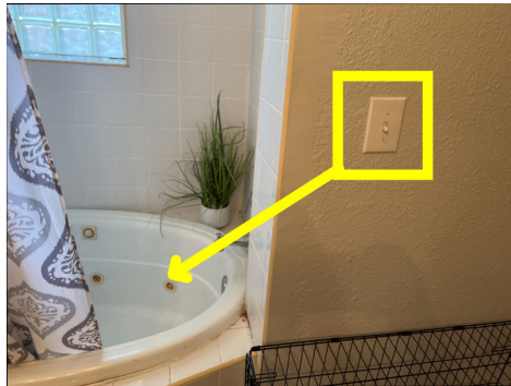
Switch can be operated from bathtub
