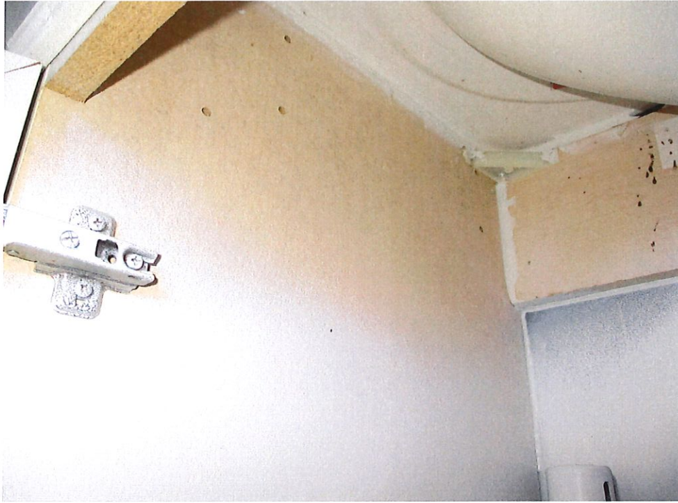
Photo 7 - Mold growth on vanity in guest bathroom.
