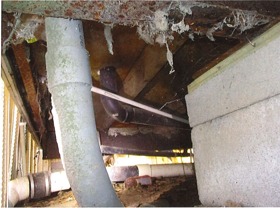
Photo 13 - Mold growth observed throughout the crawlspace on various surfaces.
