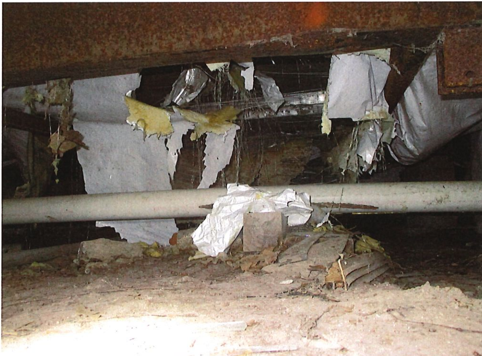
Photo 10 - Excessive moisture damage to the subfloor and insulation in crawlspace.
