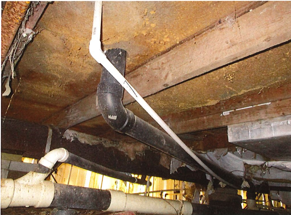
Photo 14 - Mold growth observed throughout the crawlspace on various surfaces.
