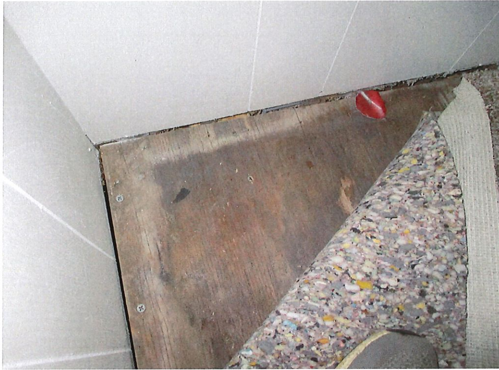
Photo 9 - Mold growth on wood decking under carpet in bedroom 1.
