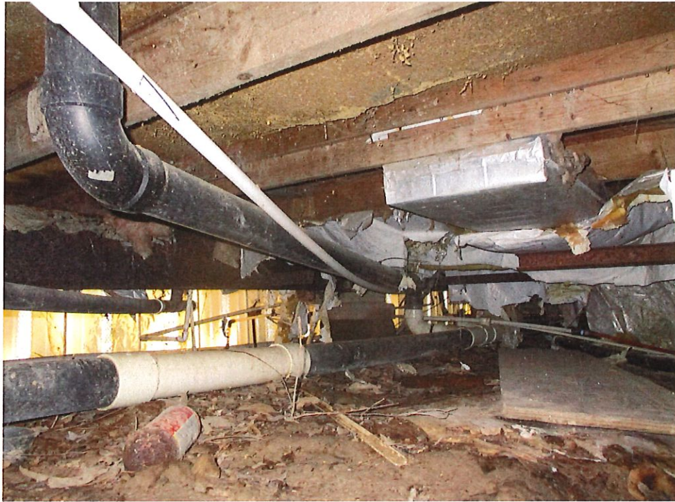
Photo 11 - Excessive moisture damage to the subfloor and insulation in crawlspace.
