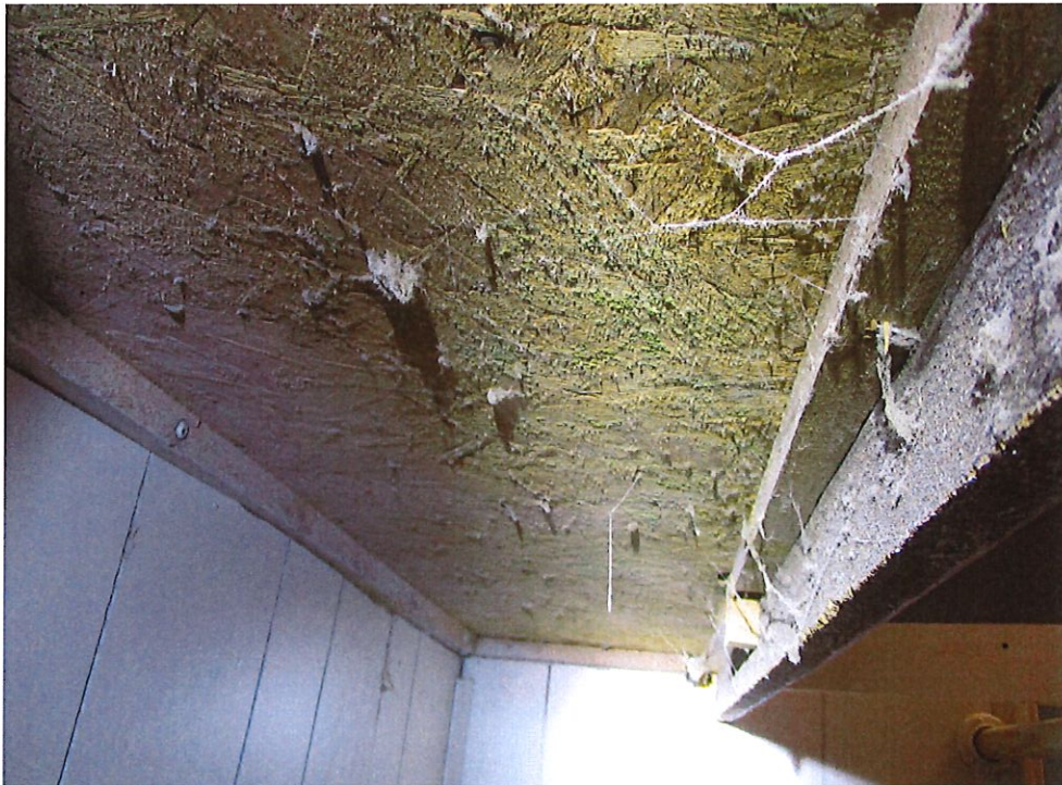
Photo 8 - Mold growth on underside of shelving in laundry room.
