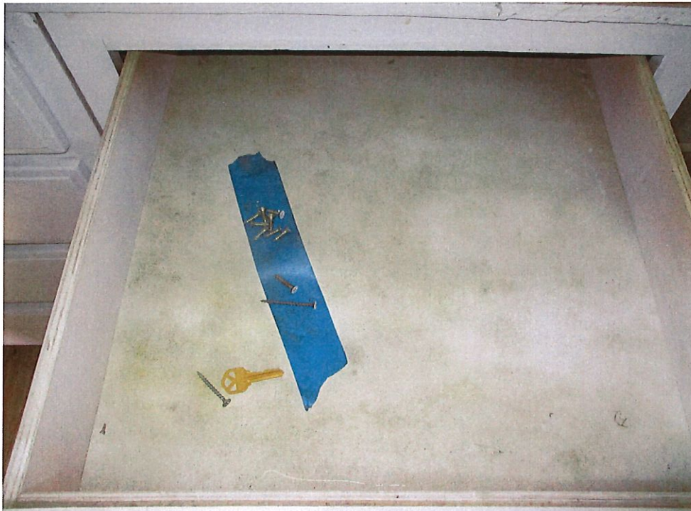
Photo 2 - Mold growth and moisture damage on cabinets and in drawers throughout kitchen.
