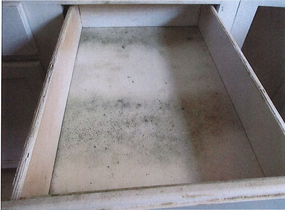
Photo 5 - Mold growth and moisture damage on cabinets and in drawers throughout kitchen.
