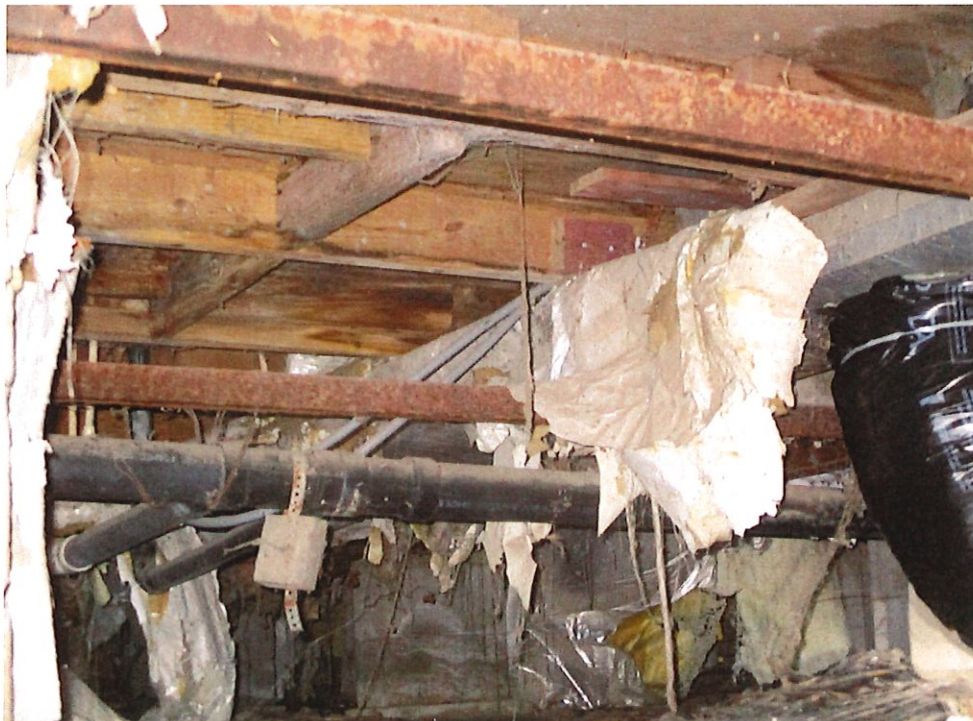
Photo 12 - Excessive moisture damage to the subfloor and insulation in crawlspace.
