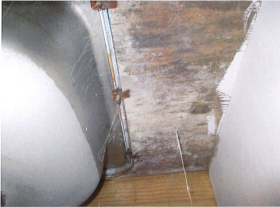
Photo 3 - Mold growth and moisture damage on cabinets and in drawers throughout kitchen.
