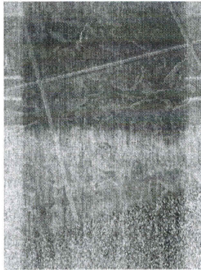
Damaged floor tile.
