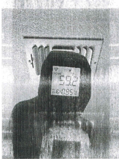
Air temperature measured at supply air vent.
