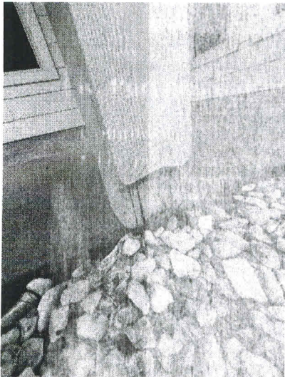
The porch was observed to have one or more loose and/or damaged support columns
