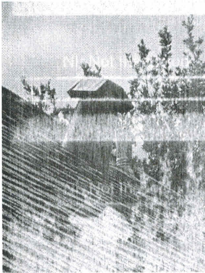
Unapproved roof材 used for dryer vent pipe.
