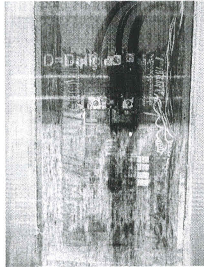
Picture of electrical service panel.
