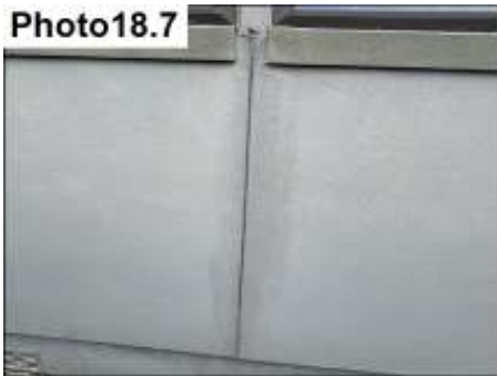
Large cracks are present at the control joints.
