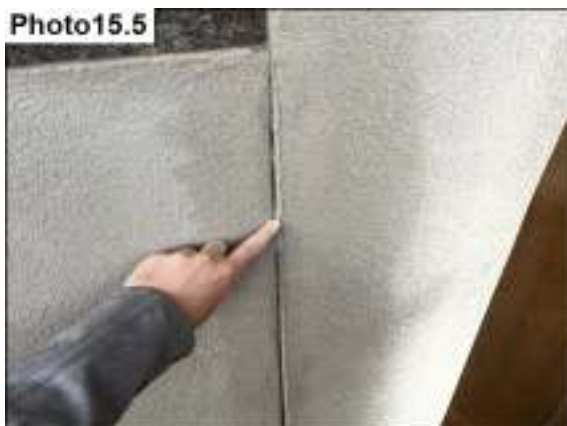
Control joint cracking is present.
