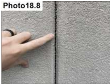
Large cracks are present at the control joints.
