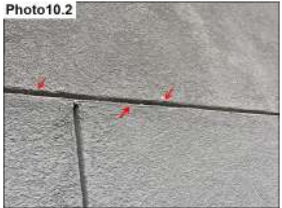
Control joint cracks are present.
