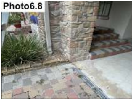
Bottom of wall is in contact with the rocks / flat work.
