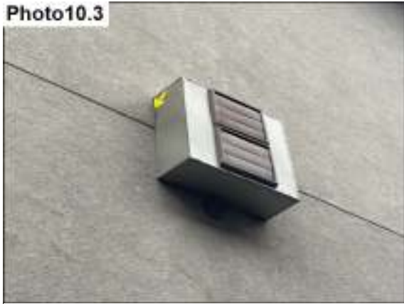
Penetrations lack sealants.
