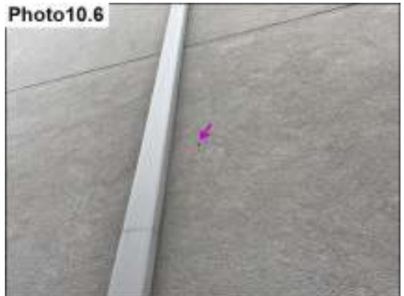
Rust aggregates are present.
