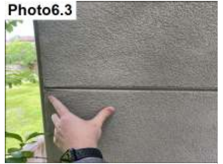
Outside corner cracking is present.
