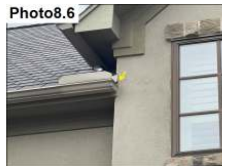
It is suggested to reseal roof flashing & fascia board terminations.
