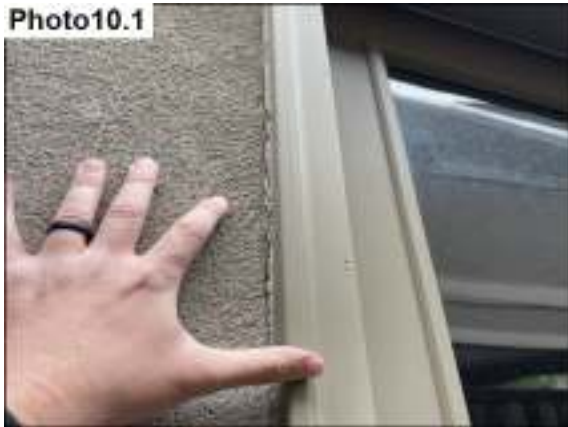
Sealant separation is noted around door frames.
