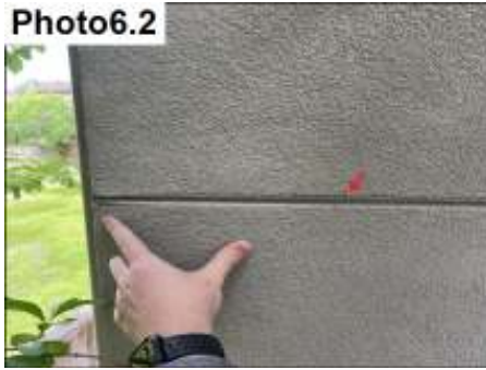
Control joint cracking is present.
