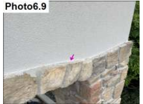
Tops of stone accents lack adequate sealants.
