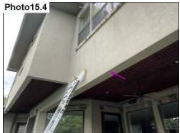
It is suggested to install weep relief at the bottom of the wall.
