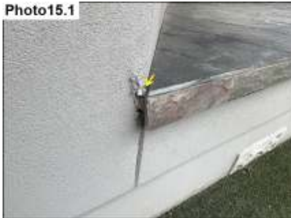
It is suggested to reseal porch flashing terminations.
