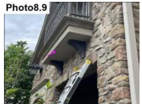
No weep relief is present at the bottom of the walls.
