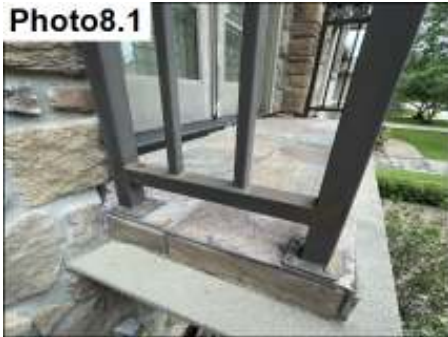
It is suggested to reseal balcony flashings.
