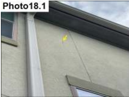
Rust aggregates are present.
