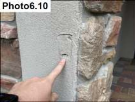
Fastener holes lack sealants.
