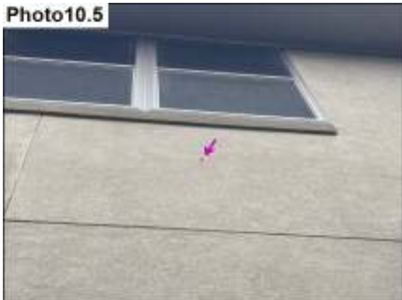
Rust aggregates are present.
