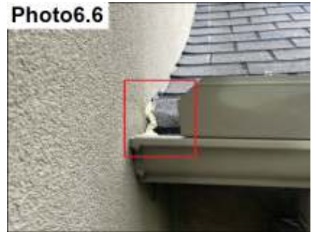
Missing kickout flashing at roof termination.
