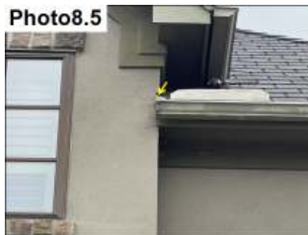
It is suggested to reseal roof flashing & fascia board terminations.
