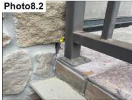
It is suggested to reseal balcony flashings.
