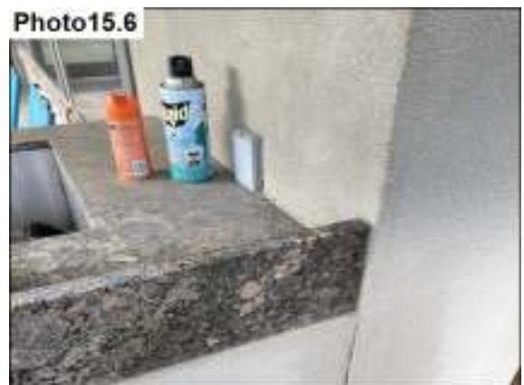
Outdoor kitchen terminations lack sealants.
