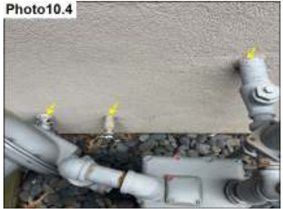
Penetrations lack sealants.
