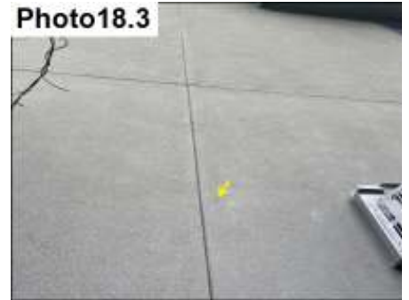
Rust aggregates are present.
