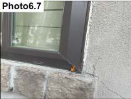
Sealant separation is noted around the window frames.
