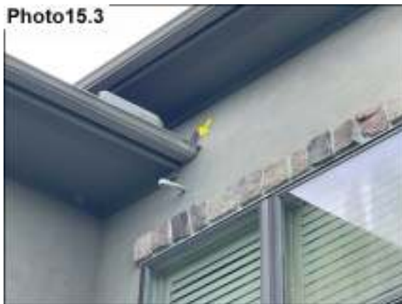
It is suggested to reseal kickout flashing.
