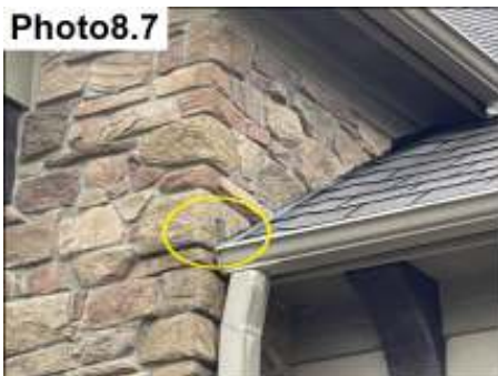
It is suggested to reseal kickout flashing.
