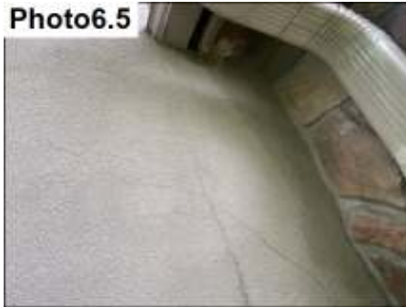
Cracking and staining is present below missing kickout flashing.
