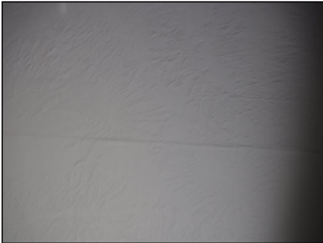
Previous repairs to ceiling did not appear to be of professional contractor quality.
