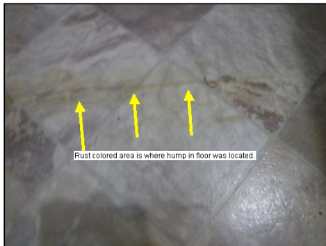
IMPORTANT NOTICE: The flooring in the bathroom was out of level in multiple areas.
