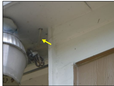
Exposed romex type wiring on exterior of home
