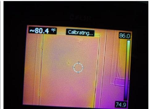
Air leaks noted around doors
