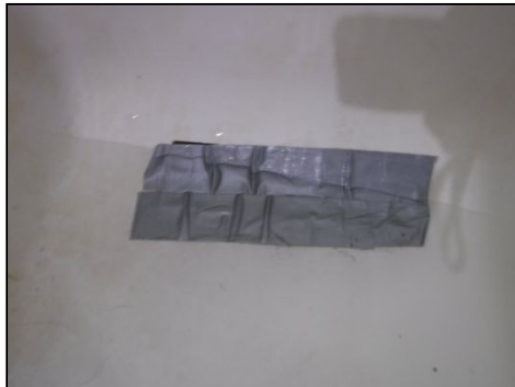
IMPORTANT NOTICE: There was duct tape in the bathtub. Presumably this was covering damage to the tub. Further evaluation and proper repair is recommended.
