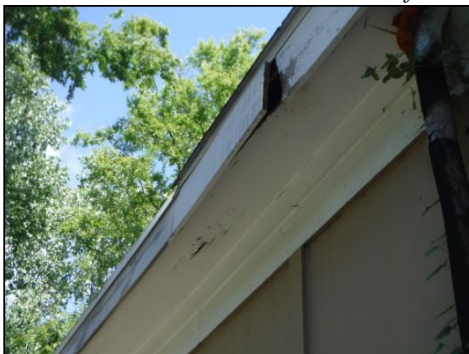
The fascia board has some deterioration on more than one location on the structure
