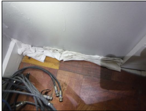
Paper towels stuffed into area where baseboard was missing
