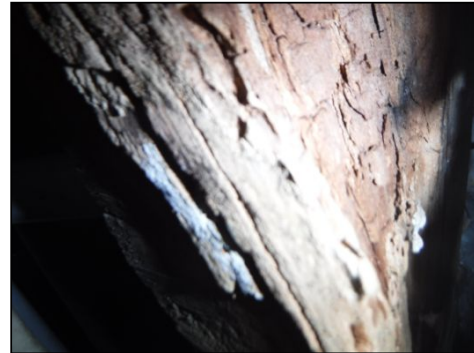
Recommend having pest control specialist review wood damage under unit
