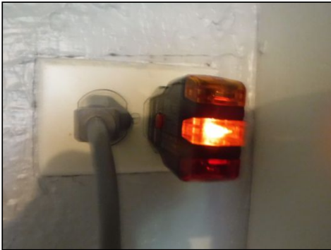
IMPORTANT NOTICE: One or more of the receptacles were noted to have an open ground. Review and repair by a licensed electrician is recommended.
