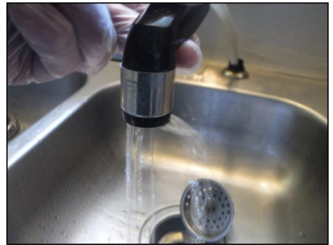
The kitchen sprayer appeared to be clogged..
