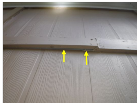
Loose trim boards on siding
