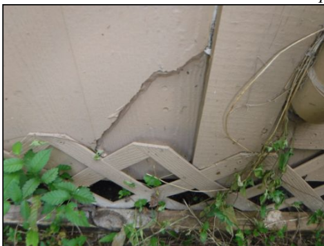
Damaged noted to exterior siding in one or more areas.
