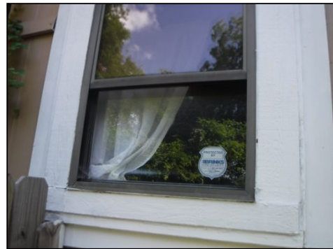
IMPORTANT NOTICE: Missing or damaged screens noted in one or more areas around the home.
