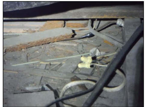
IMPORTANT NOTICE: Two wire to three wire electrical was noted to be connected in the attic space. Further evaluation and repair by a licensed electrician is recommended.
