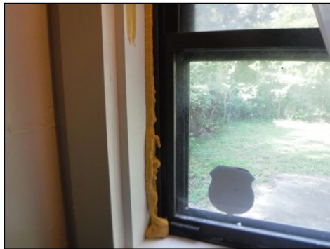
IMPORTANT NOTICE: Spray foam was noted to fill gaps around windows in one or more areas. Further evaluation and proper repair is recommended.
