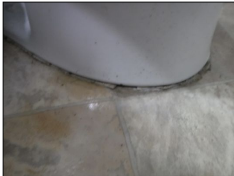
Caulk opportunities noted around the base of the toilet. Replacement is recommended.
