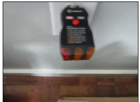
No power to outlet for unknown reason
