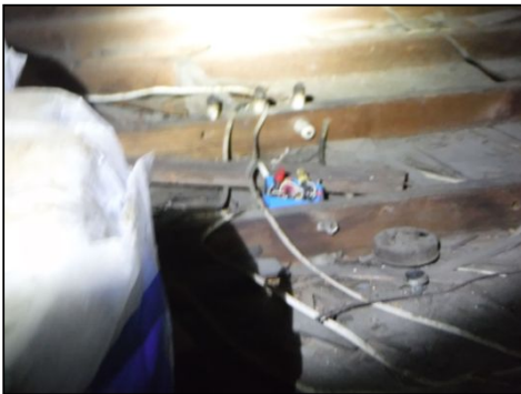
IMPORTANT NOTICE: Open junction boxes noted in the attic. Covering is recommended.
