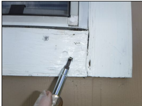
IMPORTANT NOTICE: Wood rot noted on the exterior trim in one or more areas. Replacement is recommended.
