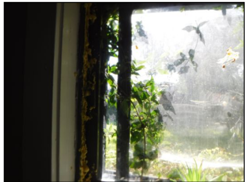
IMPORTANT NOTICE: Vines were growing inside the window frame on one of the bedroom windows. Removal of the vines and sealing of the window is recommended.
