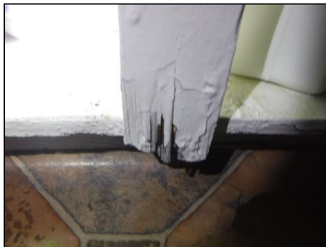
Damage noted to the cabinets in one or more areas around the home.
