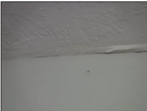
Tape seam showing in the bathroom. Proper repair is recommended.
