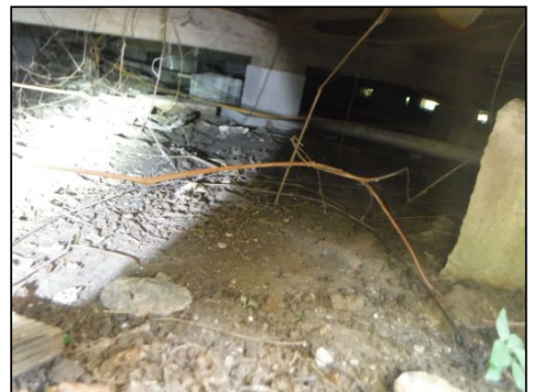
Plumbing lines in crawlspace not insulated
