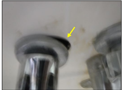
IMPORTANT NOTICE: Tub faucet handles were not sealed to the wall. Updating is recommended.
