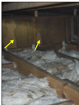
Evidence of previous moisture intrusion in the attic
