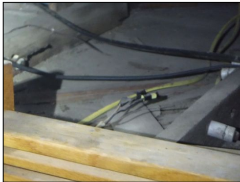
IMPORTANT NOTICE: Wiring connections were not installed in junction boxes in the attic. Further evaluation and proper repair is recommended.
