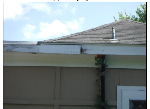
The fascia board has some deterioration on more than one location on the structure
