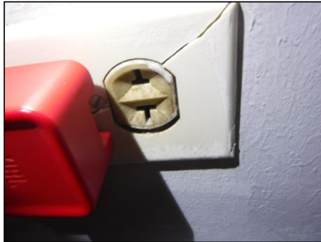
IMPORTANT NOTICE: Older two prong outlets were noted in one or more areas of the home. Updating to current standards is recommended. Damaged outlet cover noted as well.
