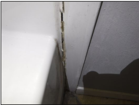
Caulk opportunities noted around the shower insert in one or more areas. Replacement is recommended to help maintain a water tight seal.
