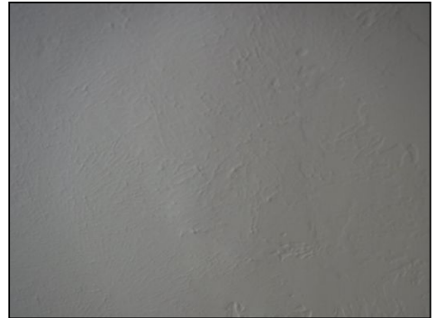
Previous repairs to ceiling did not appear to be of professional contractor quality.
