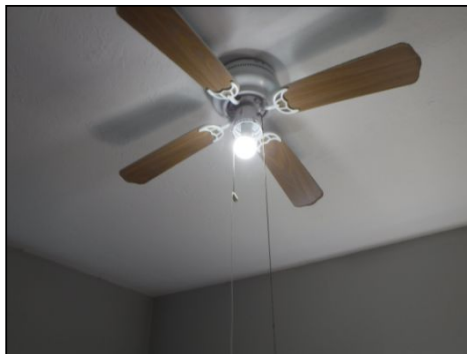
NOTE: Multiple light fixtures were missing covers. Replacement is recommended.
