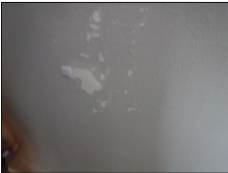
Previous repair and refinish did not appear to be of professional contractor quality.
