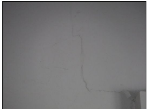
Wall cracks noted in one or more areas around the home. Further evaluation is recommended.
