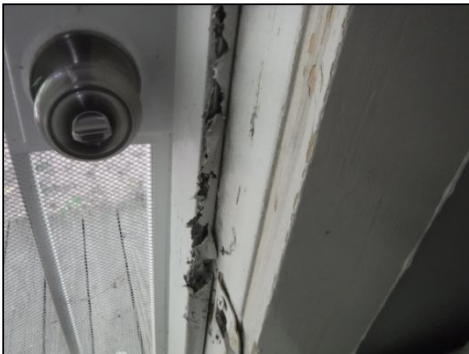
The weather strip on the side door was noted to be damaged. Replacement is recommended.
