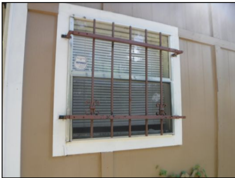
IMPORTANT NOTICE: Non-removable bars, grilles or screens were observed over one or more of the bedroom windows. When these obstructions are placed over emergency escape windows; they should be removable from the inside without the use of special tools or keys. At least one window in each bedroom should fully open with free access to the outside for safety concerns
