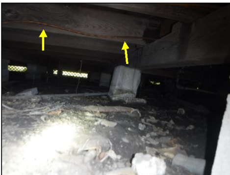
Wiring in crawl space not covered in conduit
