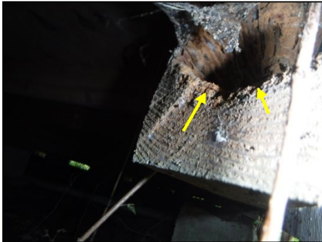
Wood damage in crawl space should be further investigated
