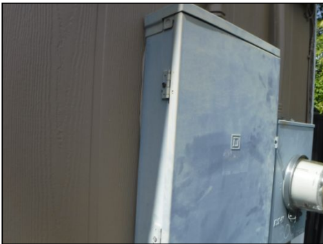
Gaps wider than {1/8"} around the service panel must be sealed.
