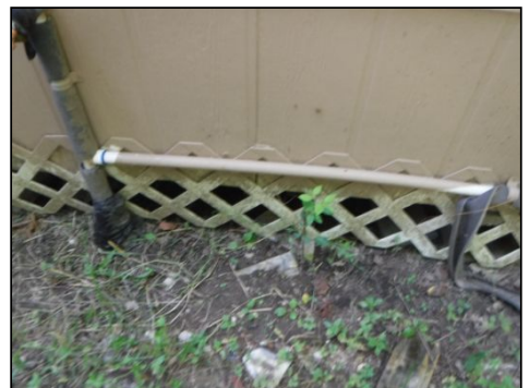
IMPORTANT NOTICE: Exposed water lines noted on the exterior of the home. Insulating the lines is recommended.
