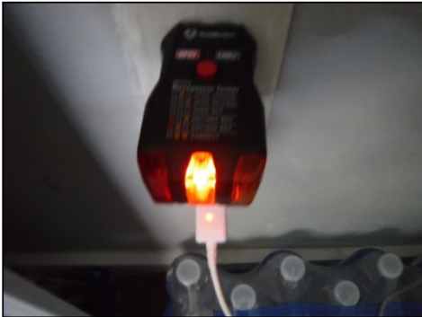
IMPORTANT NOTICE: One or more of the receptacles were noted to have an open ground. Review and repair by a licensed electrician is recommended.
