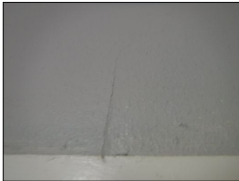
Wall cracks noted in one or more areas around the home. Further evaluation is recommended.
