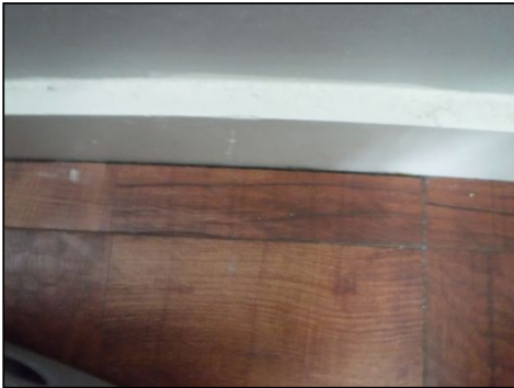
Caulk opportunities noted on the baseboard in multiple areas.
