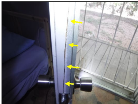
IMPORTANT NOTICE: The side entry door was noted to have a crack in it. Replacement is recommended.
