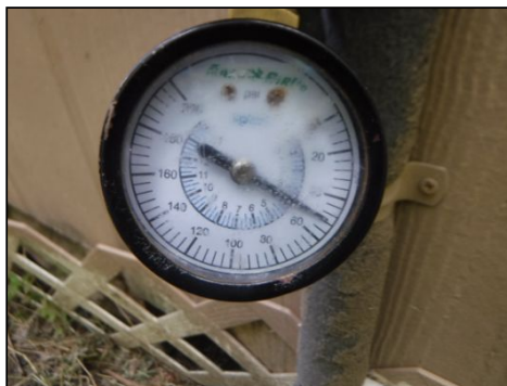
The anti static water pressure was observed at 49 psi.
