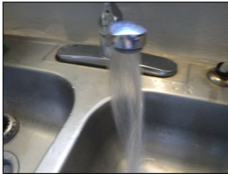
The kitchen faucet was missing an aerator. Replacement is recommended.
