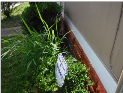
Maintenance: Shrubs planted too close to the house creating conditions conducive to infestation by Wood Destroying Insects (WDI). Shrubs should not be planted closer to the slab than half of the mature width of the shrub.
