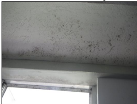
IMPORTANT NOTICE: A mold like substance was found growing on the ceiling of the bathroom. Further evaluation and proper repair is recommended.
