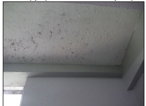
IMPORTANT NOTICE: A mold like substance was found growing on the ceiling of the bathroom. Further evaluation and proper repair is recommended.
