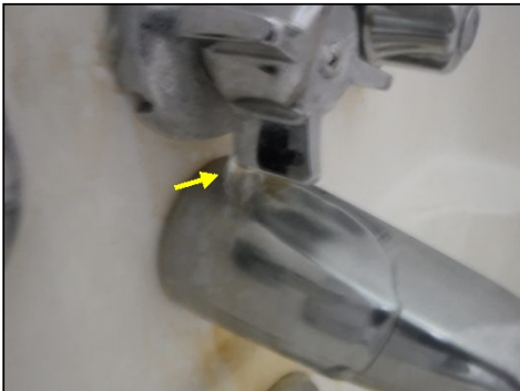
IMPORTANT NOTICE: The shower diverter was noted to leak. Further evaluation and proper repair is recommended.
