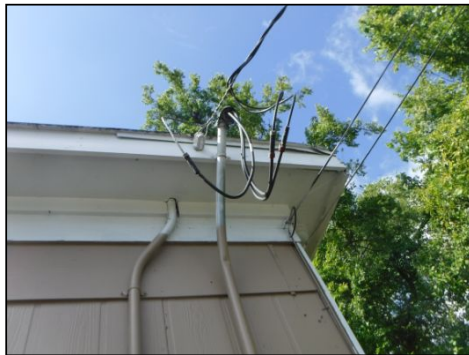
IMPORTANT NOTICE: The service entrance weatherhead does not have adequate clearance from the roof and/or structure.
