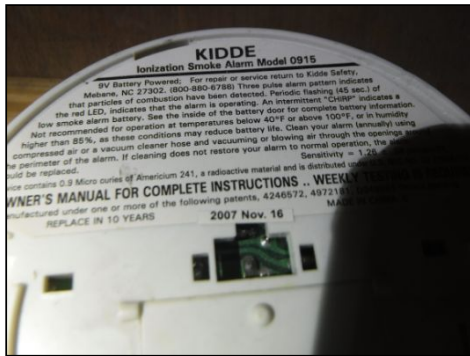
Smoke detector over ten years old
