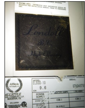
Lendell brand furnace
