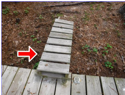
C. Item 4 (Picture) Improper walk boards boat house.
