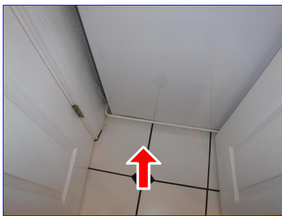
B. Item 1 (Picture) Drain pan under washing machine
