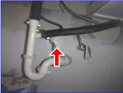
A. Item 1 (Picture) Primary drain line plumbed to the upstairs bathroom sink trap
