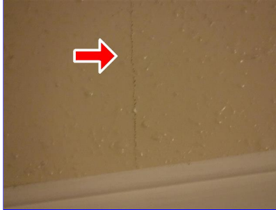
E. Item 2 (Picture) Sheetrock tape joint crack upstairs bedroom
