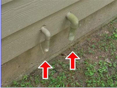
C. Item 1 (Picture) T&P valve and pan drain plumbed to the outside
