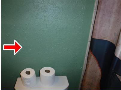
E. Item 1 (Picture) Signs of repair downstairs bathroom
