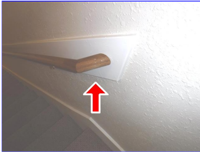
I. Item 1 (Picture) Rails return to wall per code
