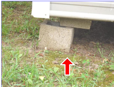
C. Item 2 (Picture) Improperly stacked blocks
