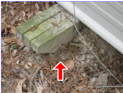
C. Item 3 (Picture) Wooden runners in contact with ground
