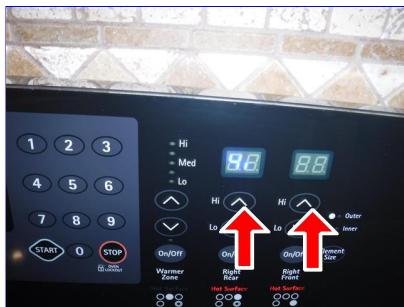
D. Item 1 (Picture) Burner display starting to go out.
