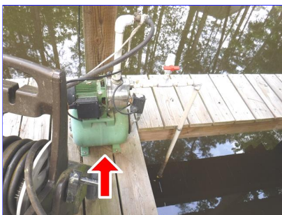
A. Item 1 (Picture) Lake pump
