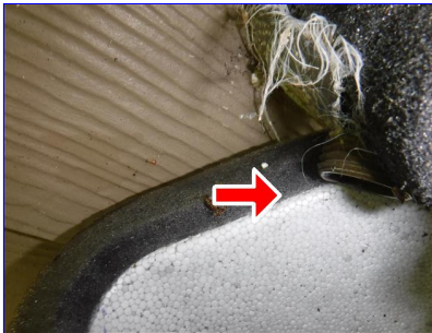
A. Item 2 (Picture) Missing anti siphon device
