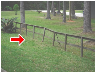
L. Item 1 (Picture) Fence in disrepair
