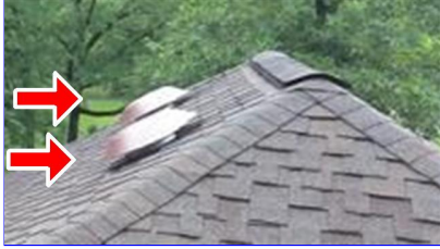
D. Item 1 (Picture) Recommend blocking old power vents
