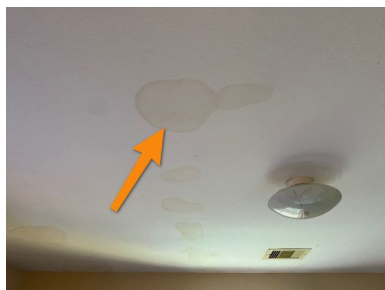
Ceiling stains at multiple locations in both units
