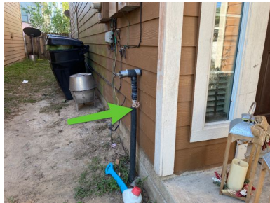
Unit B water shutoff valve
