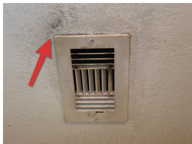
Unit b 1st Floor Bathroom
