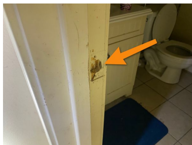
Unit b 1st Floor Bathroom
