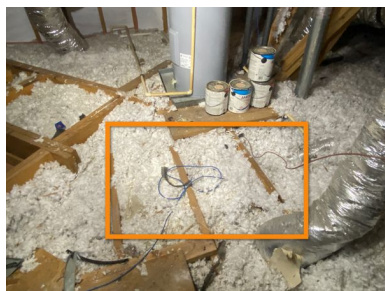
Missing attic decking to equipment
