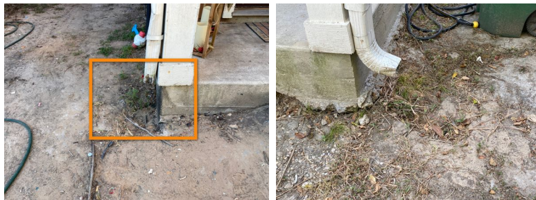
Hole in yard, missing downspout extension
