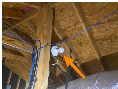
Lights were not working at several locations in both units
