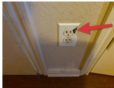
Cover plates were damaged in various areas in both units
