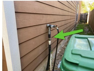
Unit A water shutoff
