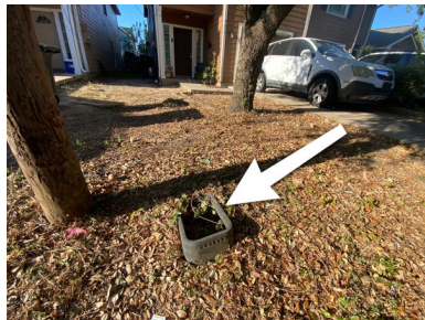
Water meter, unit b
