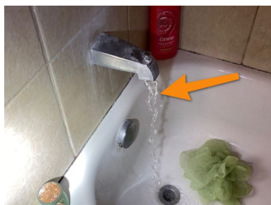
Low water pressure, both units
