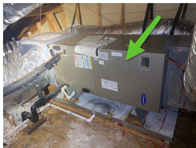
Unit B furnace
