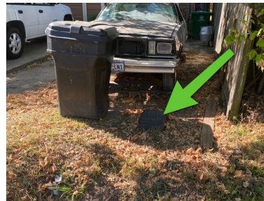
Water meter, unit a
