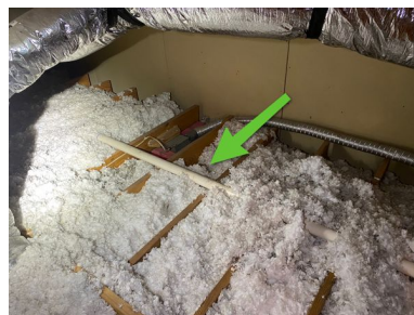
PVC drain pipe
