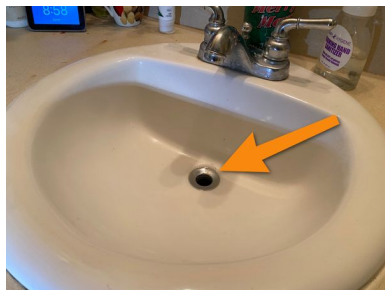
Drain stops missing at sinks at various areas in both locations
