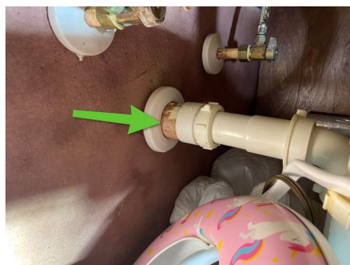
PVC drain pipe
