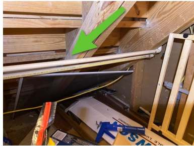
PVC water supply pipe
