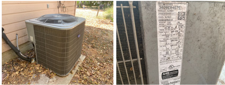
Interior - photo(s) of 1st cooling system: Electric Central Air Conditioning
