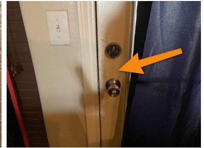
Doors did not latch
