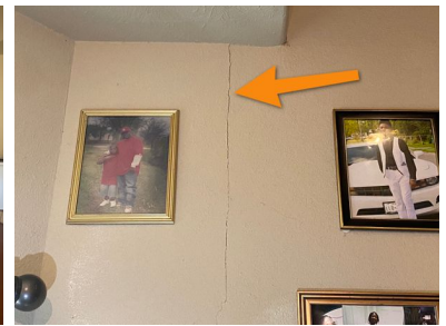
Wall crack, unit b
