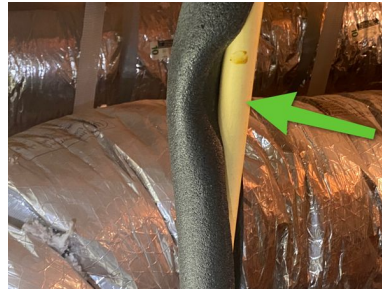
PVC water supply pipe
