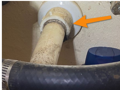
Under sink, unit B
