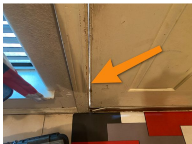
Weatherstripping was damaged at doors in both units
