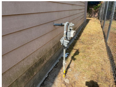
Unit a, right side
