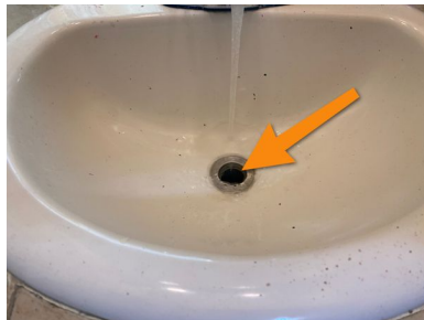
Drain stops missing at various locations
