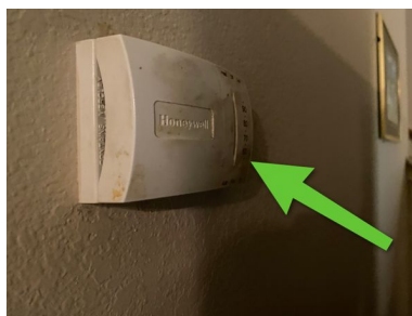
Inaccessible behind the TV - Furnace not tested
