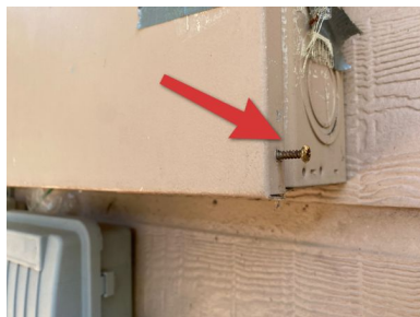
Improper method to secure the cover
