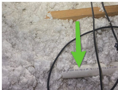
PVC drain pipe
