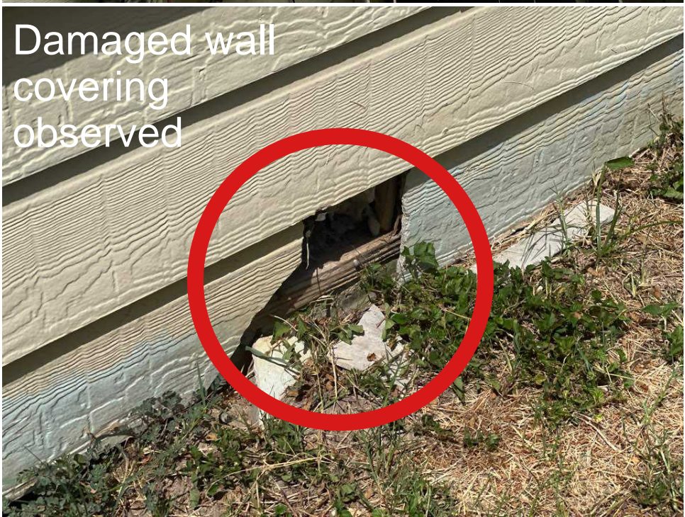
Damaged wall covering observed
