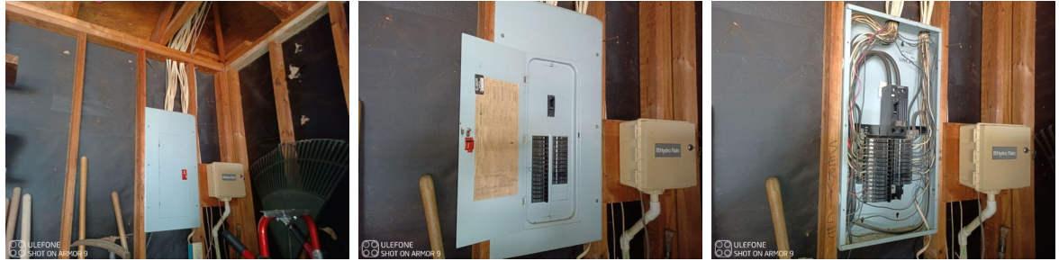
General Infrared Photos of Distribution Panels:
