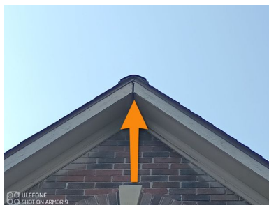
Fascia Separation, Front Exterior
