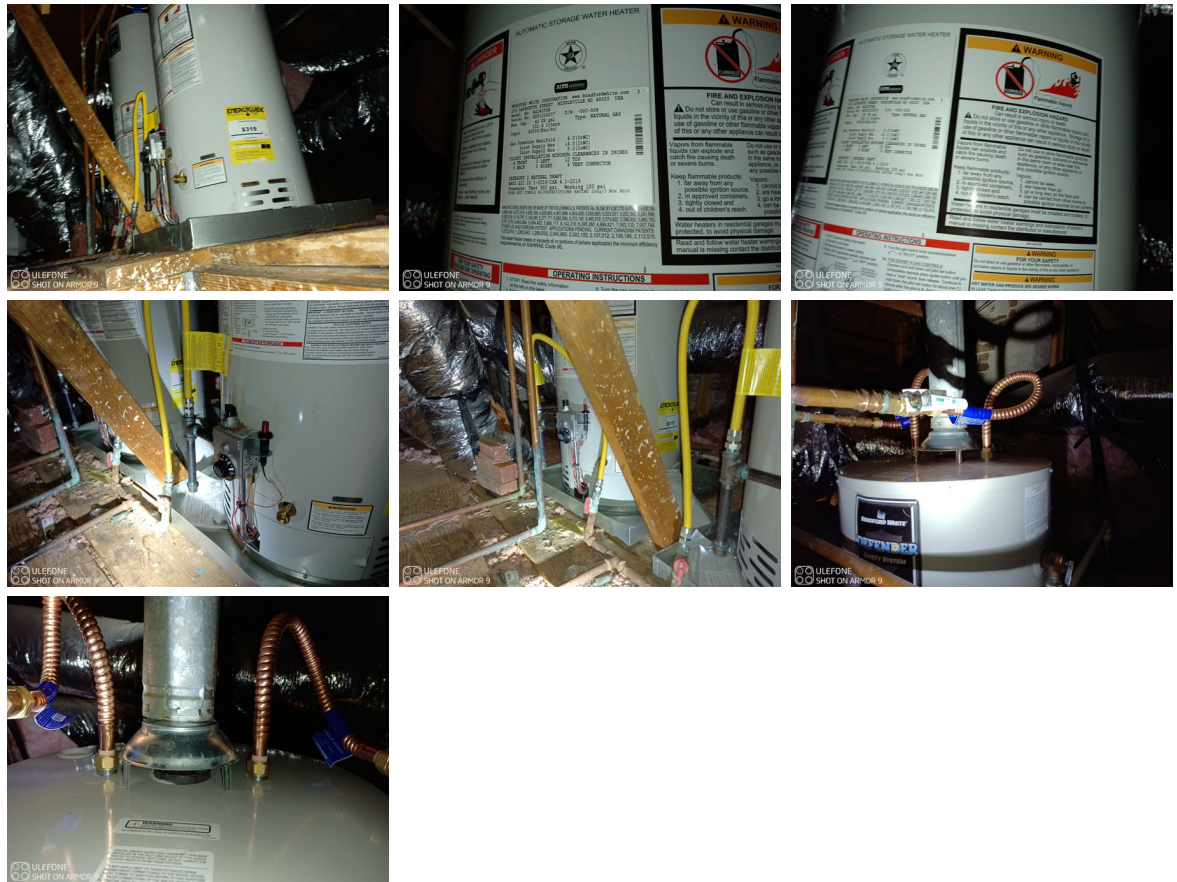
General Infrared Photos of Water Heating Equipment:
