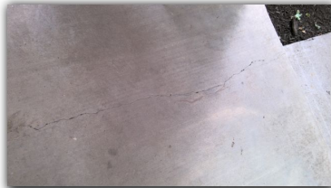
D - Cracks noted on the sidewalk. Recommend sealing cracks.
