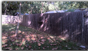
D - The fence is leaning and should be repaired.
