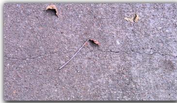
D - Cracks noted on the driveway. Recommend sealing cracks.
