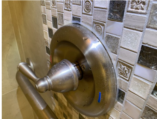
8. The hall bathroom tub faucet is dripping water.
