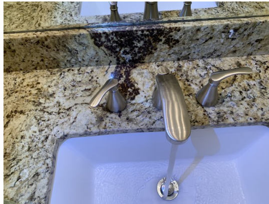
10. The hall bathroom shower diverter and shower head both leaked when tested.
