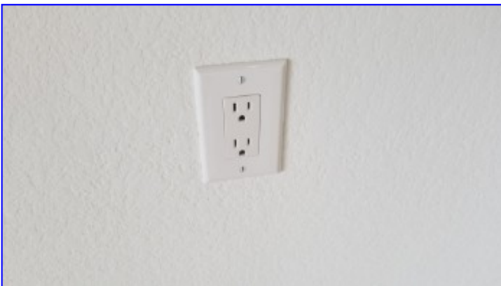
no gfci in garage
