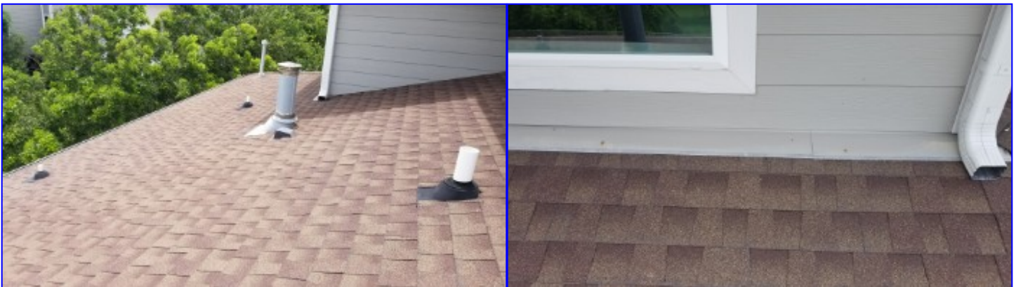
Uncoated/unsealed and or rusty flashing should be improved or repaired to prevent premature deterioration or failure. Maintaining flashing is crucial to prevent water intuition.
