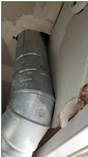
The furnace flue pipe is contacting the roof decking and should be repaired to allow the proper two inch clearance from all combustible materials.
