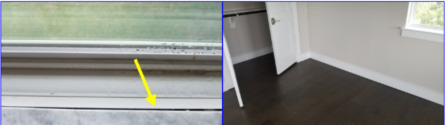
The window frame in the master shower should be sealed.
