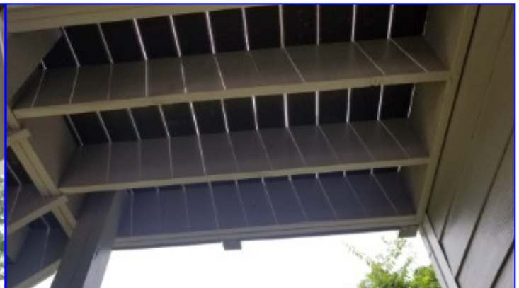
Joist hangers should be installed under the front and rear exterior stair landings to provide proper structural support.
