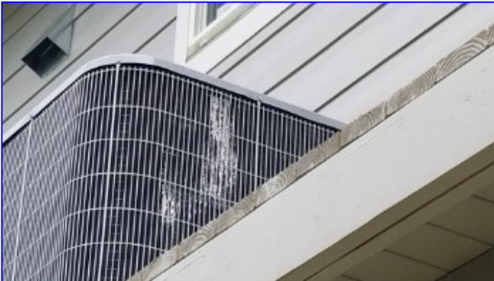
The fins of the outdoor portion of the air conditioning system were observed to be damaged and in need of repair. This condition can reduce the efficiency of the system.
