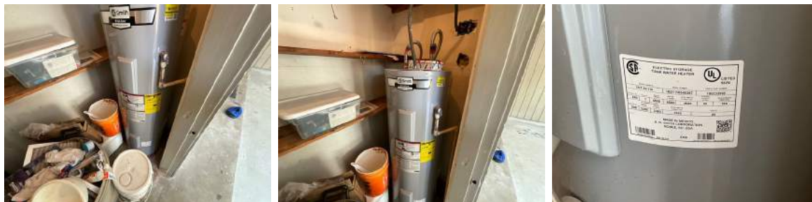
General Infrared Photos of Water Heating Equipment:
