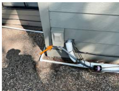
A/C Disconnect Box
