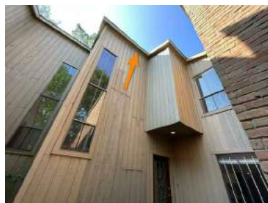
Soffit Vents Not Present
