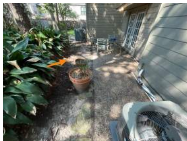
Negative Grading - Rear Exterior
