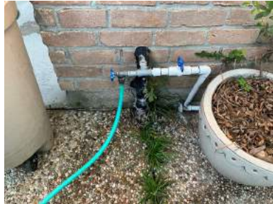
Static Water Pressure Reading: 50-55 PSI
