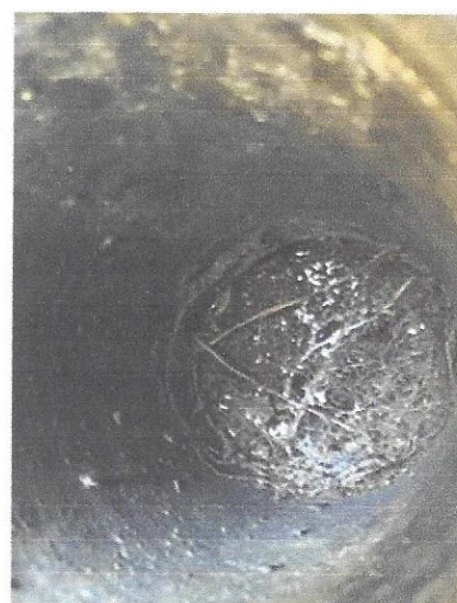
BREAK/ROOTS AT CLEAN-OUT
