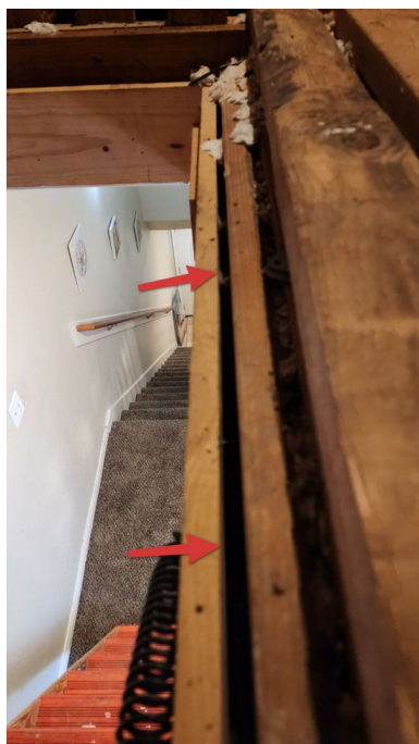
Missing shims at fasteners
