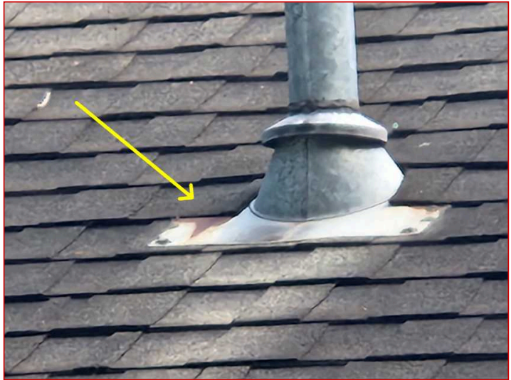
Flashing is rusty and should be painted.
