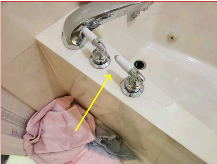
Hot and cold water lines are reversed
