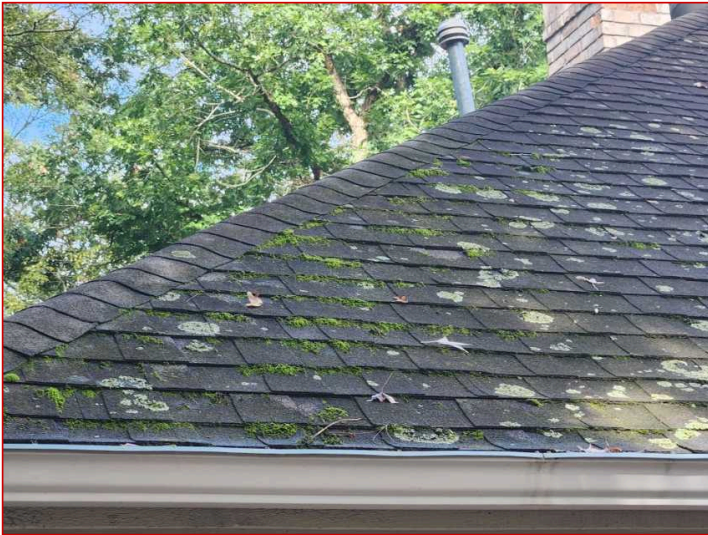
Some moss covered areas were observed on the roof from possible shade bearing tree branches which may promote acidity and shorten shingle life.
