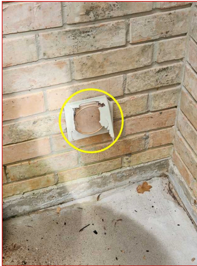
The dryer vent has either a damaged and/or missing exterior cover
