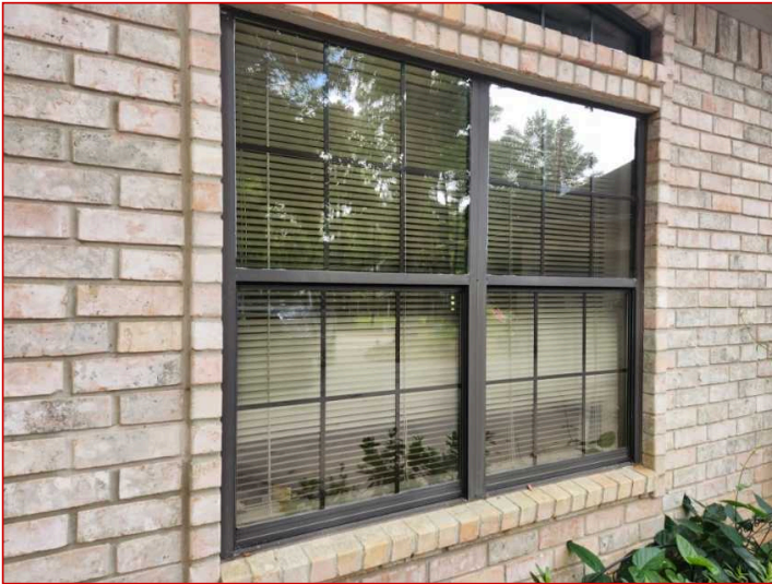
Window screens were observed to be damaged or missing.
