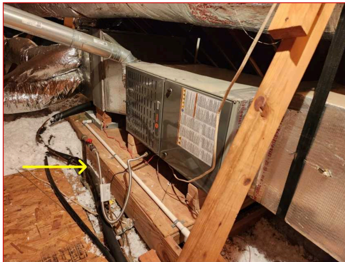
The gas supply line was not equipped with a required sediment trap just before the appliance connector. This helps keep trash out of the system.
