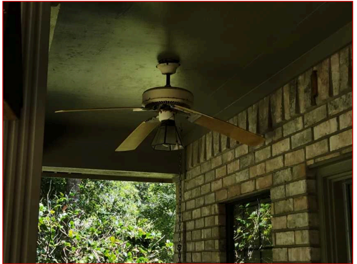
One or more ceiling fans were in bad condition.
