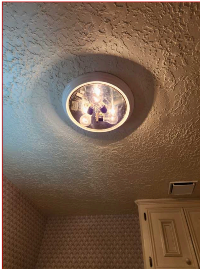
Light cover missing in guest bathroom.
