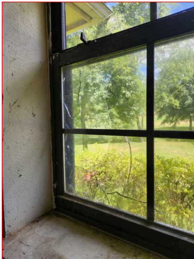
Cracked and/or broken glass was observed on one or more windows.
