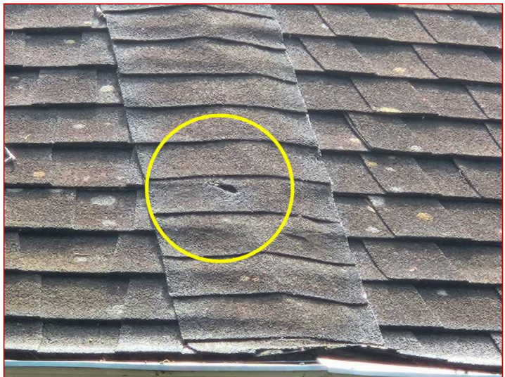
Damaged or missing shingles were noticed.
