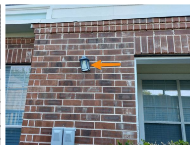
Around Exterior Lights
