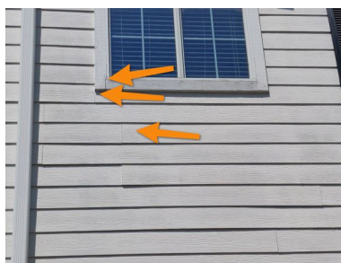
Siding on Back and Several Locations
