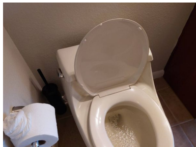
Handle Held Down to Flush in Master Bathroom
