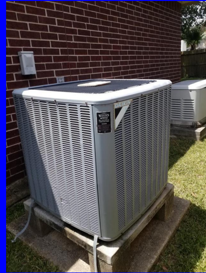
Hvac condenser located outside right side of home
