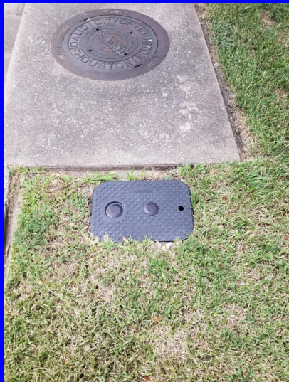
Water meter located front of home
