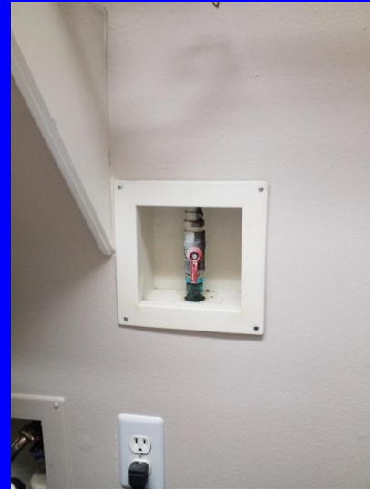
Main water shutoff located in Laundry room
