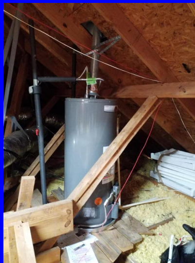
Gas water heater located in the attic space
