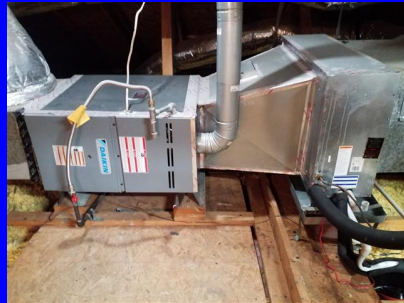
Gas furnace unit located in the attic space
