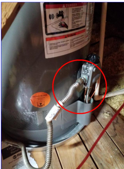
C. Item 2 (Picture) Water heater
