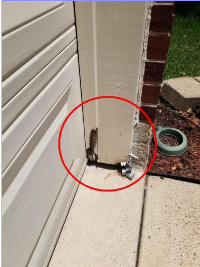
G. Item 1 (Picture) Garage door frame
