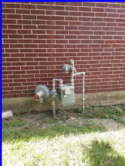
Gas meter located right side of home
