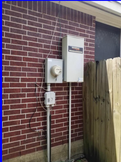
Electrical meter located outside right side of home
