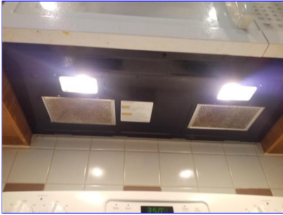
C. Item 1 (Picture) Tested and working
