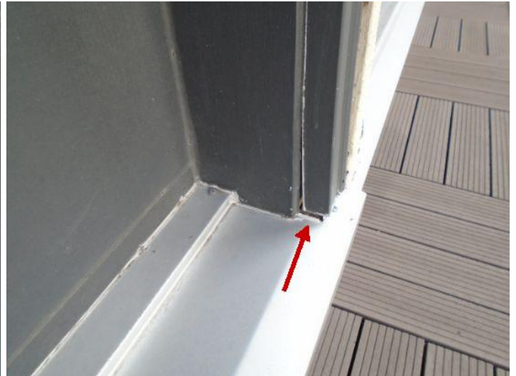
Balcony exterior siding has evidence of damages that may create an issue if not closely monitored.
