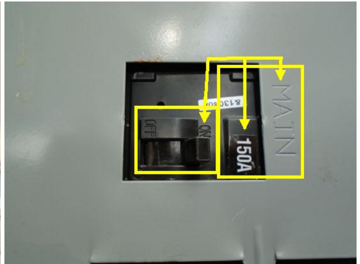
The main breaker is rated at 150 Amps and was working as intended.
