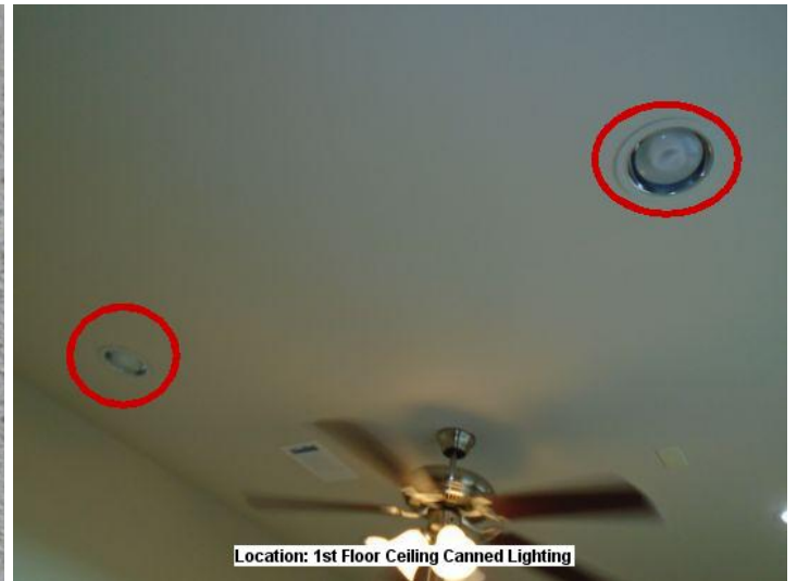
One or more overhead lights were unresponsive during today's inspection.
