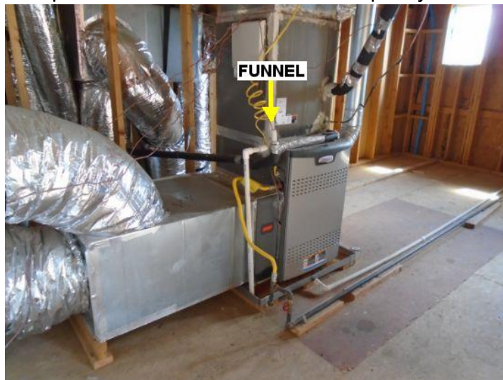
In attic and connected to the air handler is a vertical PVC pipe that has an exposed open end, twice a year (at time change) - pour 2 cups of Clorox Bleach to mitigate algae build up in this drain / vent pipe.
