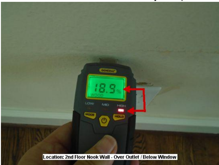
Moisture readings in two or more locations of the South facing walls were abnormal and further investigation may be necessary.
