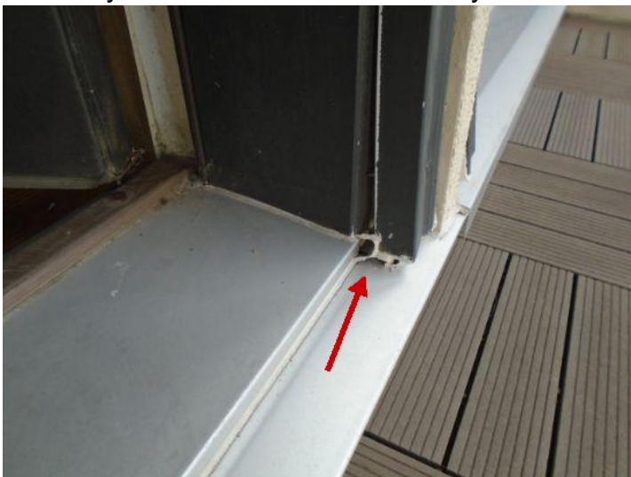
Balcony exterior siding has evidence of damages that may create an issue if not closely monitored.
