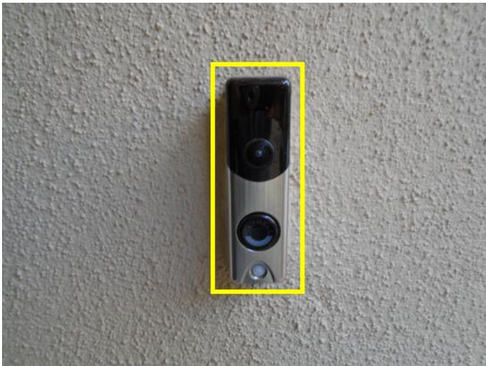
Front Doorbell was working as intended.
