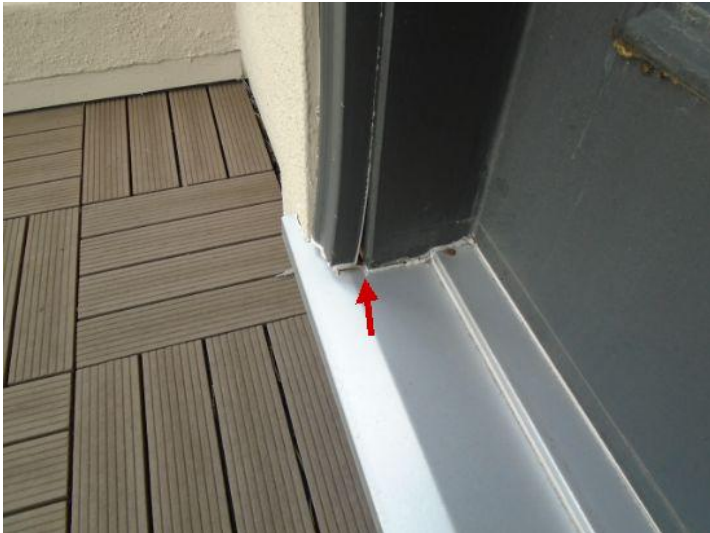
Balcony exterior siding has evidence of damages that may create an issue if not closely monitored.
