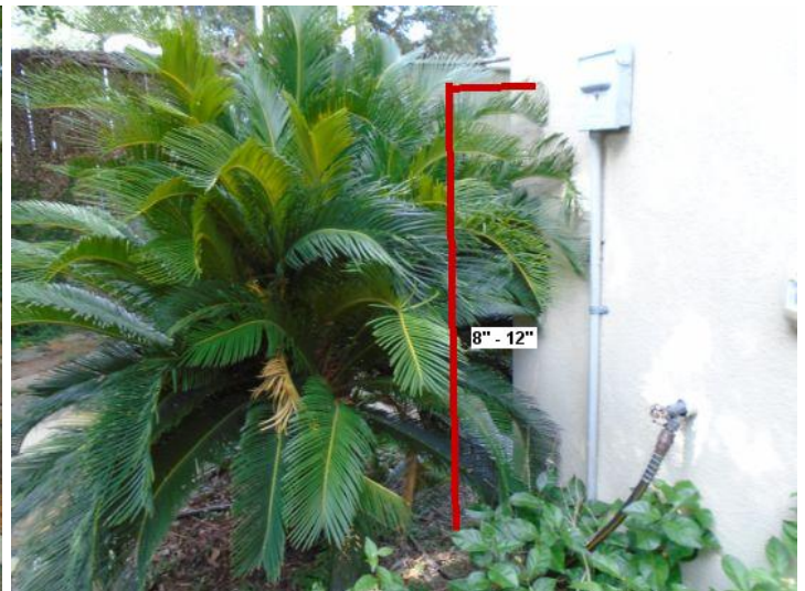
Cut all bushes away from the brick wall 8"-12" for best drying results.
