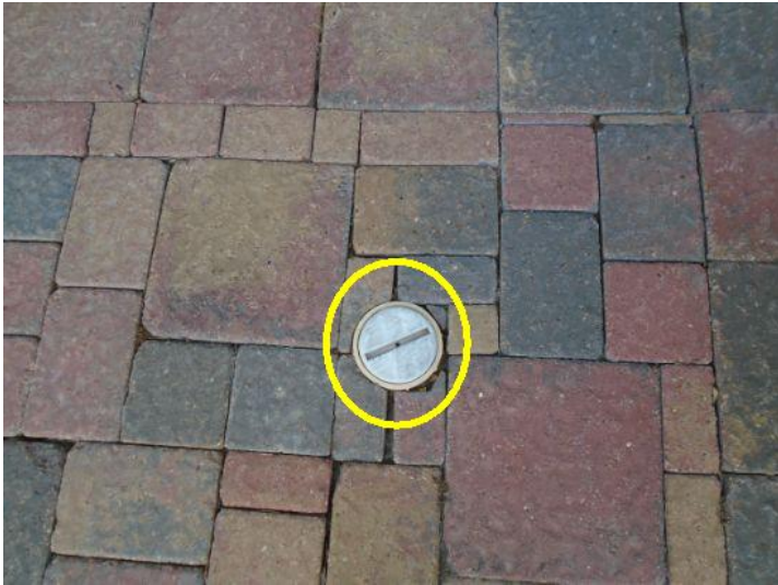
Main 4" plumbers clean out pipe is located in the front of the home.
