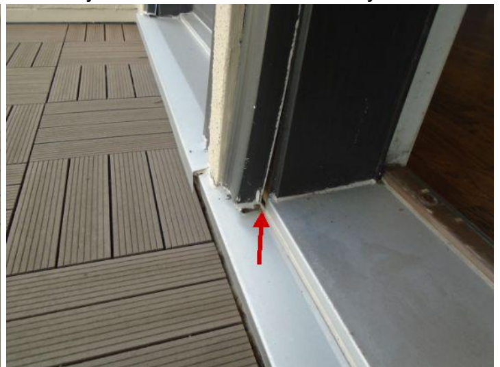
Balcony exterior siding has evidence of damages that may create an issue if not closely monitored.
