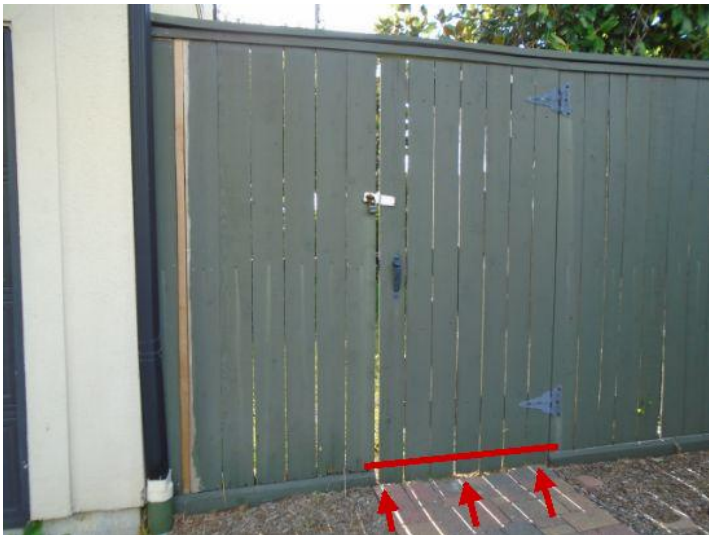
Fence gate is jamming up at the bottom and will not allow the gate to open or close properly.
