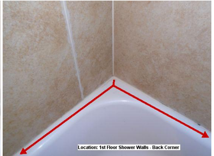
Evidence of cracked grout in one or more locations in the bathrooms of today's inspection.
