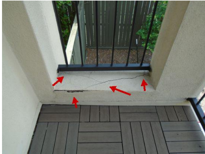
Front support beam mortar is cracked and or cracking.
