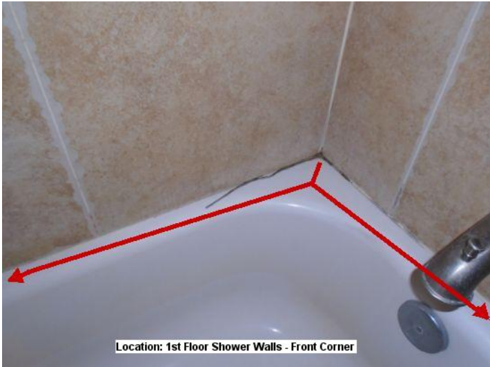
Evidence of cracked grout in one or more locations in the bathrooms of today's inspection.
