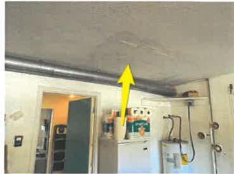
Garage: patching observed
