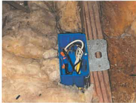
Attic: open junction box
