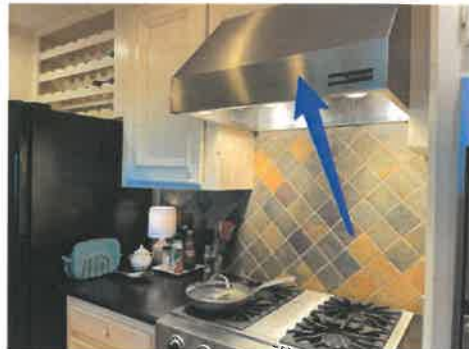
Vent hood OK
