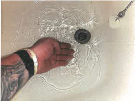
2nd floor hall bathroom: slow drain
