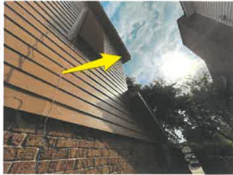
Left front: damaged soffit
