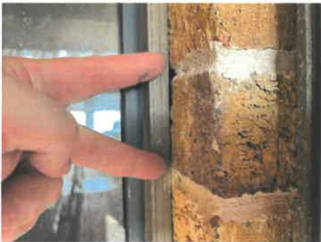
Caulking improvements needed around window frames on exterior side of the structure.
