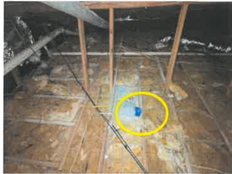
Attic: open junction box
