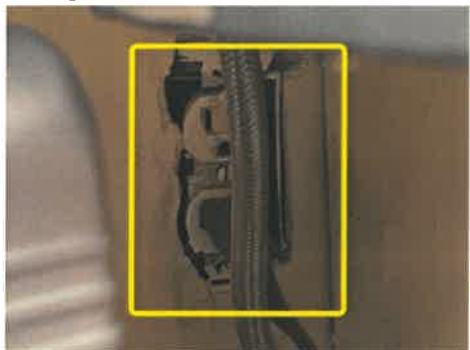
Kitchen: missing cover plate
