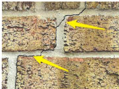
Crack in grout: typical movement, repair and monitor
