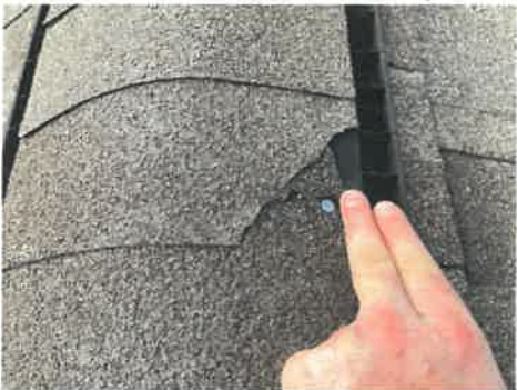
Damaged ridge cap shingle
