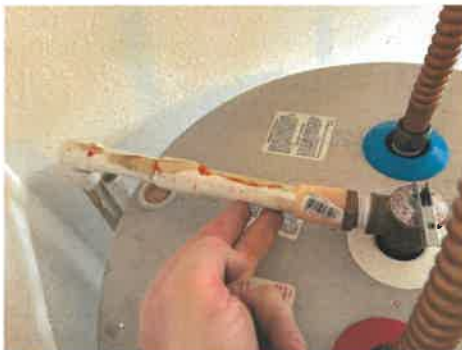
TPR discharge not proper
