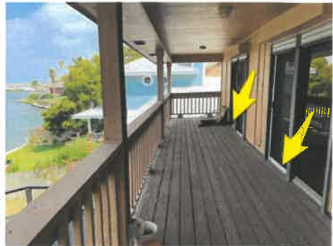
Upstairs bedrooms: screen door corrosion/damage
