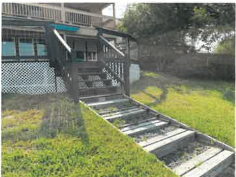
Wood to ground contact/ deck obstructs view of foundation face
