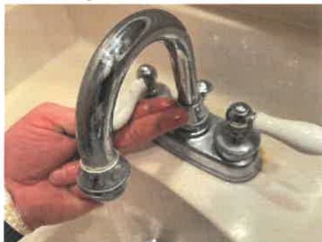
Hall bathroom: leaks at faucet on both sinks
