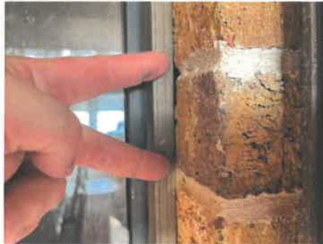
Caulking improvements needed around window frames on exterior side of the structure.
