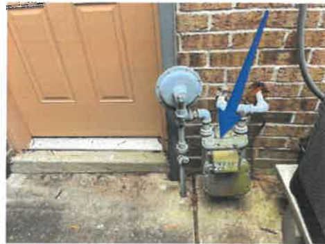
Right: gas meter
