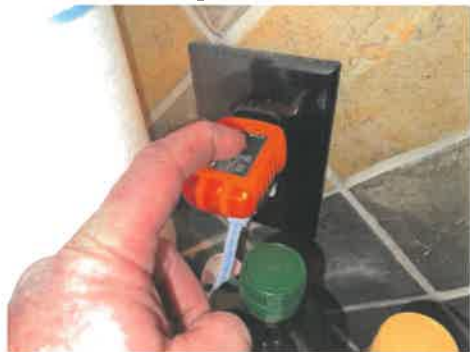
Kitchen: not all GFCI protected
