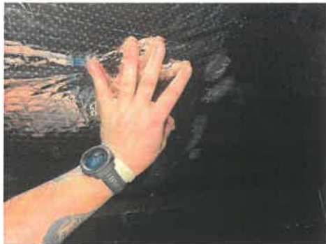
Barrier in place blocks visual inspection of roof sheathing
