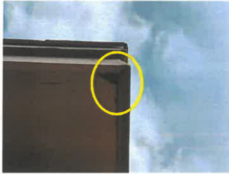
Left front: damaged soffit
