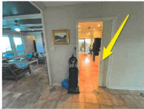
Kitchen: door doesn't close all the way
