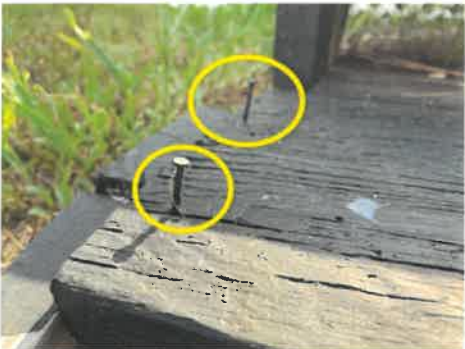
Damaged steps/raised nails
