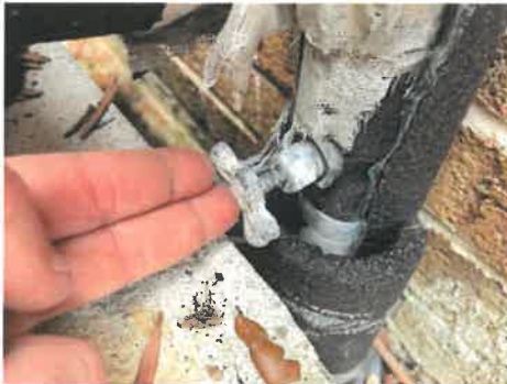
Right: water shut off valve
