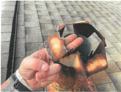
Rusted/damaged rain cap on exhaust flue
