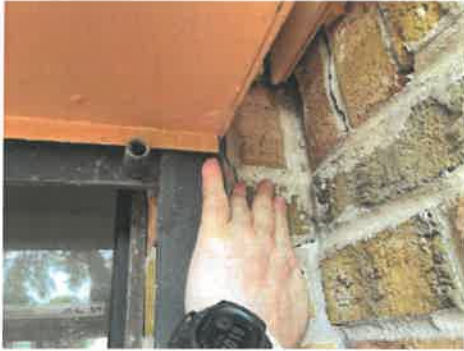
Front: loose brick veneer needs repaired
