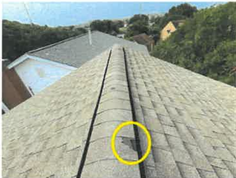
Damaged ridge cap shingle
