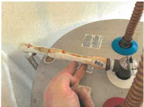
TPR discharge not proper
