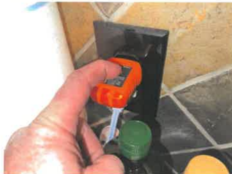
Kitchen: not all GFCI protected
