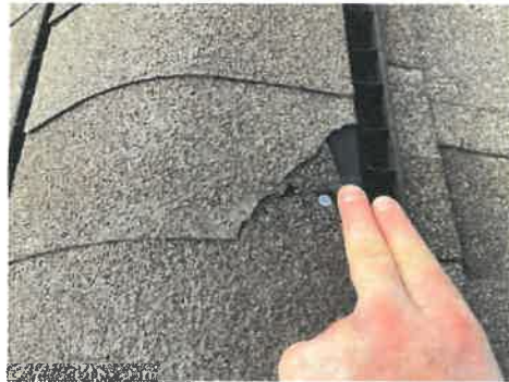
Damaged ridge cap shingle
