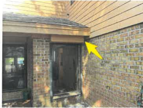
Front: loose brick veneer needs repaired
