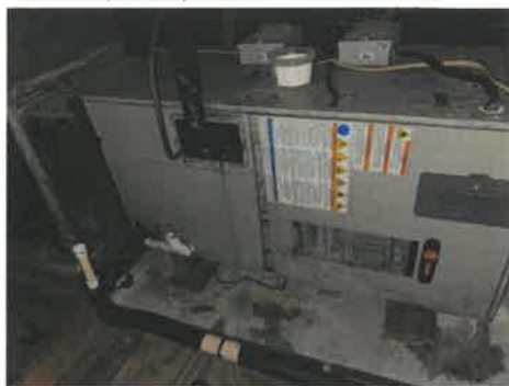
Condensation buildup on outside of unit
