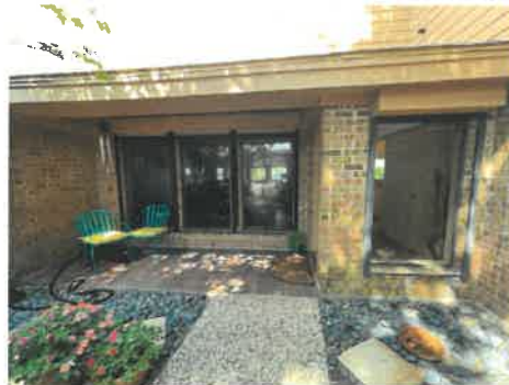
Caulking improvements needed around window frames on exterior side of the structure.
