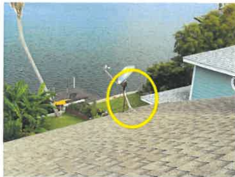
Satellite dish on roof
