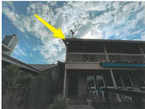
Right rear: missing trim board/fascia
