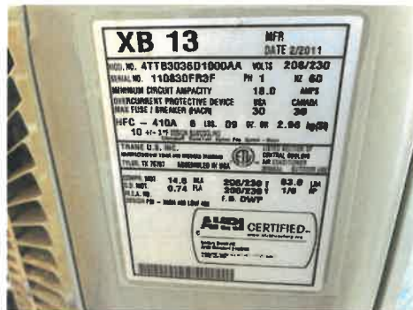
2nd floor unit: 2011 model 3 ton unit
