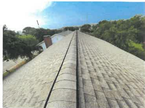
Minor granular deterioration
