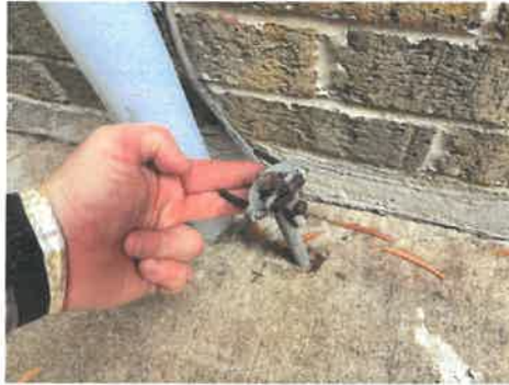
Ground wire/rod OK
