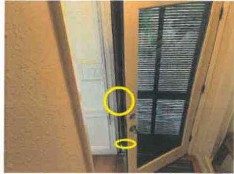
Back exterior door: won't latch
