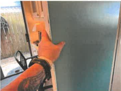
Garage door: not fire rated
