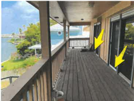
Upstairs bedrooms: screen door corrosion/damage
