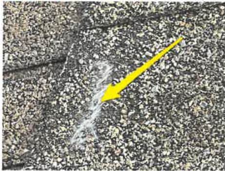
Minor granular deterioration
