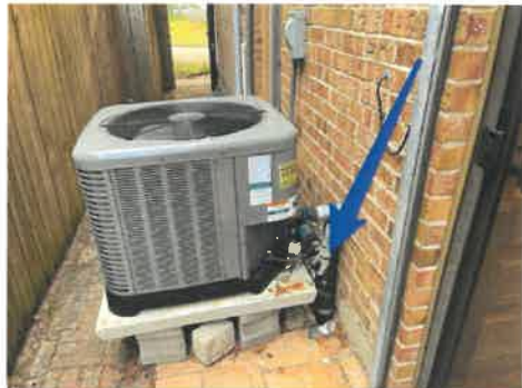
Right: water shut off valve
