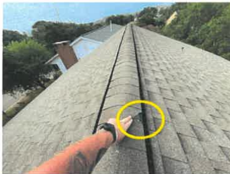
Damaged ridge cap shingle
