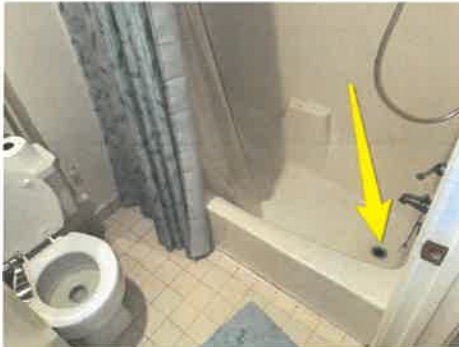
2nd floor hall bathroom: slow drain
