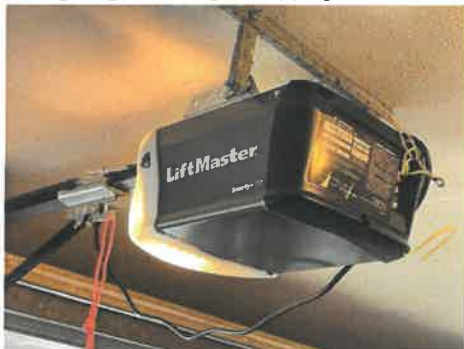
Liftmaster garage door opener OK
