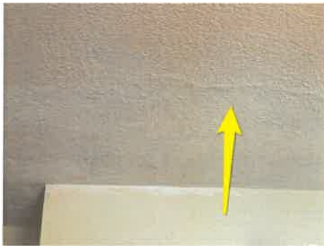
2nd floor rear middle bedroom: patching observed
