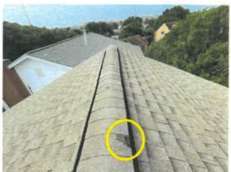
Damaged ridge cap shingle
