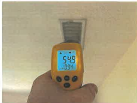
2nd floor supply cool-air temperature 54 degrees
