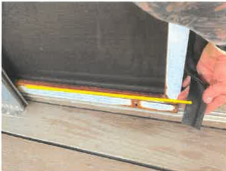
Upstairs bedrooms: screen door corrosion/damage
