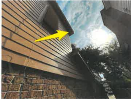
Left front: damaged soffit
