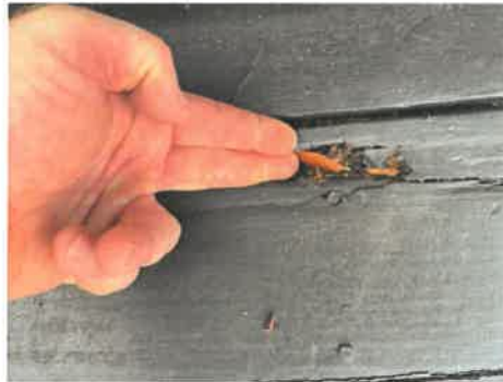
Deck has some deterioration: recommend replacement
