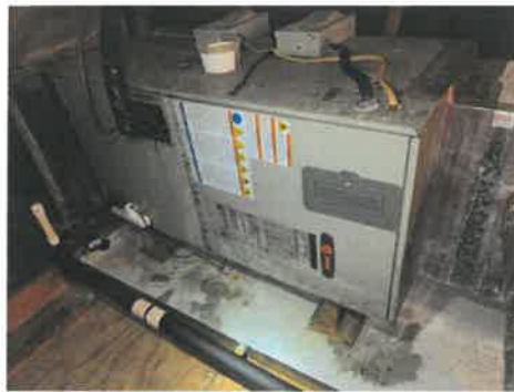
Condensation buildup on outside of unit
