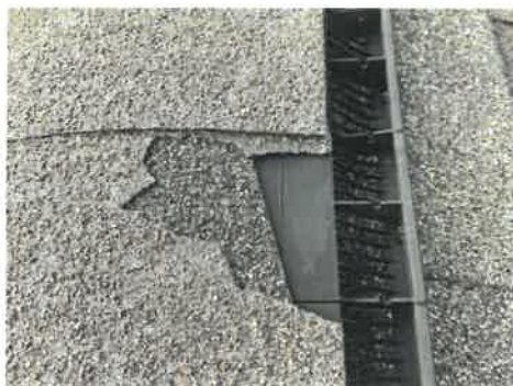
Damaged ridge cap shingle
