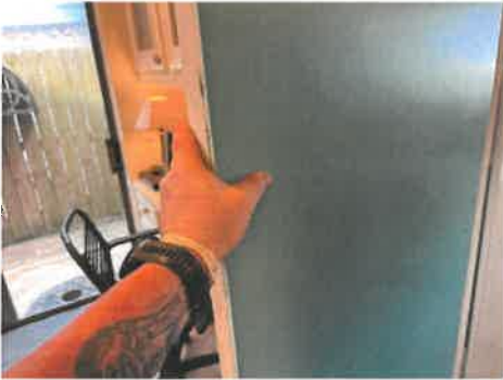
Garage door: not fire rated
