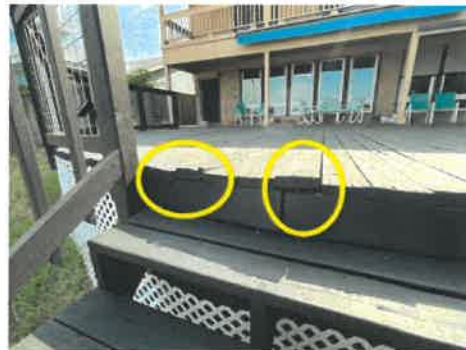
Raised decking needs secured in place
