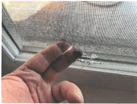
Living room: Window screen damage
