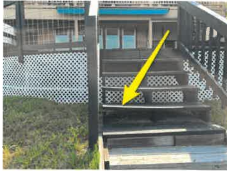
Damaged steps/raised nails
