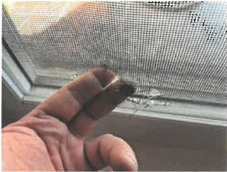
Living room: Window screen damage
