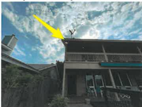
Right rear: missing trim board/fascia
