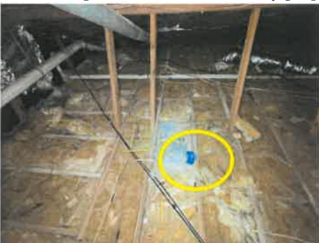
Attic: open junction box
