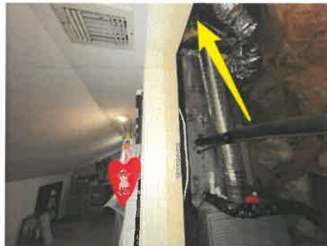
Fire stop missing
