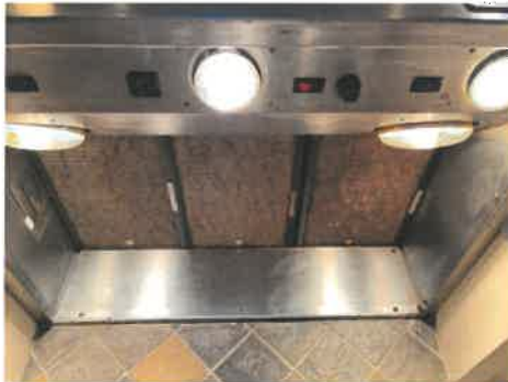
Vent hood OK
