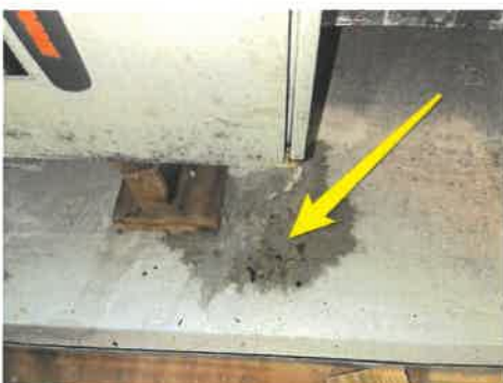
Condensation buildup on outside of unit
