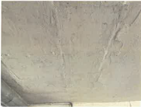
Garage: patching observed
