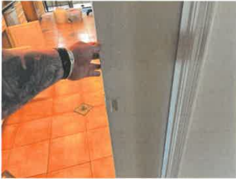
Kitchen: door doesn't close all the way
