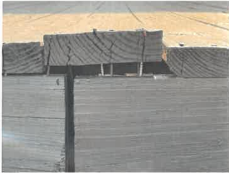
Raised decking needs secured in place
