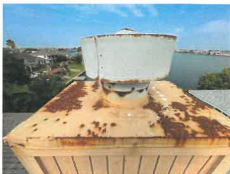
Chimney cap is rusted
