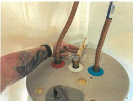
TPR discharge not proper
