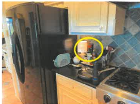
Kitchen: not all GFCI protected
