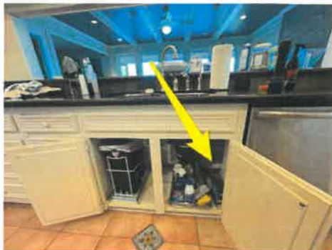
Kitchen: missing cover plate
