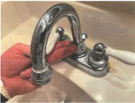
Hall bathroom: leaks at faucet on both sinks
