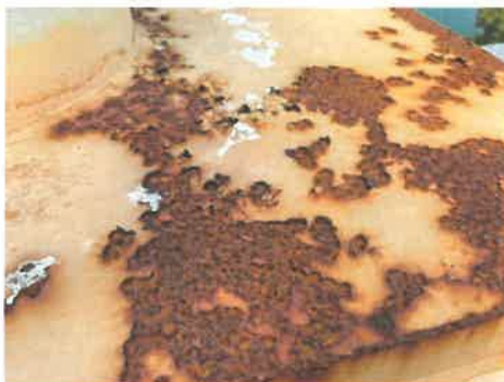
Chimney cap is rusted
