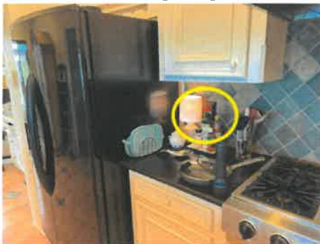
Kitchen: not all GFCI protected
