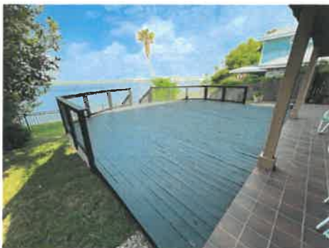
Deck has some deterioration: recommend replacement
