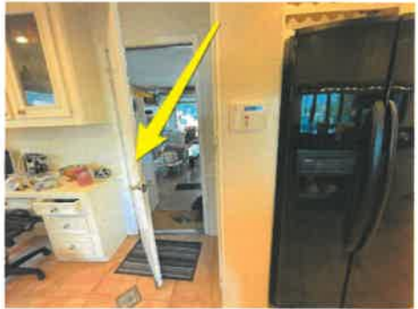
Garage door: not fire rated
