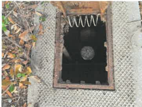
Front: water meter
