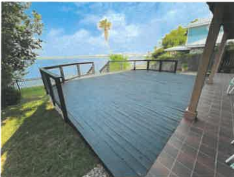
Deck has some deterioration: recommend replacement
