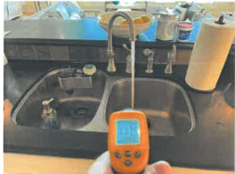
Hot water temperature
