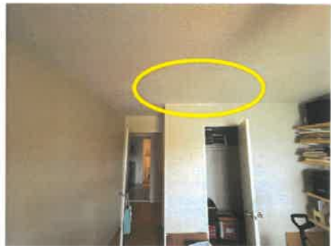
2nd floor rear middle bedroom: patching observed
