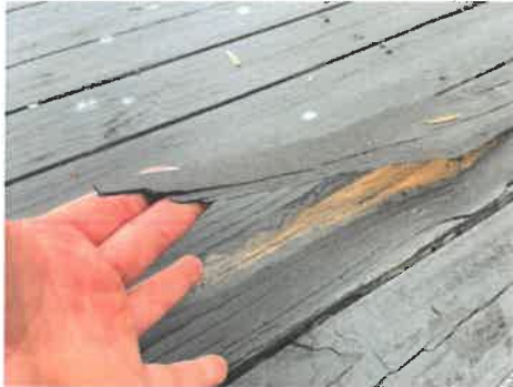
Deck has some deterioration: recommend replacement
