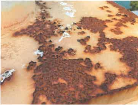
Chimney cap is rusted
