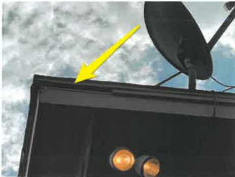
Right rear: missing trim board/fascia
