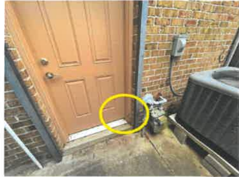
Right: wood decay
