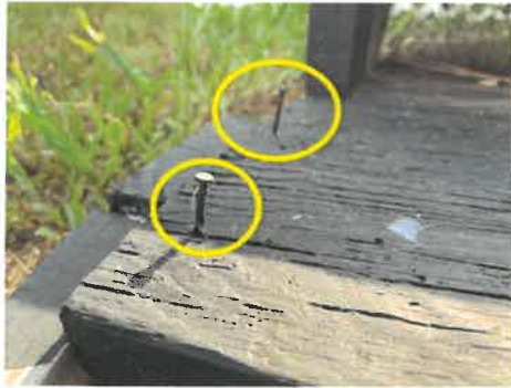
Damaged steps/raised nails
