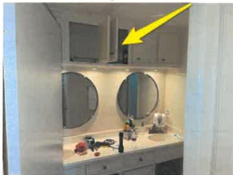
Master bathroom: open splice
