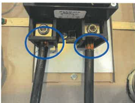
Garage: service panel with 2/0 copper service entrance wires
