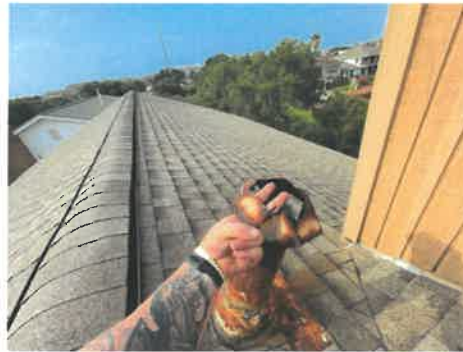
Rusted/damaged rain cap on exhaust flue
