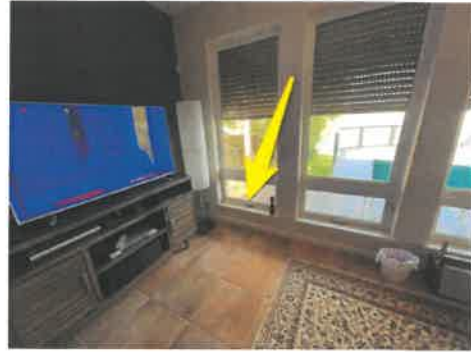
Living room: Window screen damage
