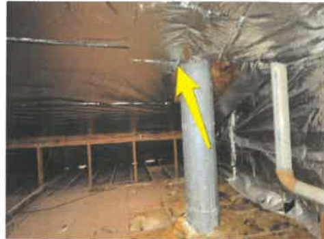
Moisture stain around chimney
