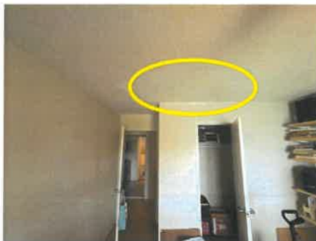
2nd floor rear middle bedroom: patching observed
