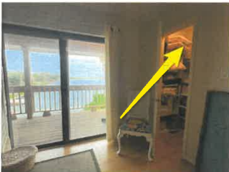
Right rear corner bedroom closet: moisture stain
