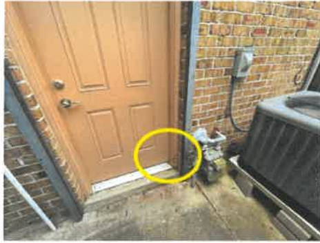
Right: wood decay
