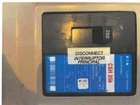
Garage: service panel with 200 amp disconnect
