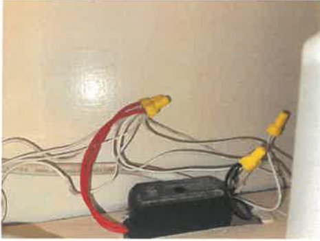
Master bathroom: open splice
