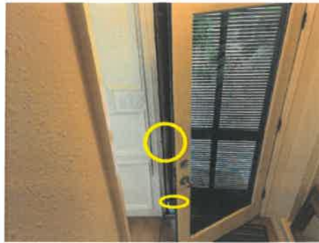
Back exterior door: won't latch
