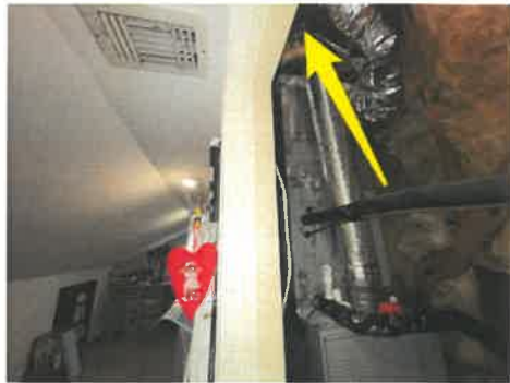
Fire stop missing
