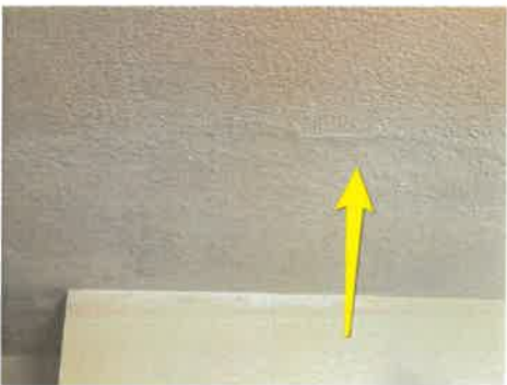
2nd floor rear middle bedroom: patching observed
