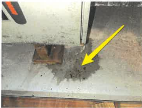
Condensation buildup on outside of unit
