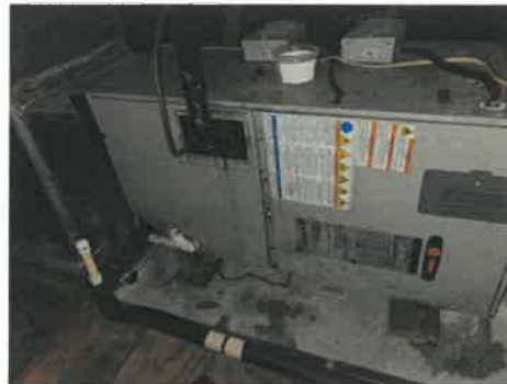
Condensation buildup on outside of unit
