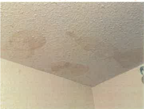
Right rear corner bedroom closet: moisture stain
