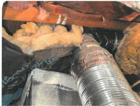
Fire stop missing
