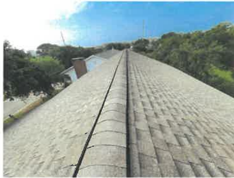
Minor granular deterioration
