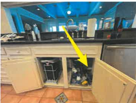
Kitchen: missing cover plate
