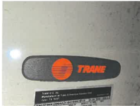
Unit 1 attic: Trane manufacturer
