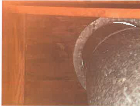
Moisture stain around chimney
