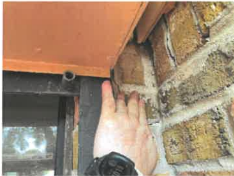
Front: loose brick veneer needs repaired
