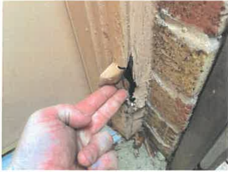
Right: wood decay
