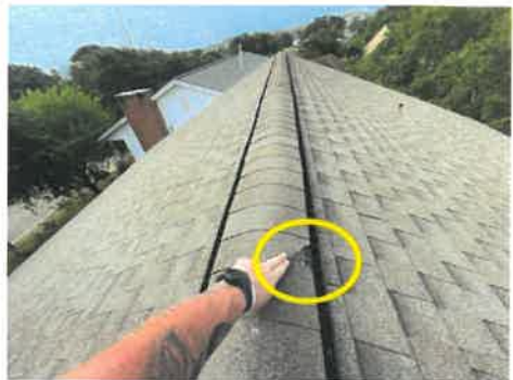
Damaged ridge cap shingle
