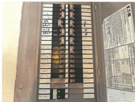
Garage: service panel appears properly labeled
