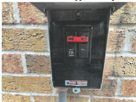
Service disconnects OK
