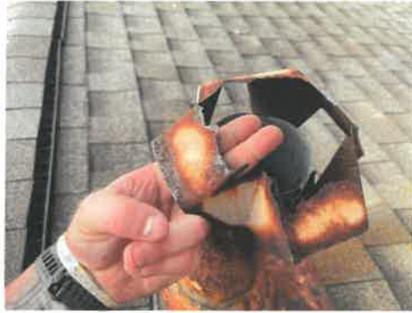
Rusted/damaged rain cap on exhaust flue
