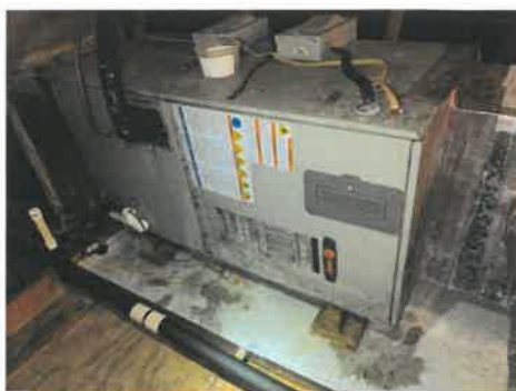
Condensation buildup on outside of unit
