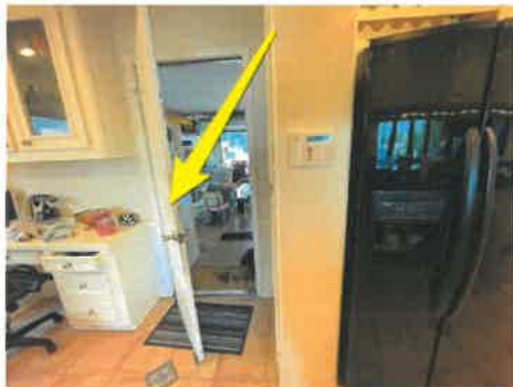
Garage door: not fire rated
