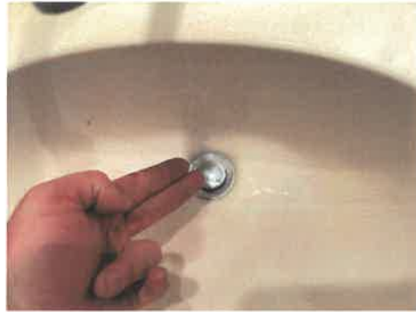
Hall bathroom: inoperable stopper
