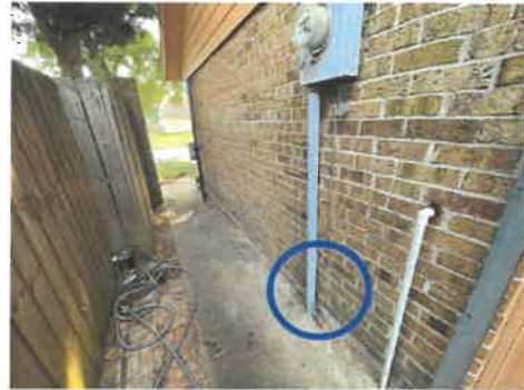
Ground wire/rod OK
