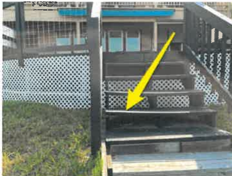
Damaged steps/raised nails
