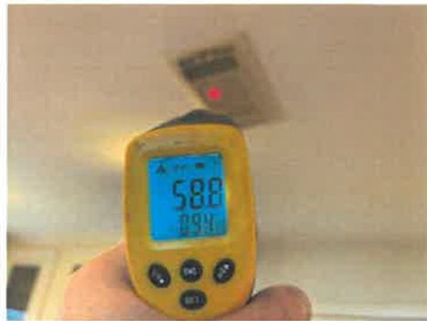
1st floor supply cool-air temperature 58 degrees
