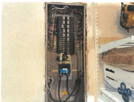
Garage: service panel with dead front off
