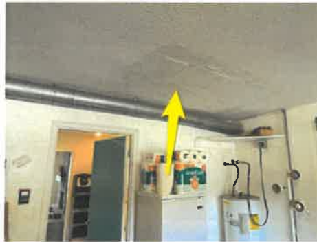
Garage: patching observed
