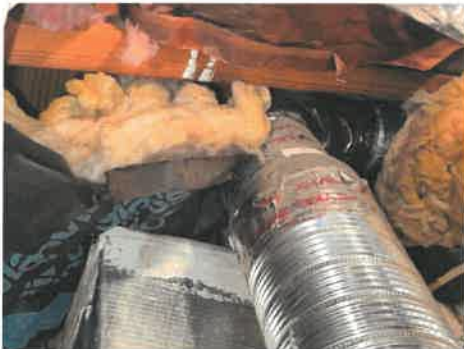
Fire stop missing
