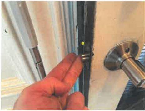
Back exterior door: won't latch
