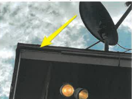
Right rear: missing trim board/fascia
