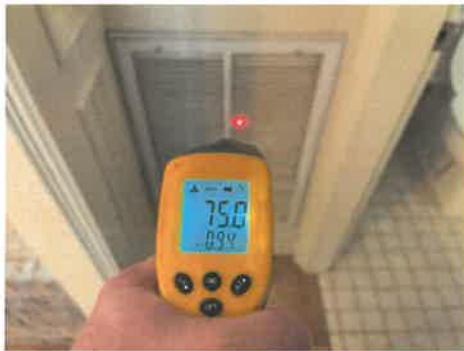
1st floor return air temperature 75 degrees
