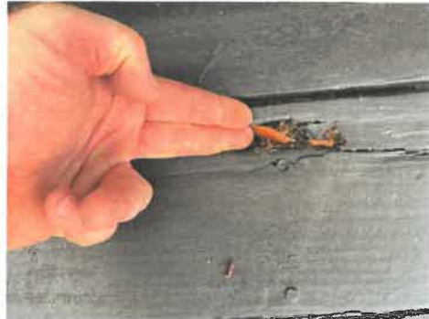
Deck has some deterioration: recommend replacement
