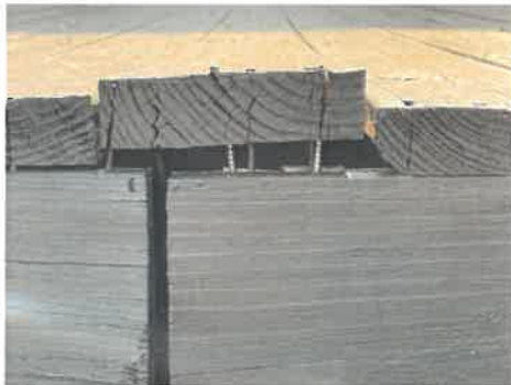
Raised decking needs secured in place
