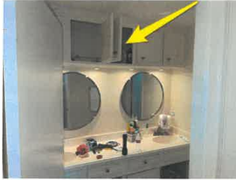
Master bathroom: open splice
