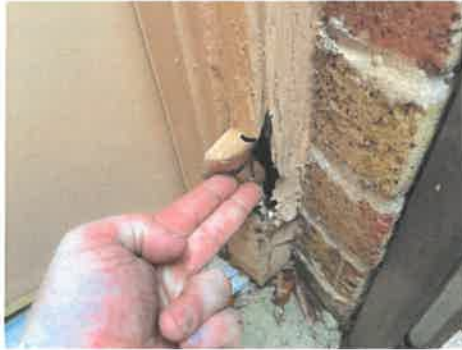
Right: wood decay
