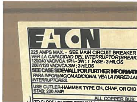
Garage: service panel Eaton manufacturer 225 amp rating
