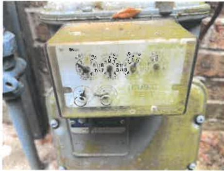
Right: gas meter
