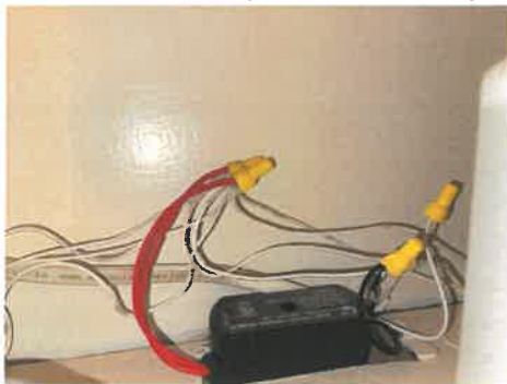
Master bathroom: open splice
