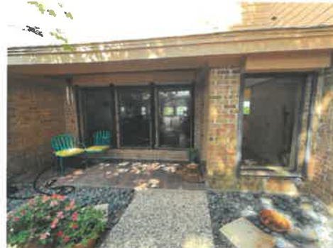
Caulking improvements needed around window frames on exterior side of the structure.
