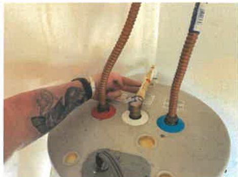
TPR discharge not proper
