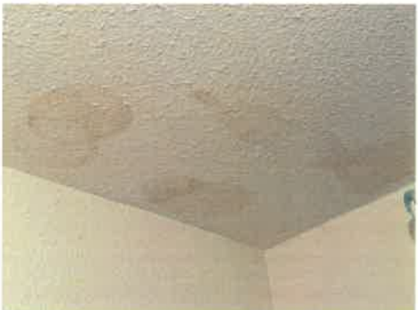
Right rear corner bedroom closet: moisture stain
