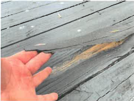
Deck has some deterioration: recommend replacement
