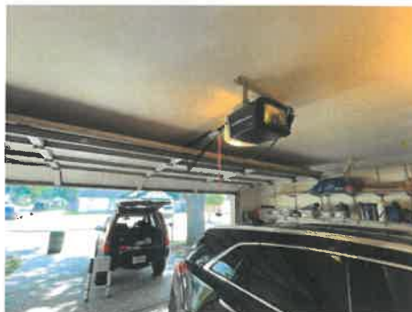
Liftmaster garage door opener OK
