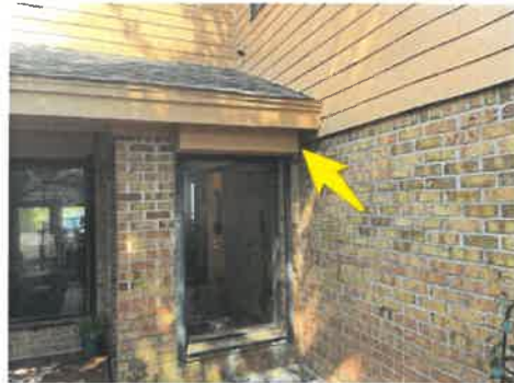
Front: loose brick veneer needs repaired
