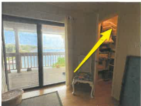
Right rear corner bedroom closet: moisture stain
