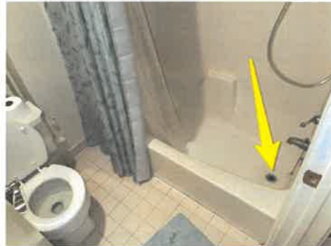
2nd floor hall bathroom: slow drain
