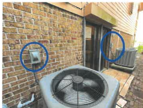
Service disconnects OK
