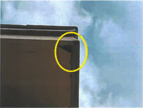
Left front: damaged soffit
