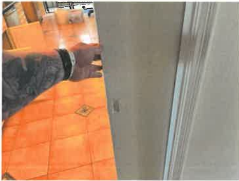
Kitchen: door doesn't close all the way
