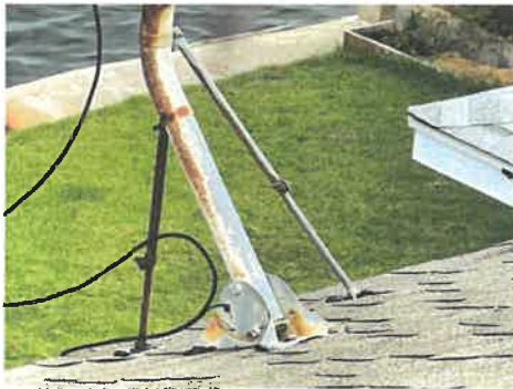
Satellite dish on roof
