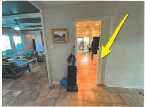
Kitchen: door doesn't close all the way
