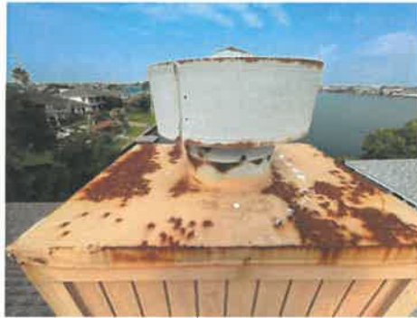
Chimney cap is rusted
