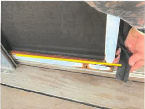
Upstairs bedrooms: screen door corrosion/damage
