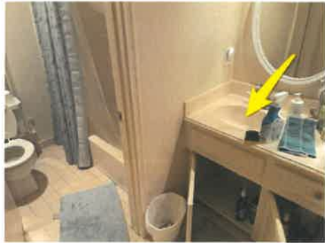
Hall bathroom: inoperable stopper
