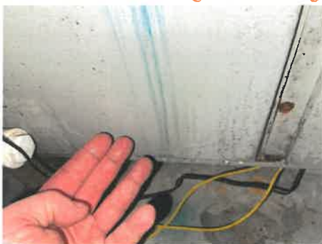
Condensation buildup on outside of unit
