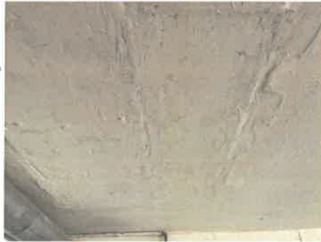
Garage: patching observed
