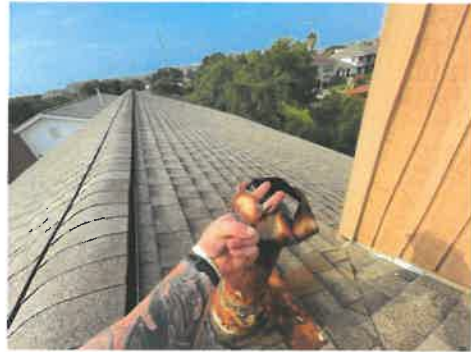
Rusted/damaged rain cap on exhaust flue
