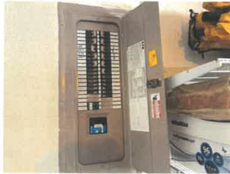
Garage: service panel
