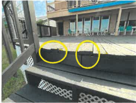
Raised decking needs secured in place
