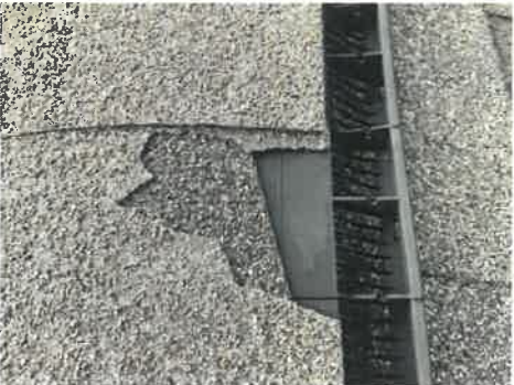
Damaged ridge cap shingle
