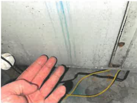
Condensation buildup on outside of unit
