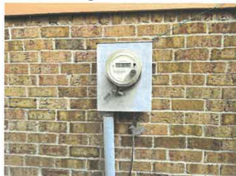
Right: service meter
