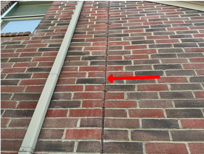
Brick seam seal improvements needed at right of home.
