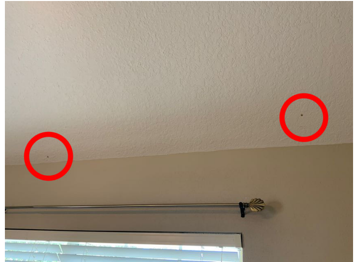
Nail pops throughout home.
