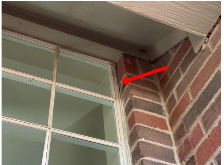
Exterior caulking improvements needed at front of home.
