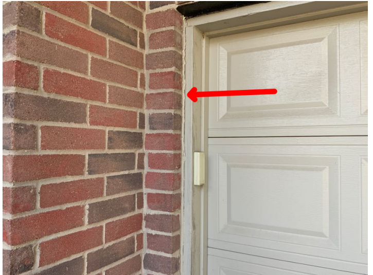
Trim board seal improvements needed at garage.
