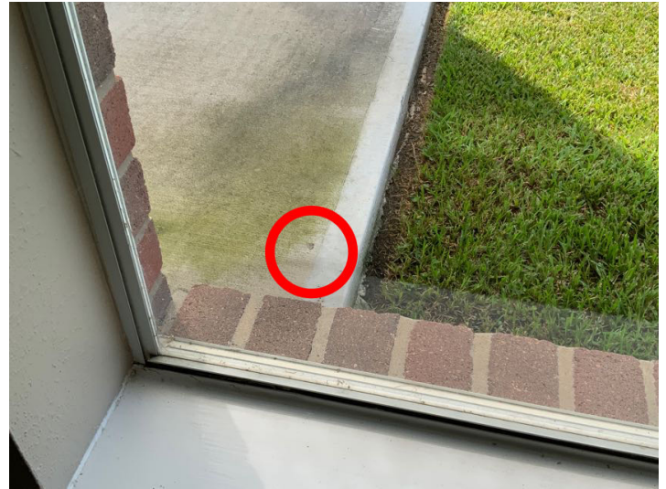
Cracked windows in living room.
