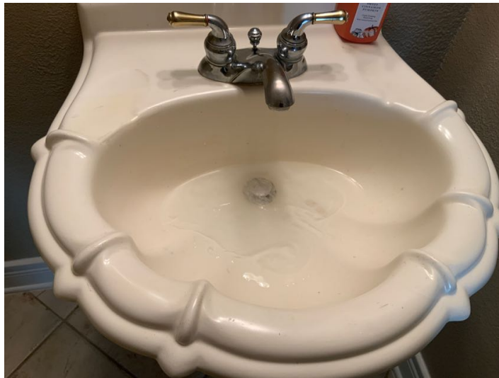
Slow drain at main bathroom sink.
