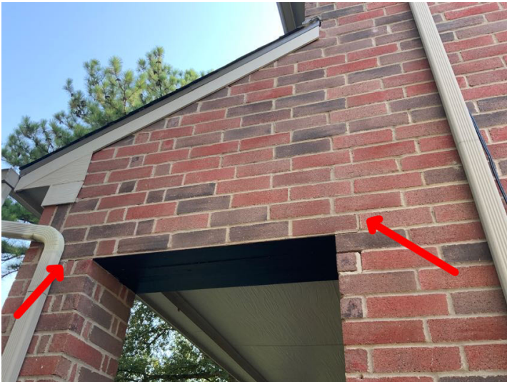
Lintel movement cracks at right of home.
