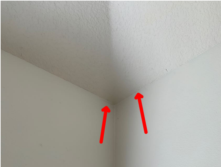
Seam failure in primary bedroom.
