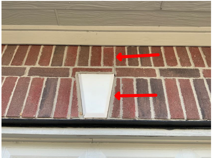
Minor settlement crack at front of home.
