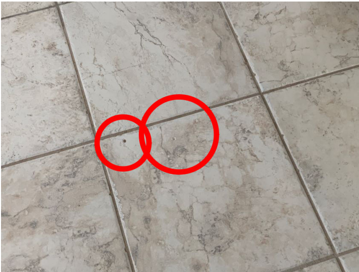
Chipped tile in primary bedroom.
