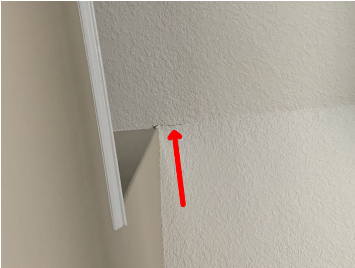
Seam failure at entryway.
