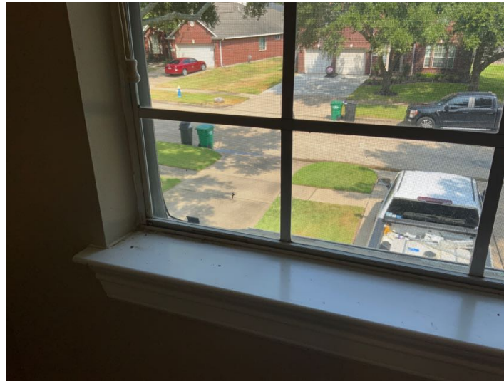
Damaged screen at upstairs front right bedroom.
