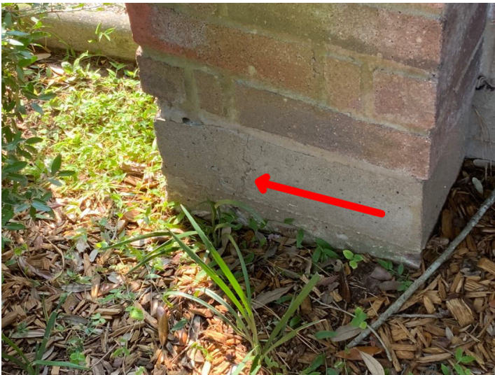
Broken front left corner.
