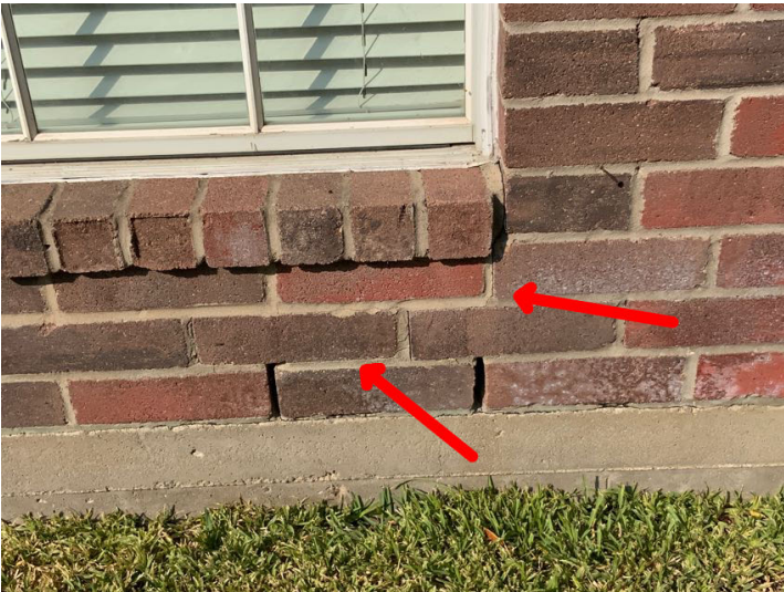
Minor settlement crack at left of home.
