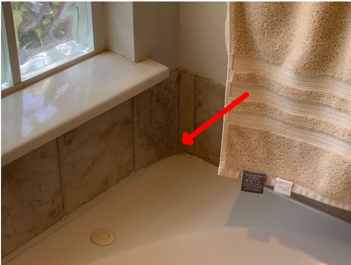
Bathtub enclosure caulking improvements needed at primary bathroom.
