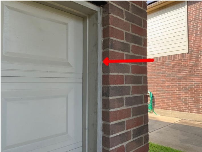
Trim board seal improvements needed at garage.
