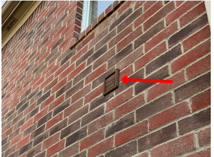
Vent perimeter seal improvements needed at right of home.
