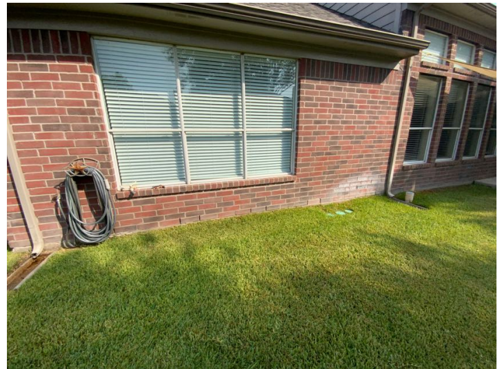
High soil blocking visual inspection of foundation at Back of home.
