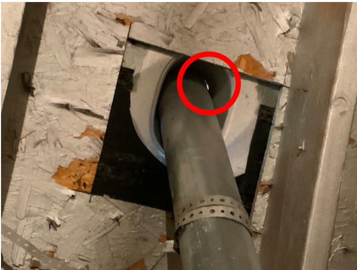
Daylight at water Heater flue pipe.
