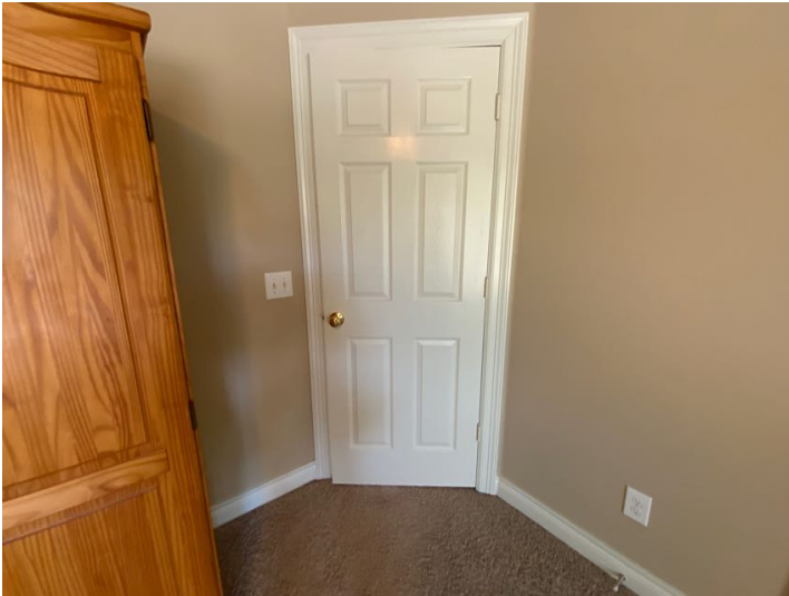
Upstairs front left bedroom door does not latch.
