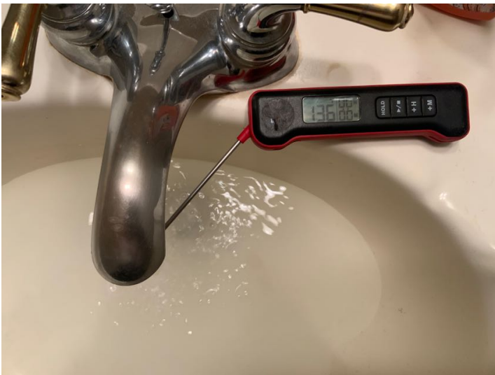
Recommend adjusting to a safe water temperature of 120°.
