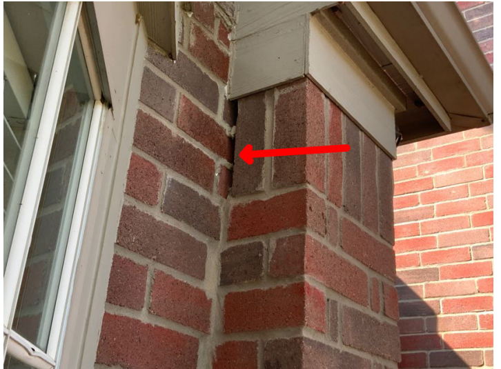
Brick seam seal improvements needed at front of home.
