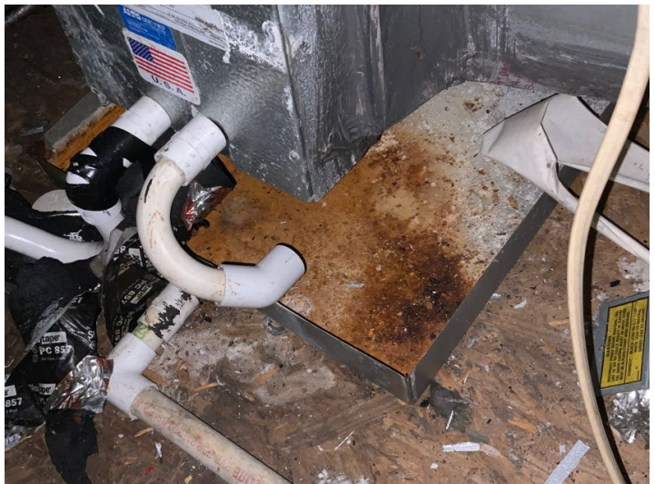
Rust in drip pan under unit 1.
