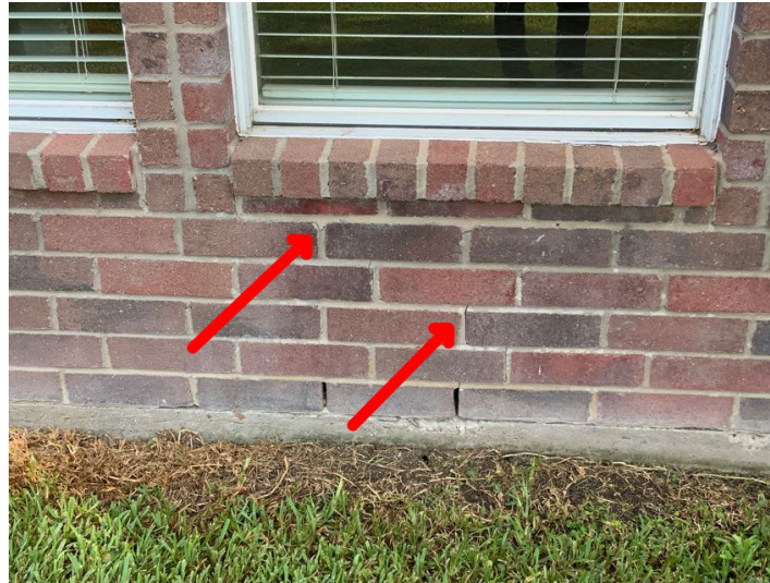
Minor settlement crack at Back of home.
