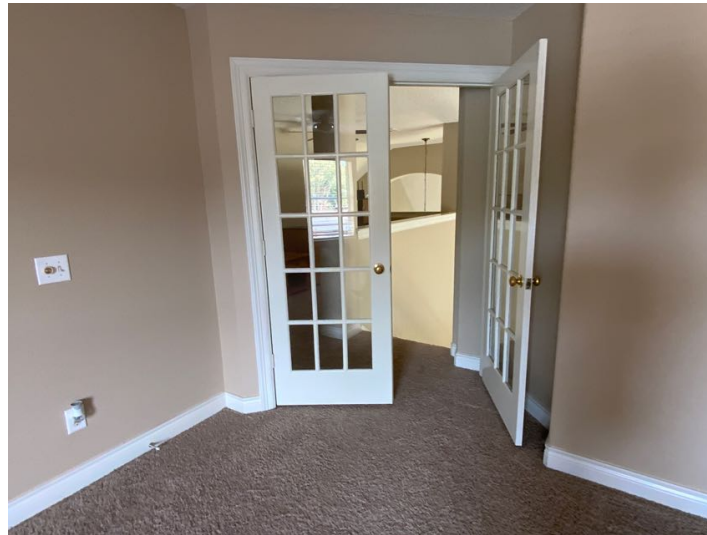
Trim adjustments needed at upstairs media room.
