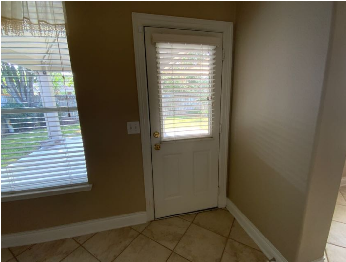
Trim adjustments needed at Back door.
