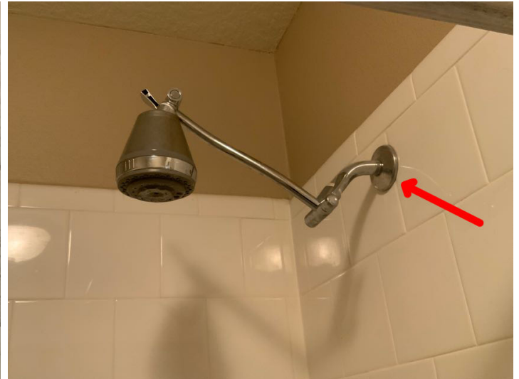
Faucet seal improvements needed at upstairs bathroom bathtub.
