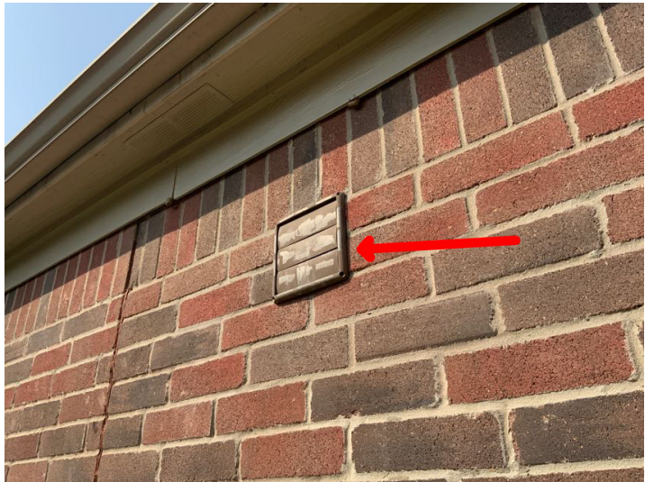
Vent perimeter seal improvements needed at left of home.
