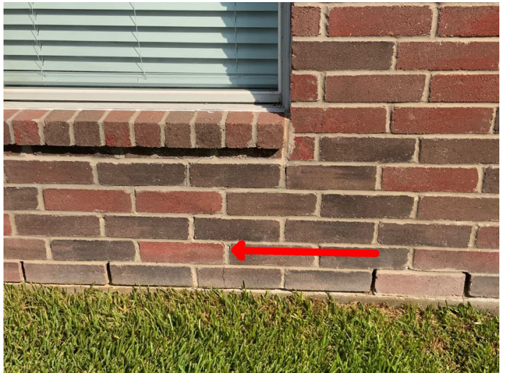
Minor settlement crack at Back of home.
