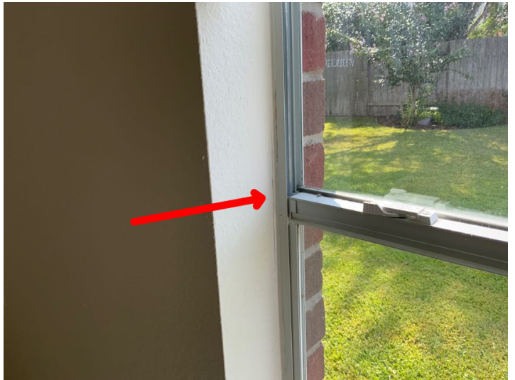
Interior caulking improvements needed throughout home.
