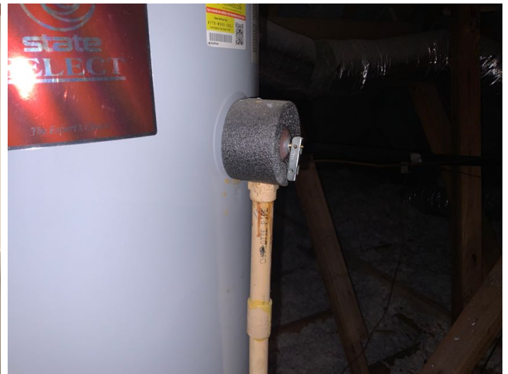
Inoperative TPR valve .
