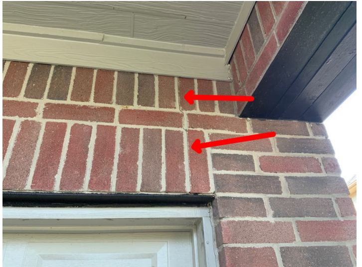
Lintel movement crack at garage.
