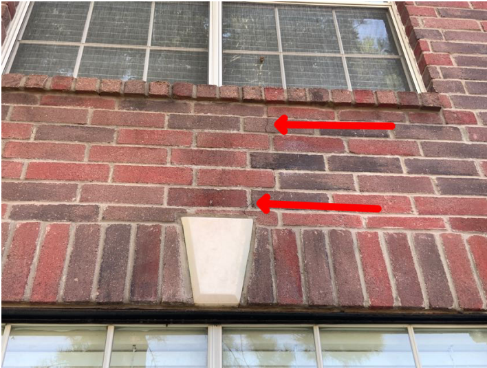
Minor settlement crack at front of home.
