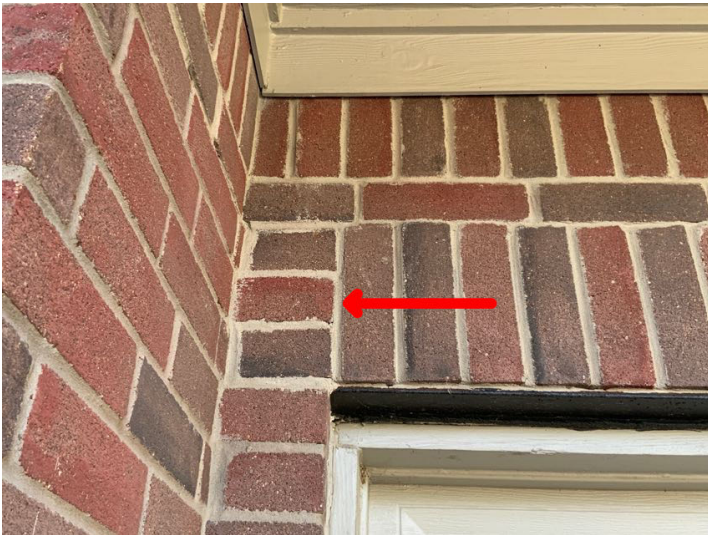
Lintel movement crack at garage.
