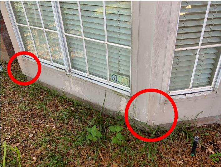
Damaged siding at ground of home.
