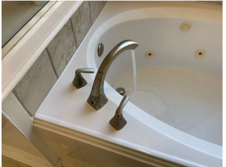
Loose faucet at primary bathroom bathtub.
