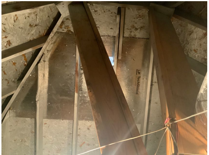
Evidence of prior repairs.
