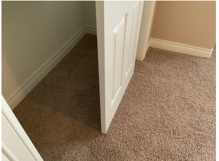
Missing hardware at upstairs front left bedroom closet.
