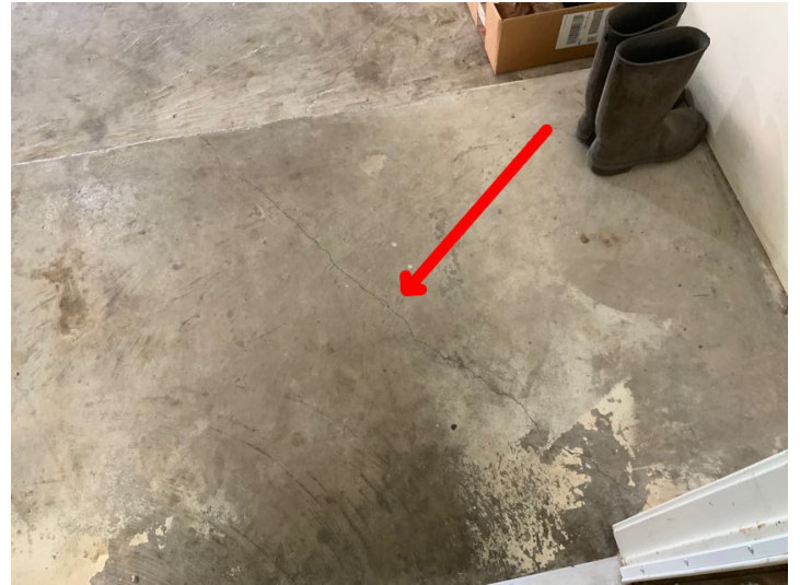
Minor cracks in garage floor.
