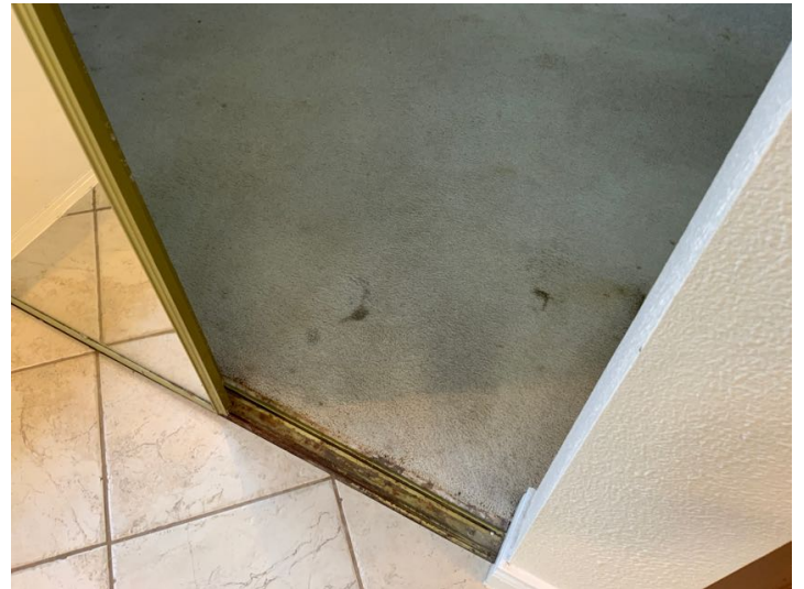
Damaged and stained carpets at primary bedroom closet.
