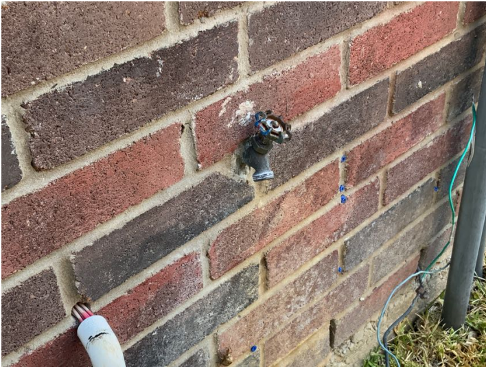
Anti siphon valves are required.
