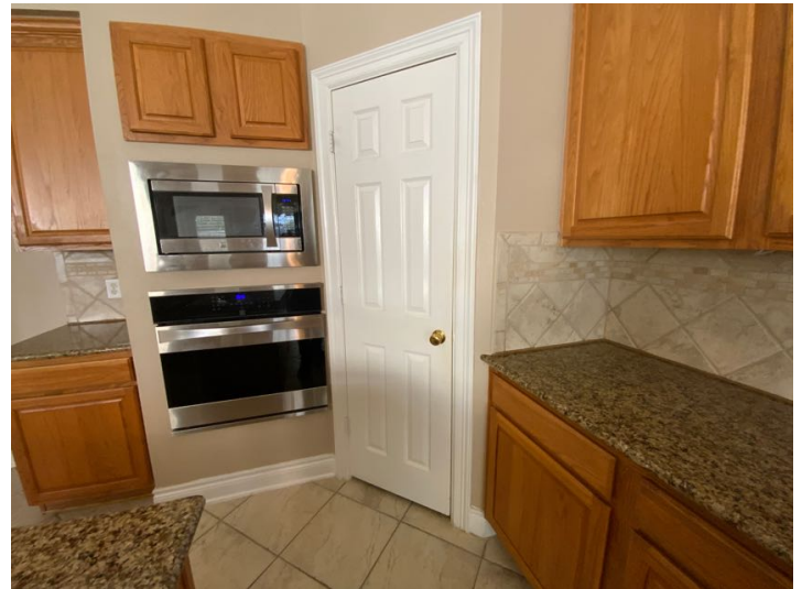
Trim adjustments needed at pantry door.
