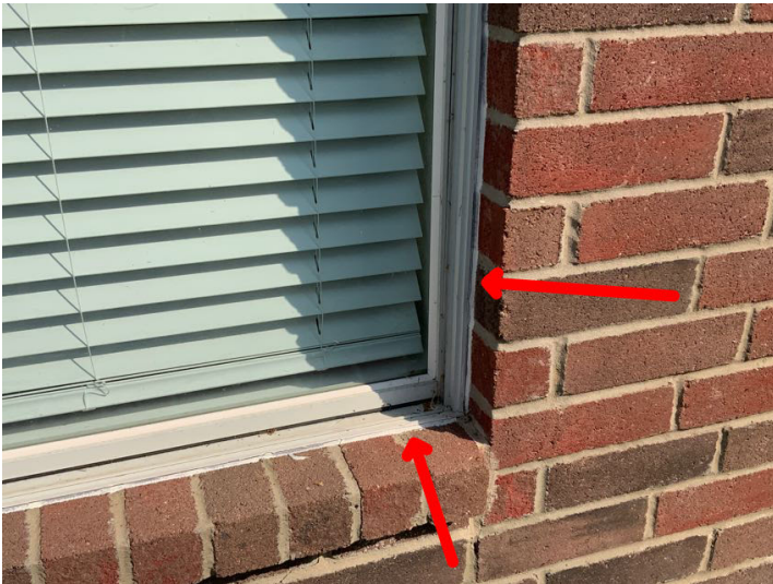
Exterior caulking improvements needed at Back of home.
