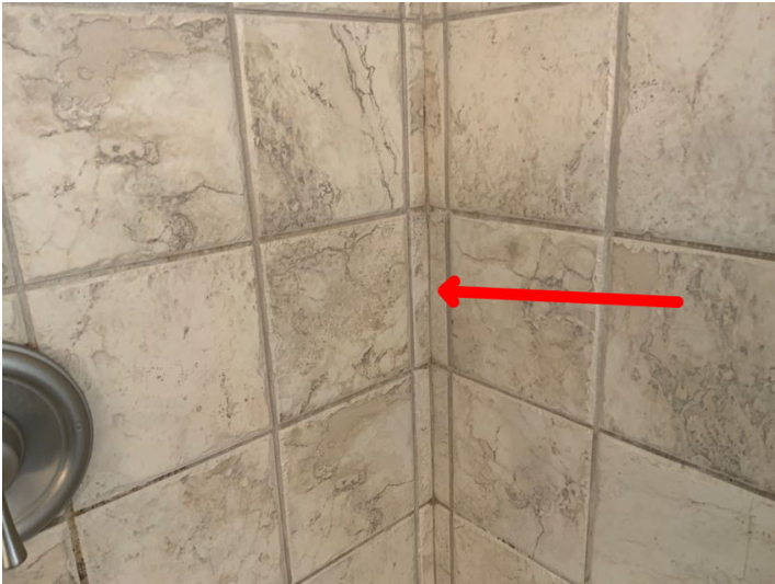
Shower enclosure caulking improvements needed at primary bathroom.
