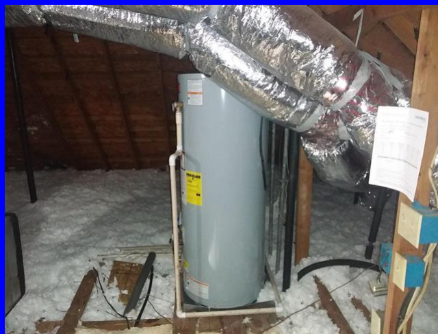
50 gallon water heater in attic
