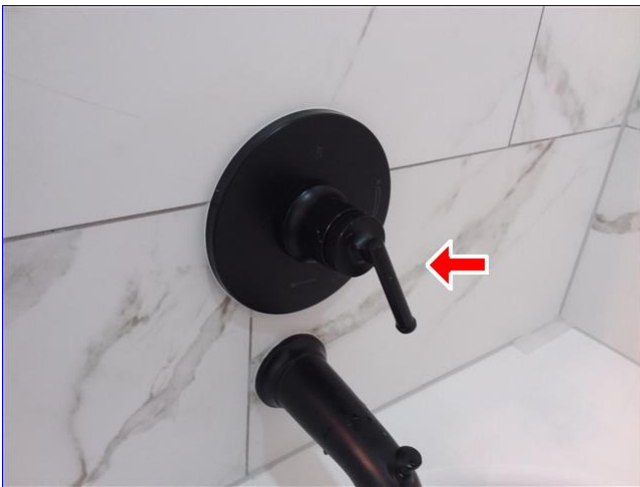
A. Item 5(Picture) all master bathroom handles
