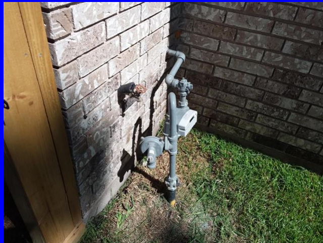
gas meter left side
