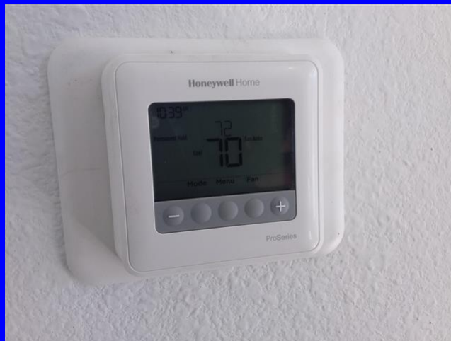
thermostat outside master bedroom
