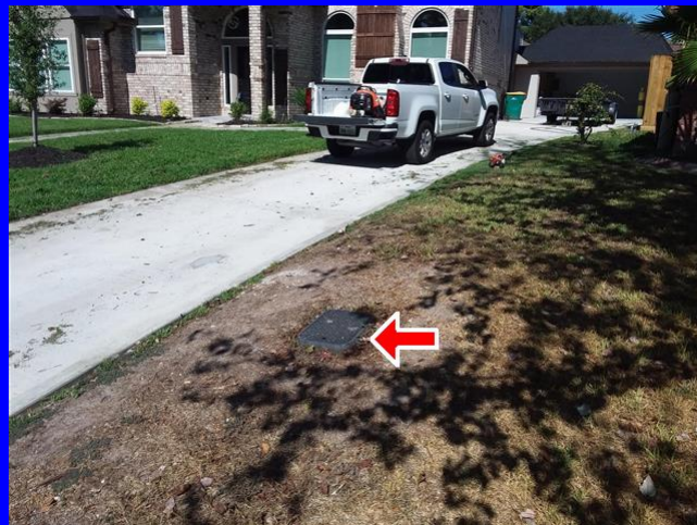
water meter front right
