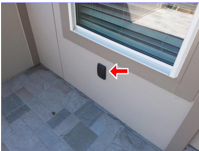
B. Item 3(Picture) upper balcony cannot be opened
