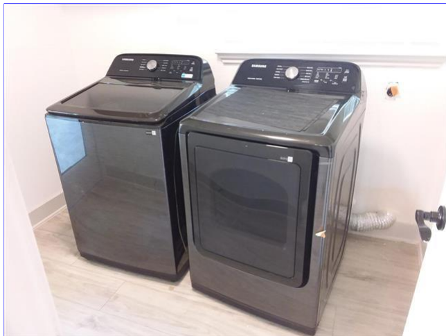
H. Item 1(Picture) washer and dryer installed
