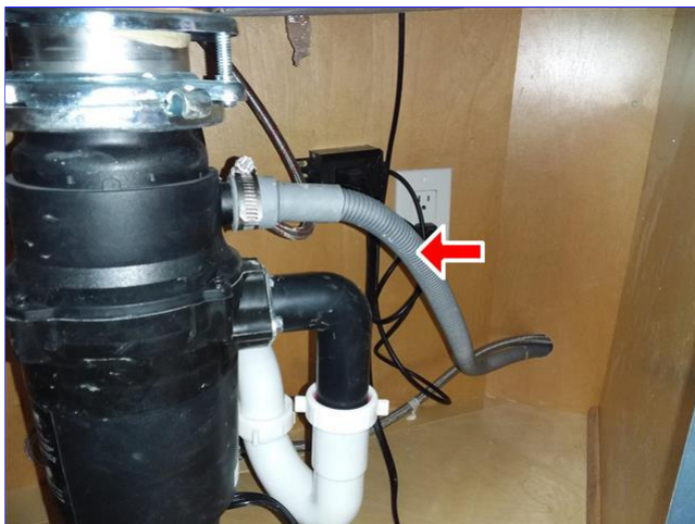
A. Item 2(Picture) missing high loop
