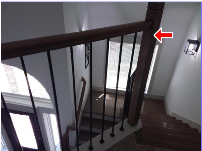
I. Item 1(Picture) loose handrail
