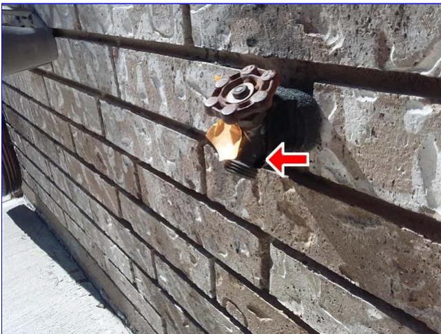
A. Item 3(Picture) missing anti siphon
