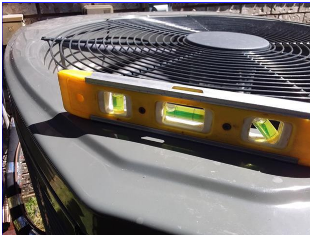
B. Item 3(Picture) unit not level
