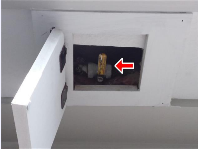
J. Item 3(Picture) incorrect valve installation
