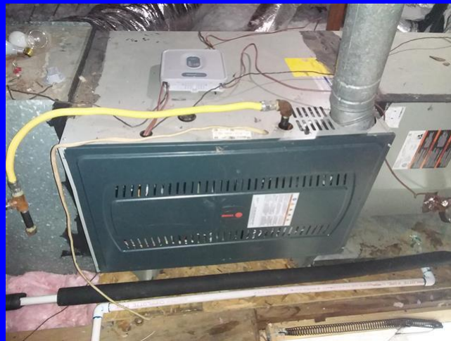
gas furnace upper attic
