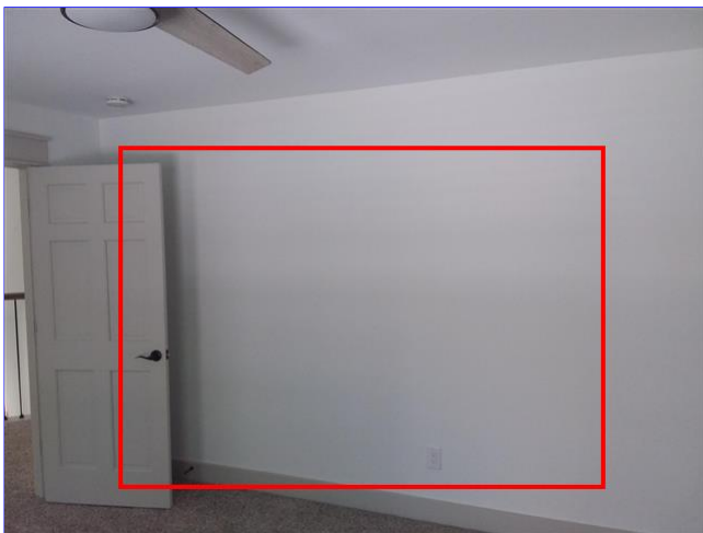
D. Item 4(Picture) left upstairs bedroom wall
