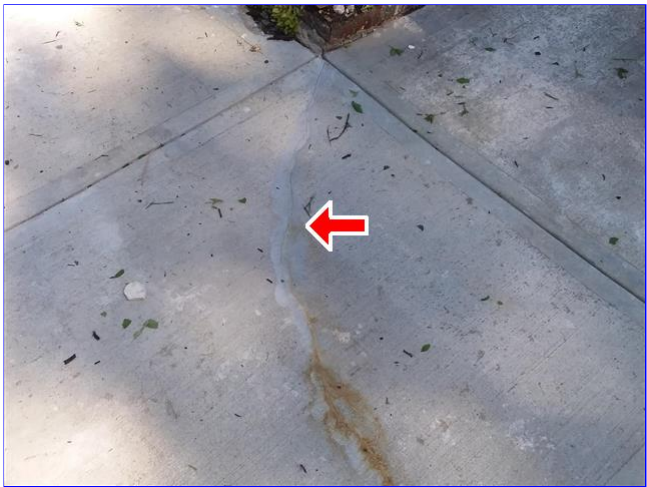
L. Item 3(Picture) walkway crack
