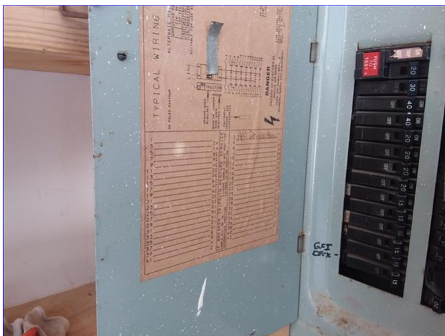
A. Item 1(Picture) missing labels
