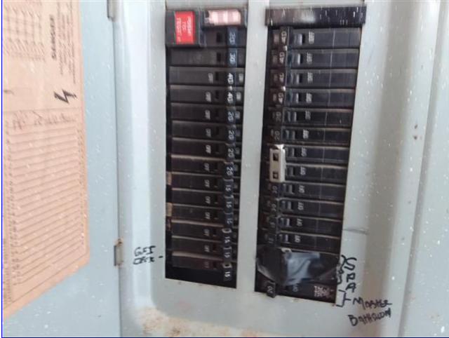
B. Item 1(Picture) missing AFCI breakers
