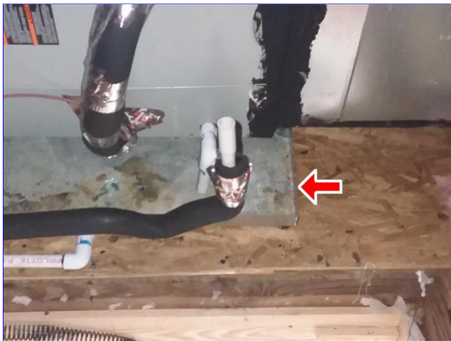
B. Item 4(Picture) missing pan switch
