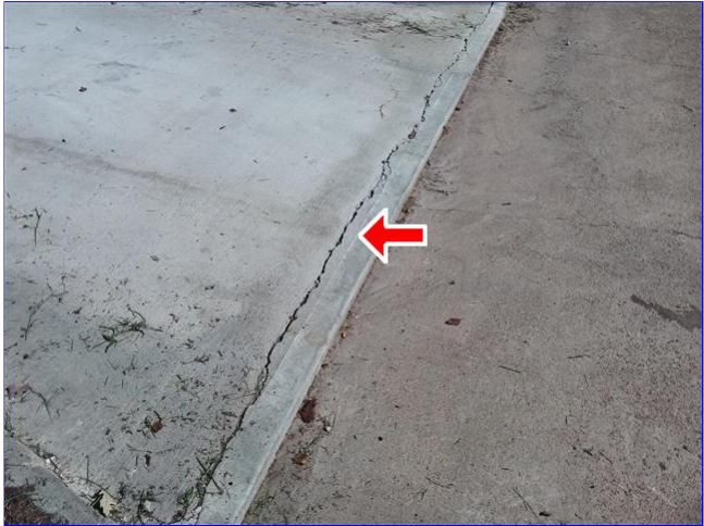
L. Item 2(Picture) driveway cracks
