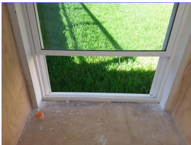
H. Item 1(Picture) missing screens in areas
