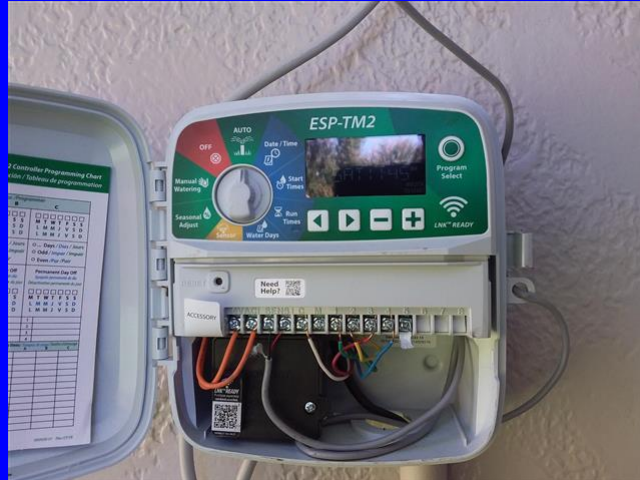
sprinkler system control panel garage exterior 4 wired zones
