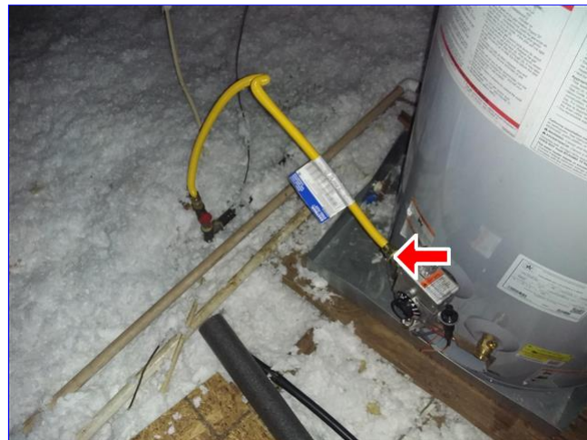
C. Item 2(Picture) missing drip leg
