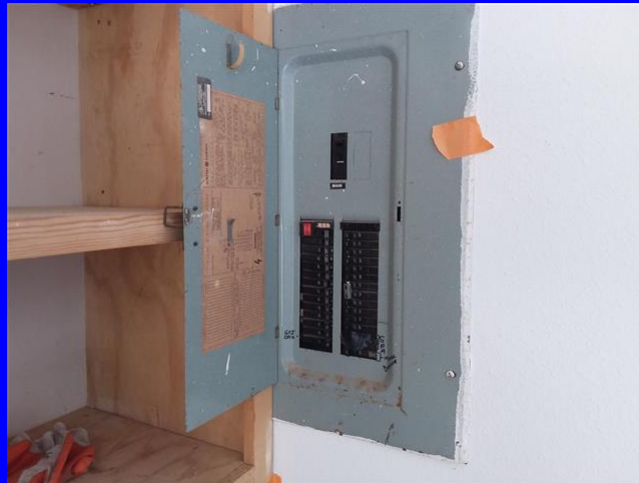
150 amp panel in garage
