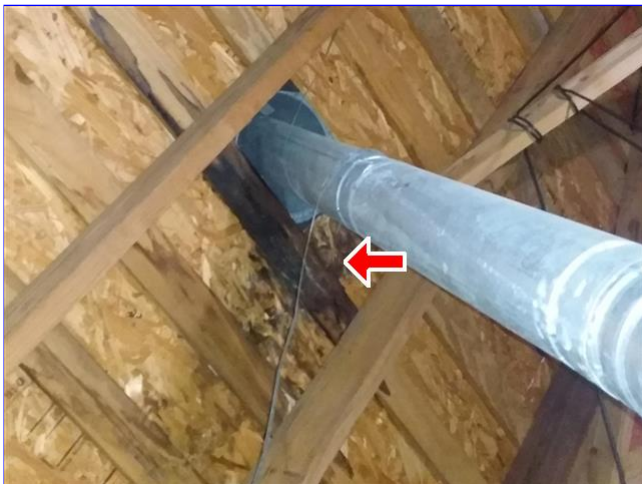
D. Item 11(Picture) furnace exhaust
