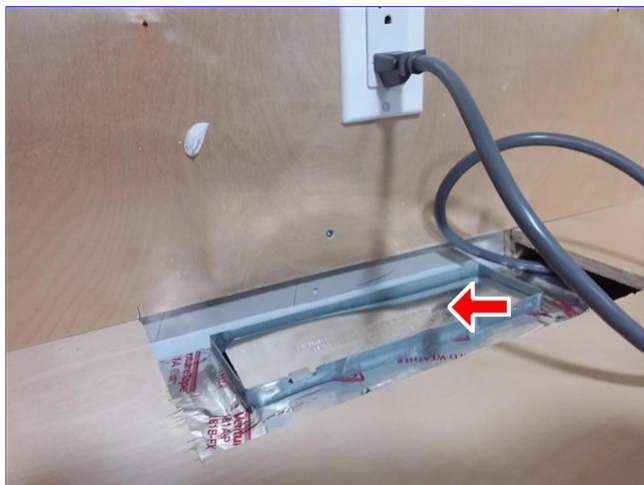
C. Item 1(Picture) vents into cabinet
