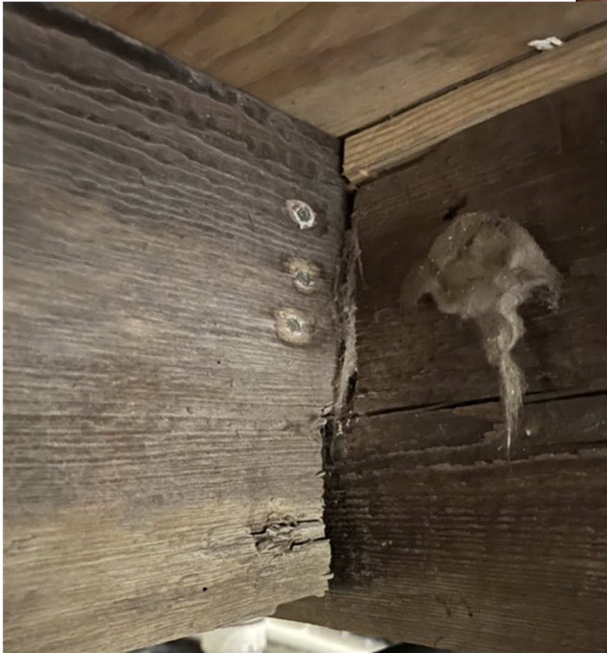
Figure 11: The original joists re notched, however since the joists are true 2"x8" construction, they appear to hold up to the stress without splitting.
