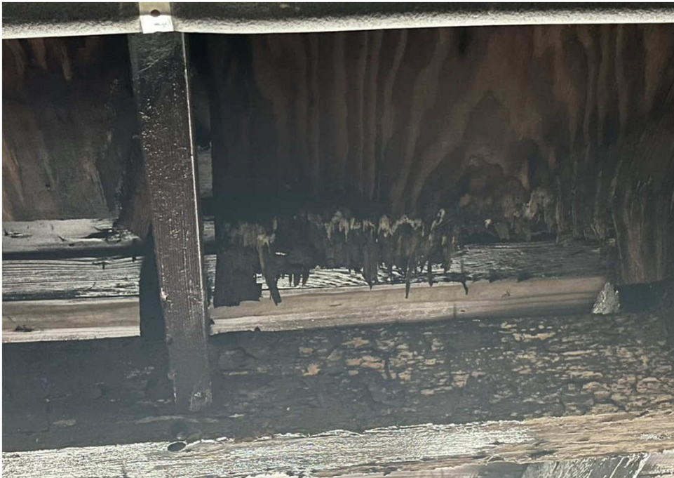
Figure 8&9: Replace rotten decking and joists below front entry room
